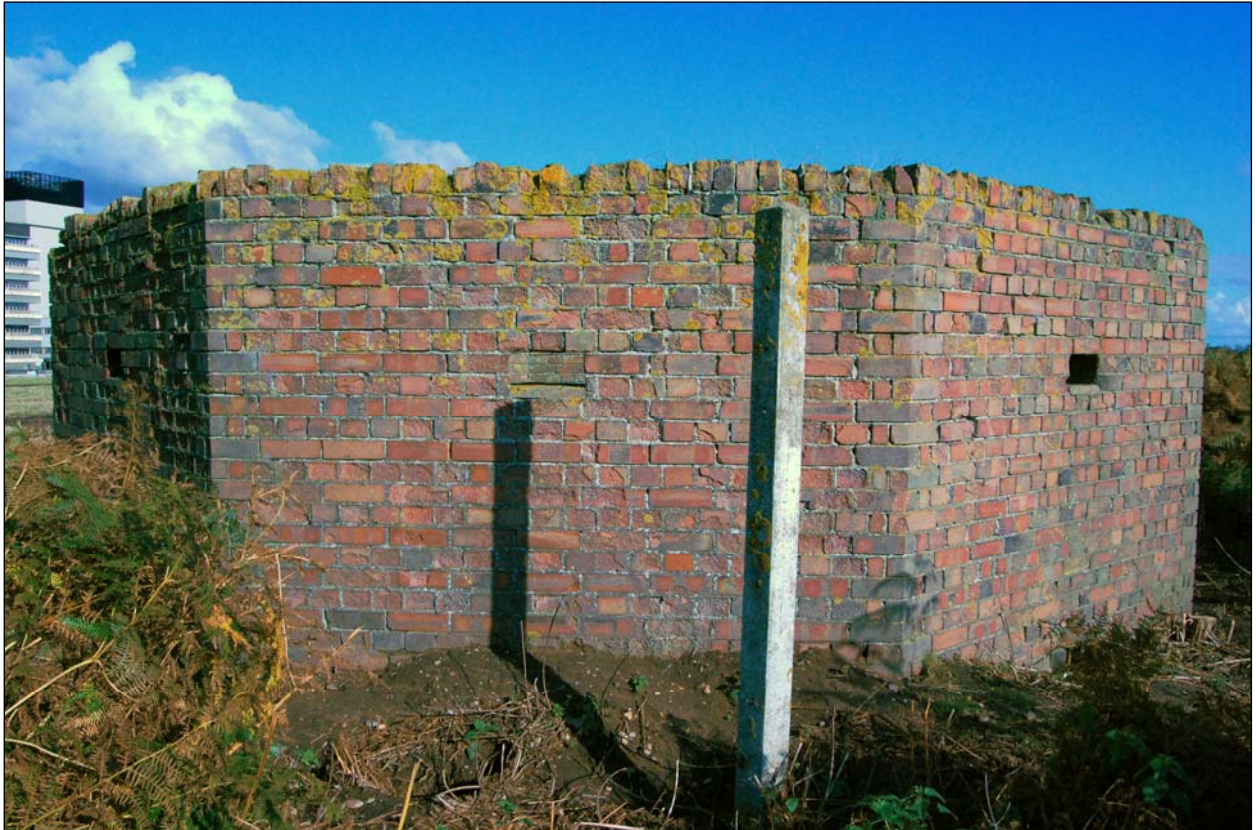
Plate 9. HFDF curtain wall, typical elevation with loophole, facing north-east (photo edited to compensate for low light conditions)
