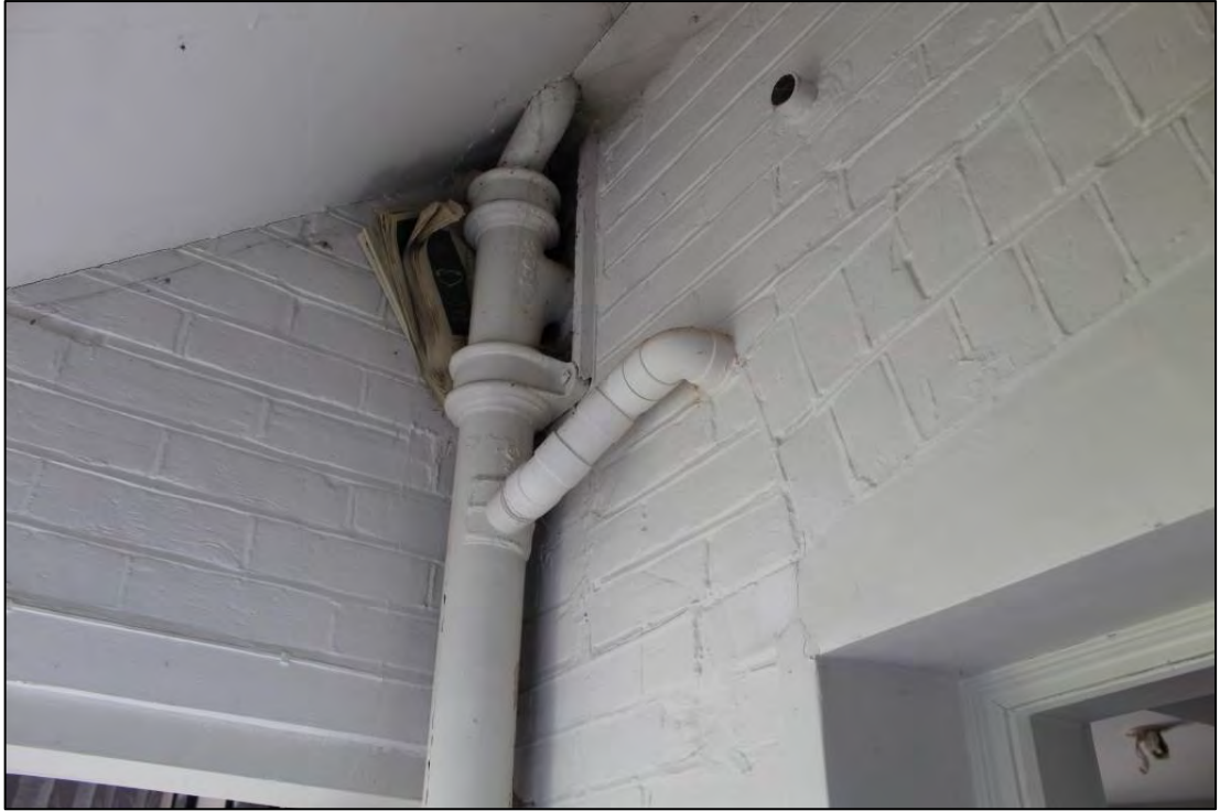
Photo 16: Exposed soil pipe in Room 2
