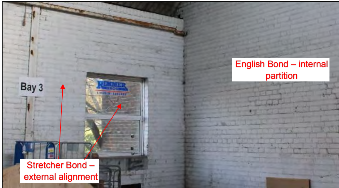
Photo 50: Detail of contrasting brick bonds between internal partition and external elevation, Room C13 looking north-east
