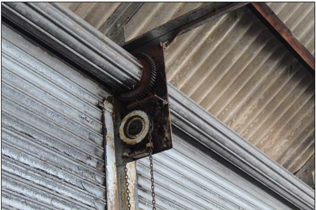
Photo 54: Chain pulley system in Room C14
