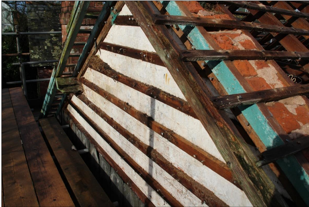
Fig.25 Southern gable end showing brick wall with battens for hanging slate tiles (removed)
