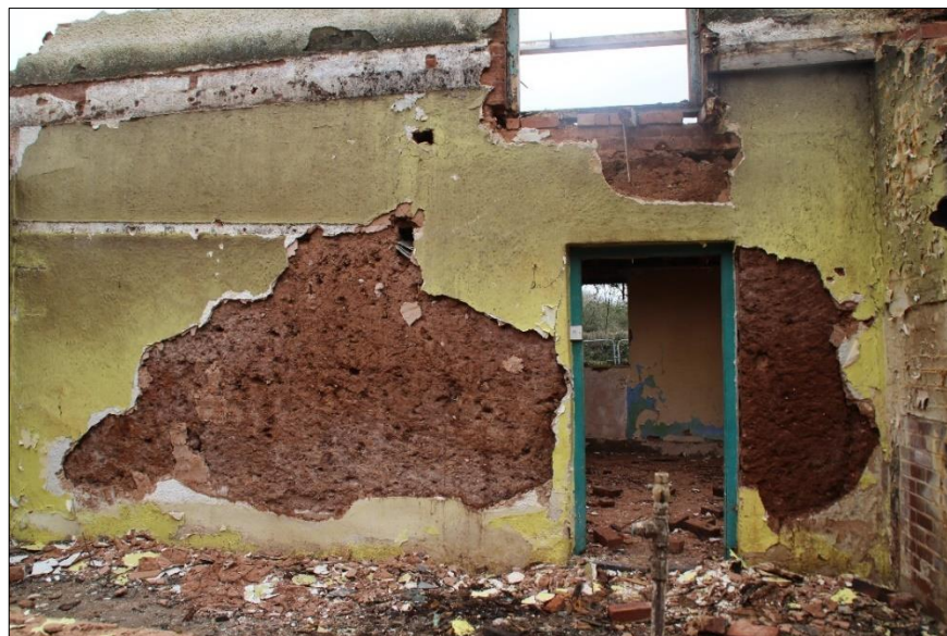
Fig.54 View of the western wall of the building within the former kitchen extension
