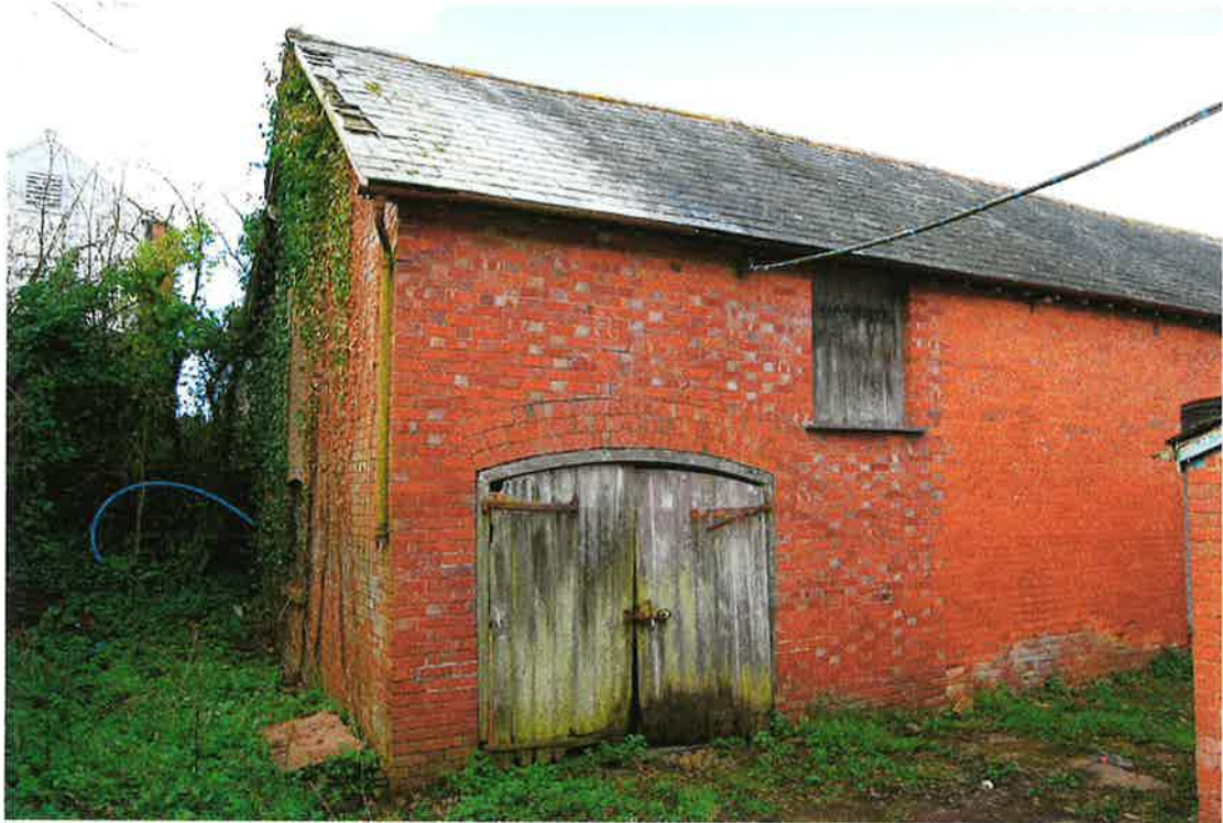
Pl.28: The Cart Shed from the south-east; note the vertical break between it and the adjacent Barn (Building B) to the right.
