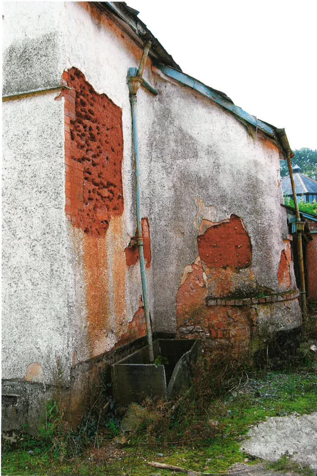
Pl.5: The rear, or west, elevation of the northern portion of the farmhouse, showing the semi-circular projection and the condition of the cob.
