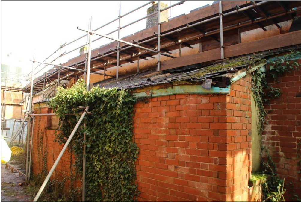
Fig.13 View of the kitchen extension on the western elevation, view taken looking north-east
