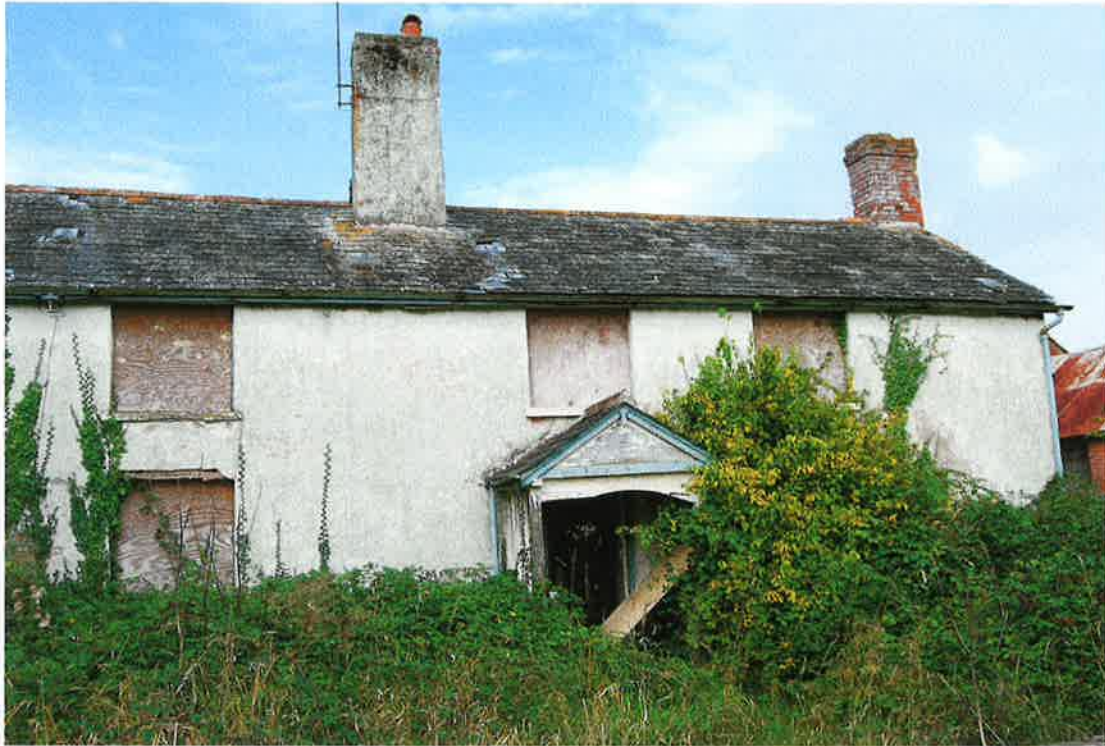
Pl.3: The northern end of the east elevation of the farmhouse; the porch protects the main entrance into the property, which is within the shorter northern section.
