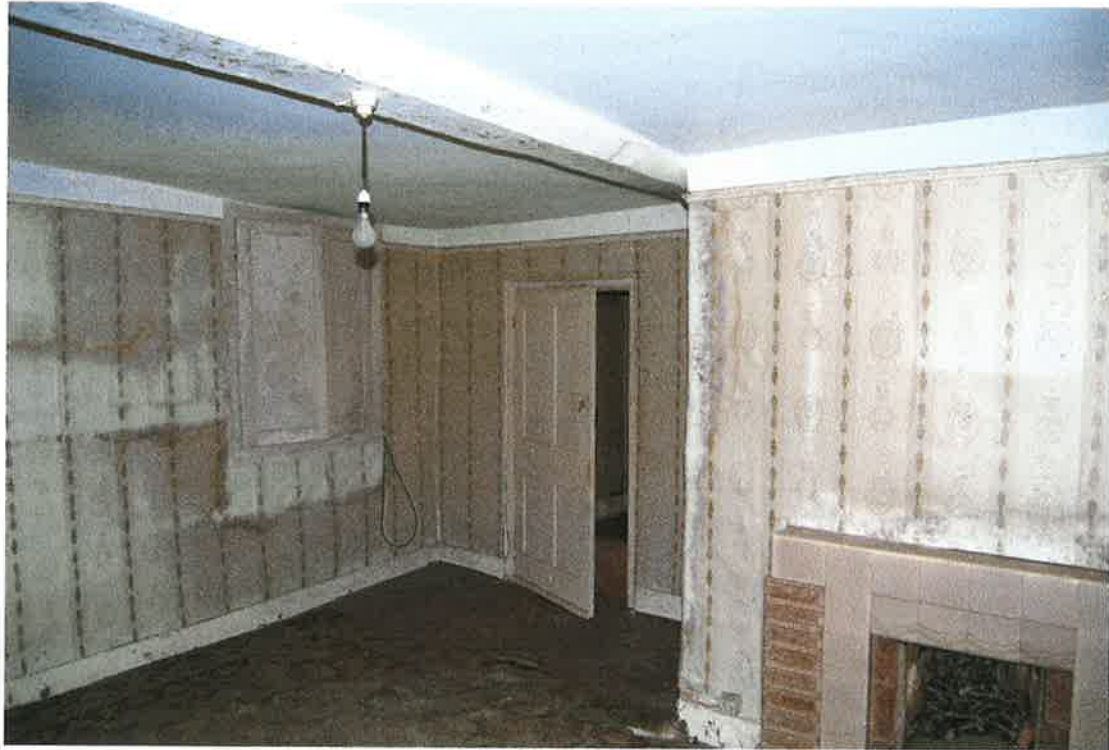
Pl.16: The living room, looking north; the mid-20 th century fireplace is in the large stack to the right and the cupboard on the left could be the site of an original window.
