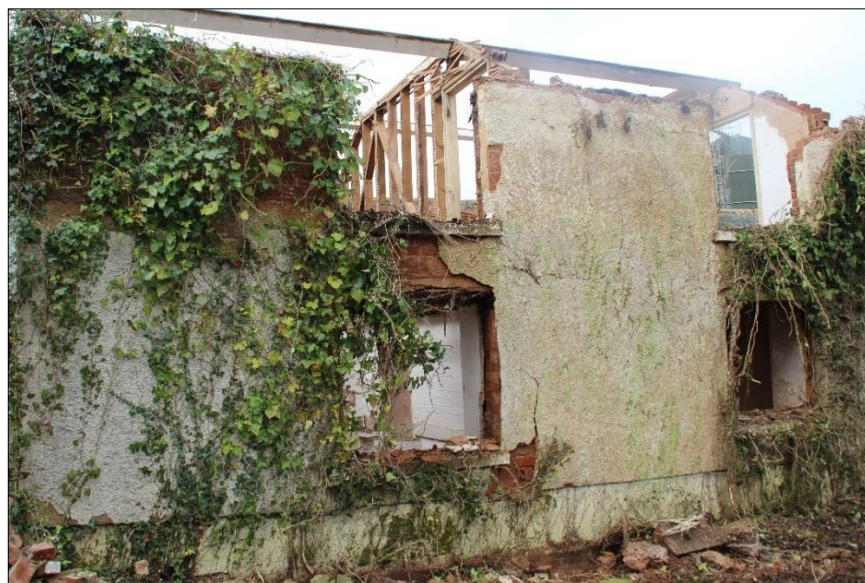
Fig.49 View of the southern part of the building, eastern elevation, looking west
