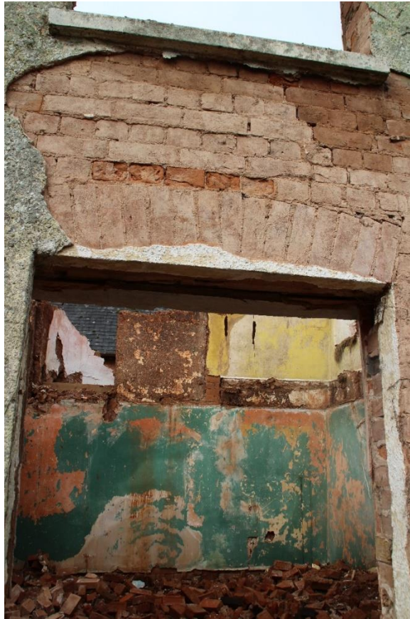
Fig.40 Detail of shallow segmental arches over doors and windows on eastern elevation
