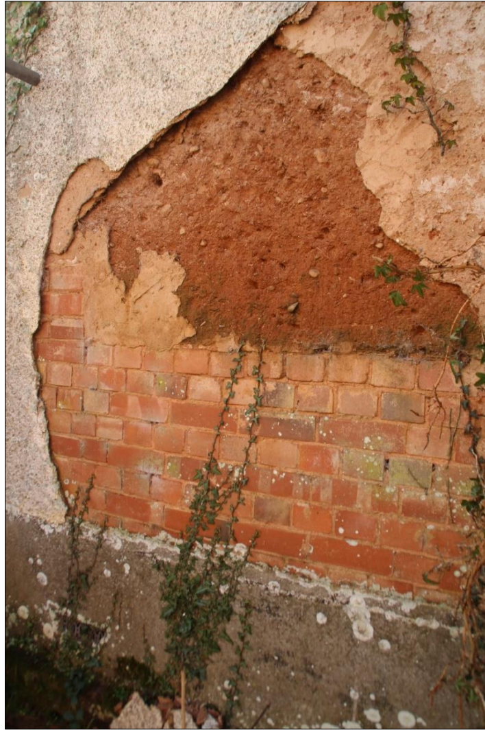
Fig.10 detail of north gable wall showing brick and cob with render layers
