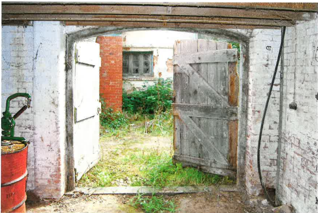
Pl.29: The inside of the double doorway in the east wall of the Cart Shed.
