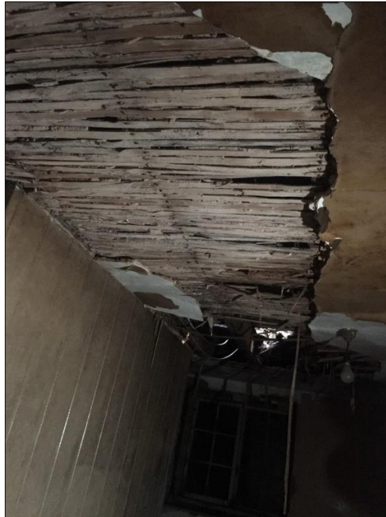
Fig.28 The rear hallway with lathes in the ceiling
