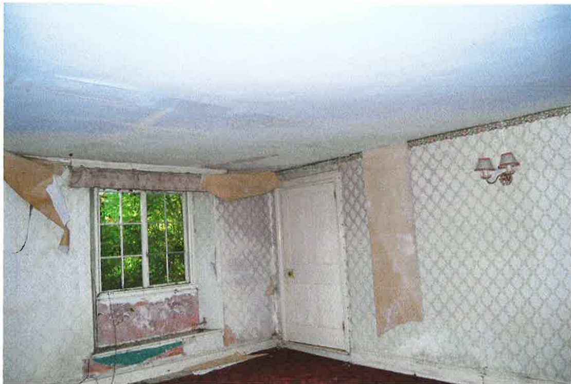
Pl.9: The northern, or sitting, ground-floor room, looking south-east; note the two-light casement and the four panelled door – standard patterns throughout the building.
