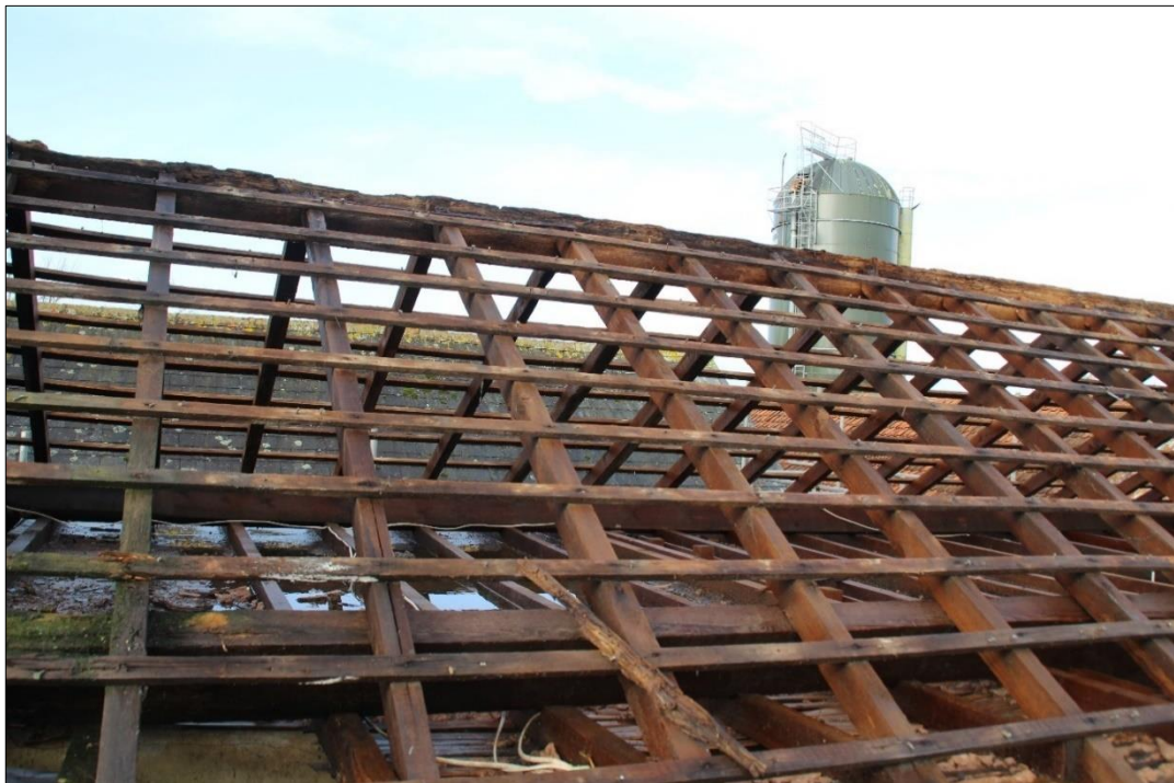
Fig.19 View of the eastern roofscape, looking internally within purlin resting on rafters
