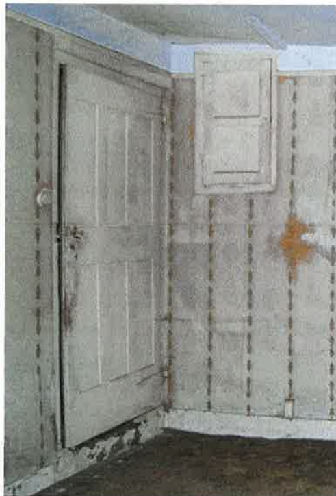
Pl.17: The south door of the living room and the small 'spice cupboard' type feature in the north wall next to it.
