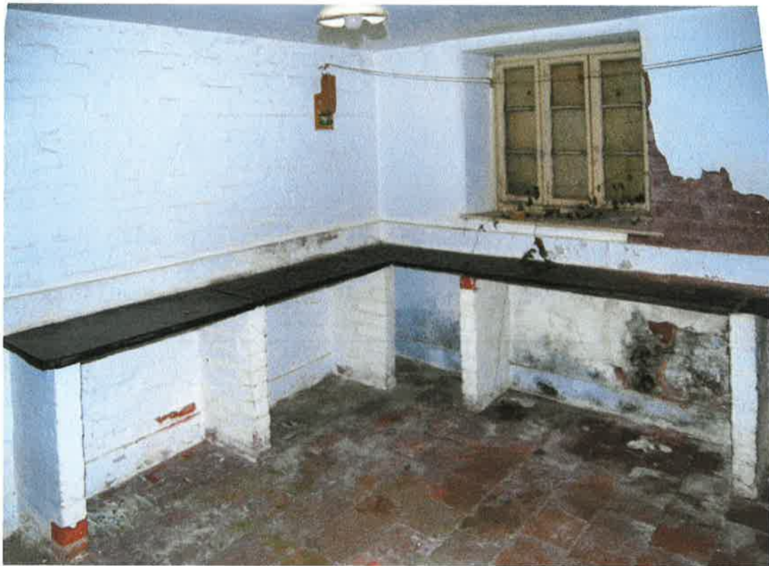
Pl.18: The slate shelves on brick piers in the presumed dairy at the south end of the farmhouse. Note the three-light window in the rear wall and the quarry tile floor.
