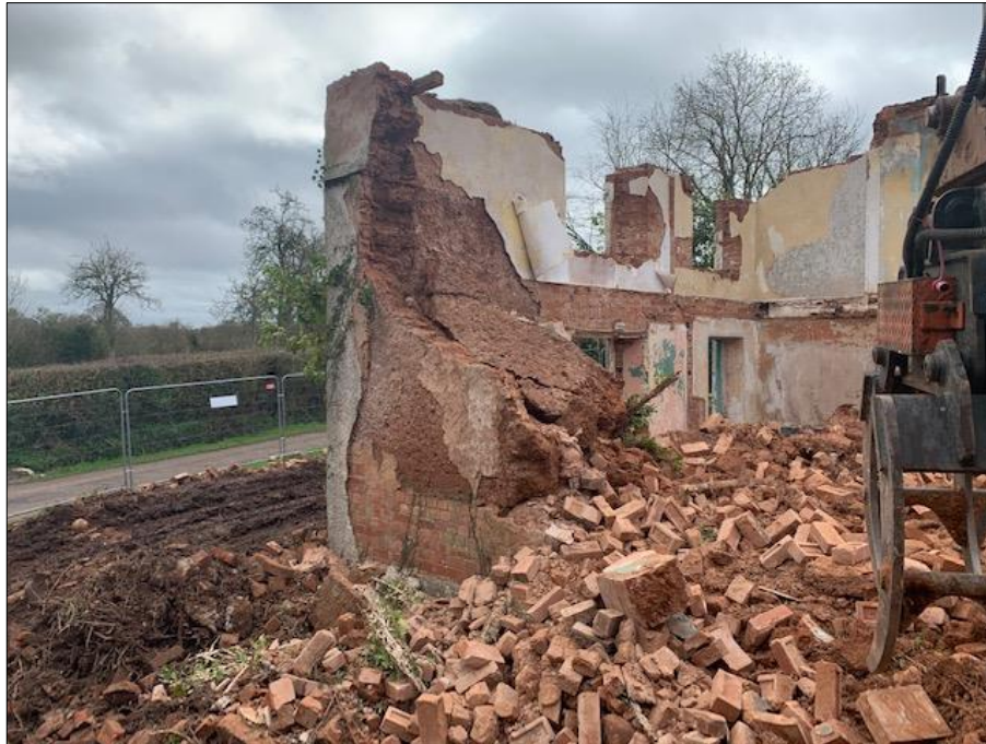
Fig.57 View of the northern elevation as its collapses showing cob
