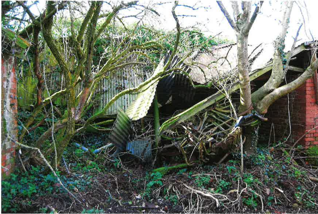
Pl.34: One of the collapsed shelters at the western end of the farmyard.
