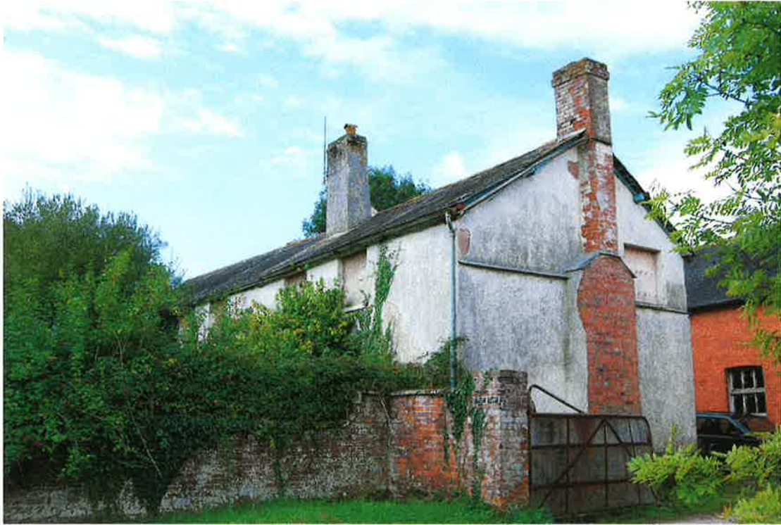
Pl.6: The farmhouse from the north-east, showing the north gable and the rebuilt chimney stack.
