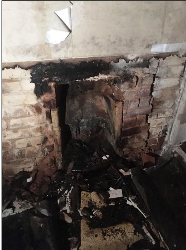
Fig.32 Brick fireplace in living room
