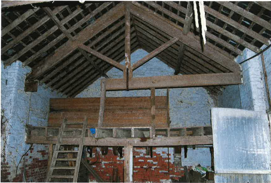
Pl.25: The inside of the Barn Range, looking north; note the cut tie-beam of the truss, the inserted gallery, and beneath, the line of belt shafting against the cross-wall.
