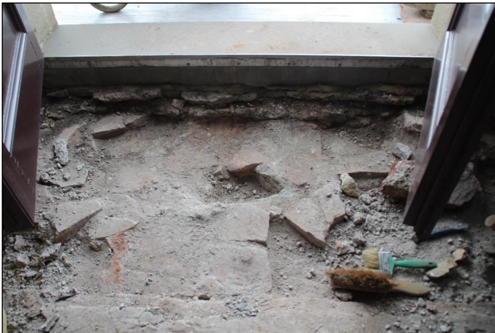
Photo 15 Detail of the floor and outer wall substructure with Pennant stone by the garden entrance
