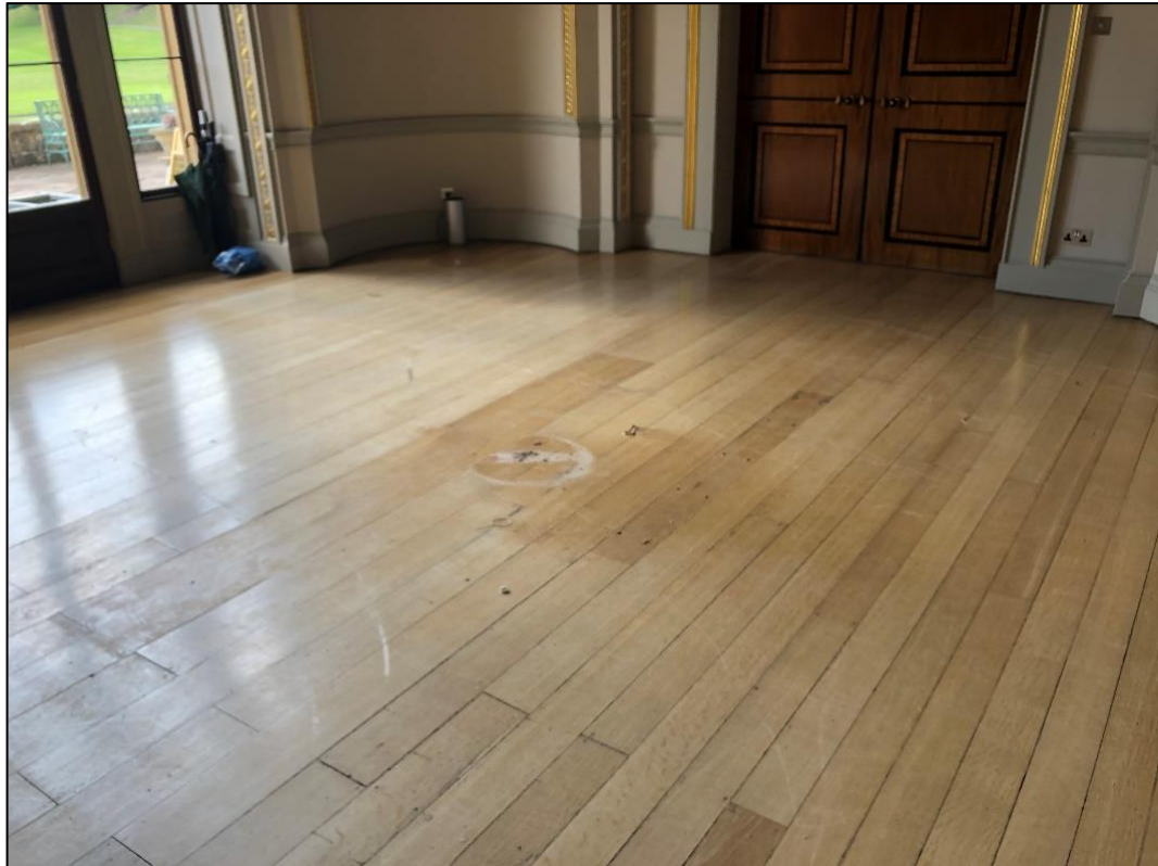
Fig.5 Image of the room looking south-west towards the library doors and garden terrace
