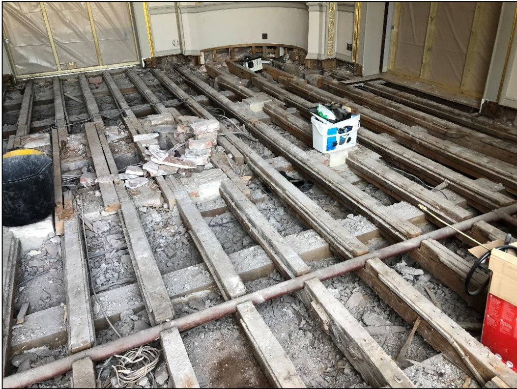
Photo 9 View of the central eastern area of the room including the stove void
