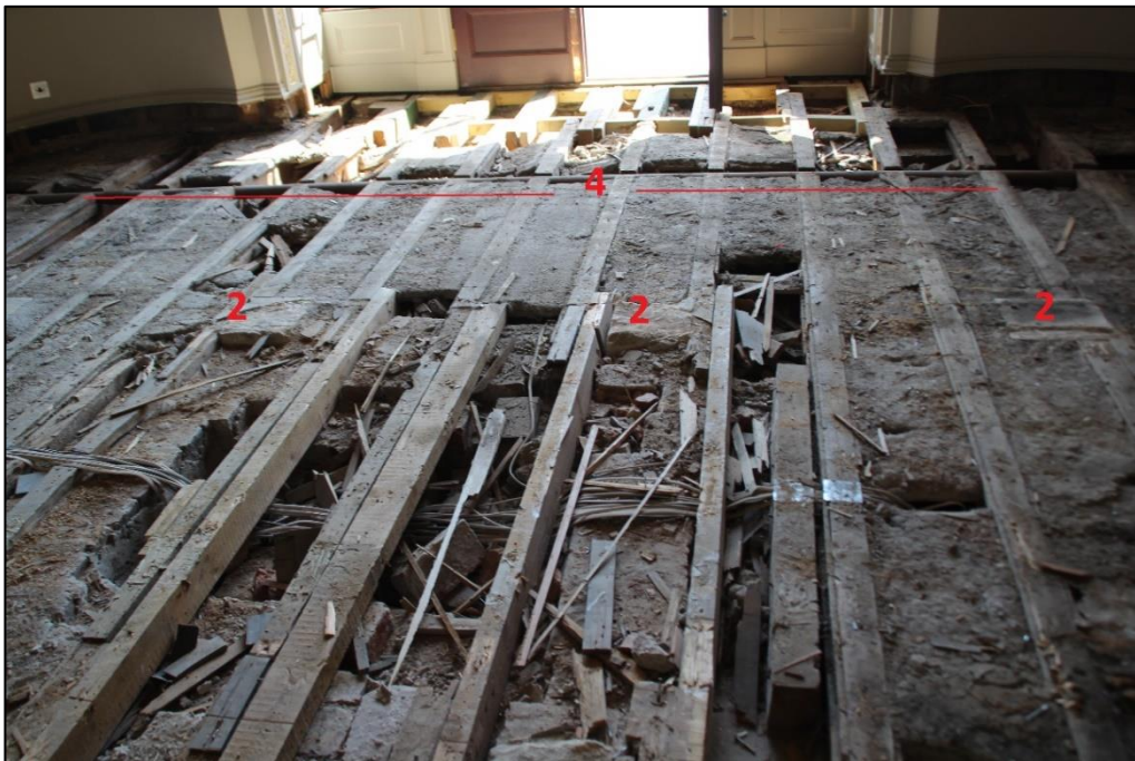
Photo 6 View of the central south portion of the room overlooking the garden terrace
