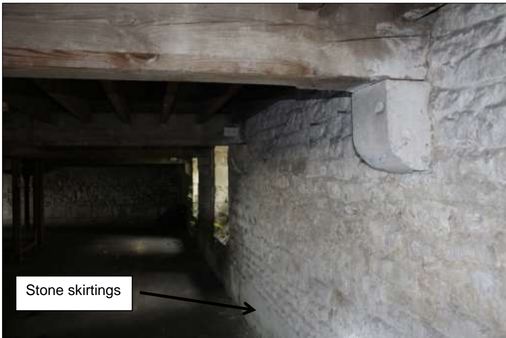
Fig.19 Main span beams resting on stone corbels, lower growing floor of Maltings 1
