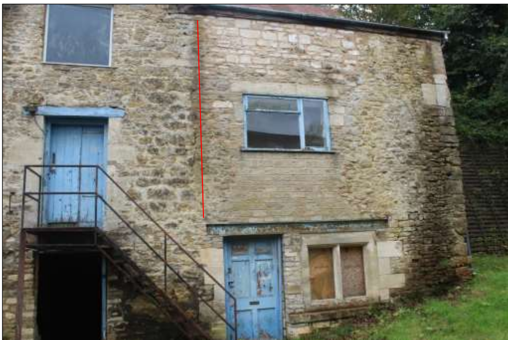
Fig.63 View of western north-facing elevation of Maltings 2, the kiln, showing building join in red
