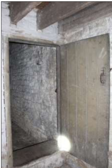
Fig.21 Timber door and step from lower growing floor to kiln area, Maltings 1
