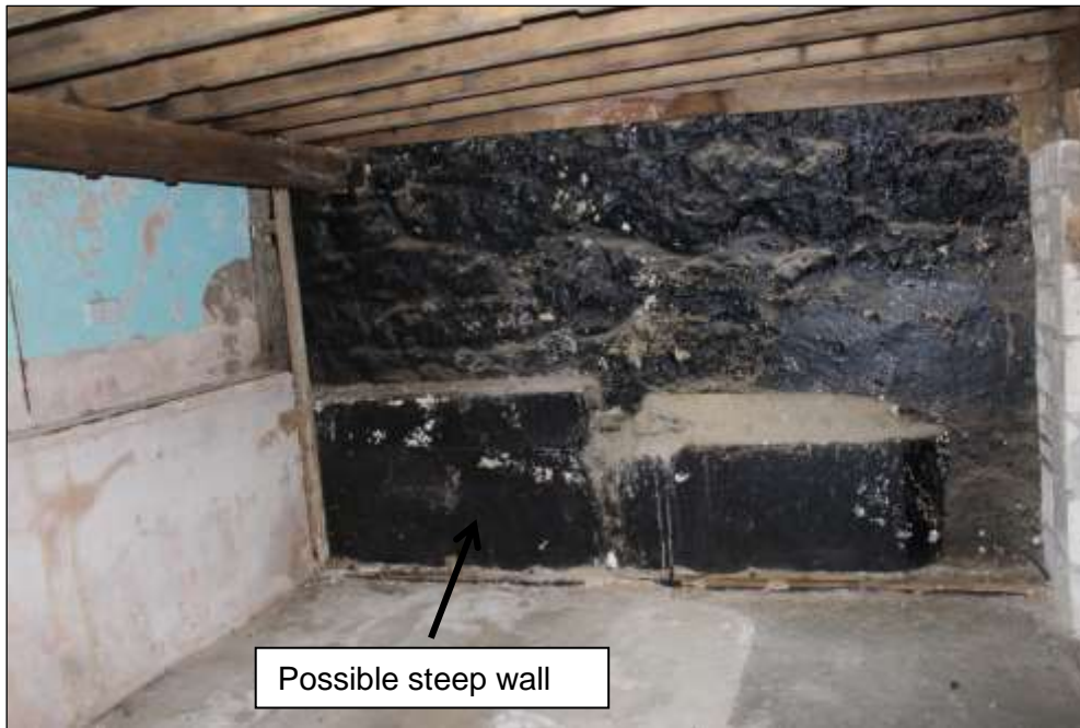
Fig.71 Area which may have formerly been a steep in Maltings 2 lower ground floor
