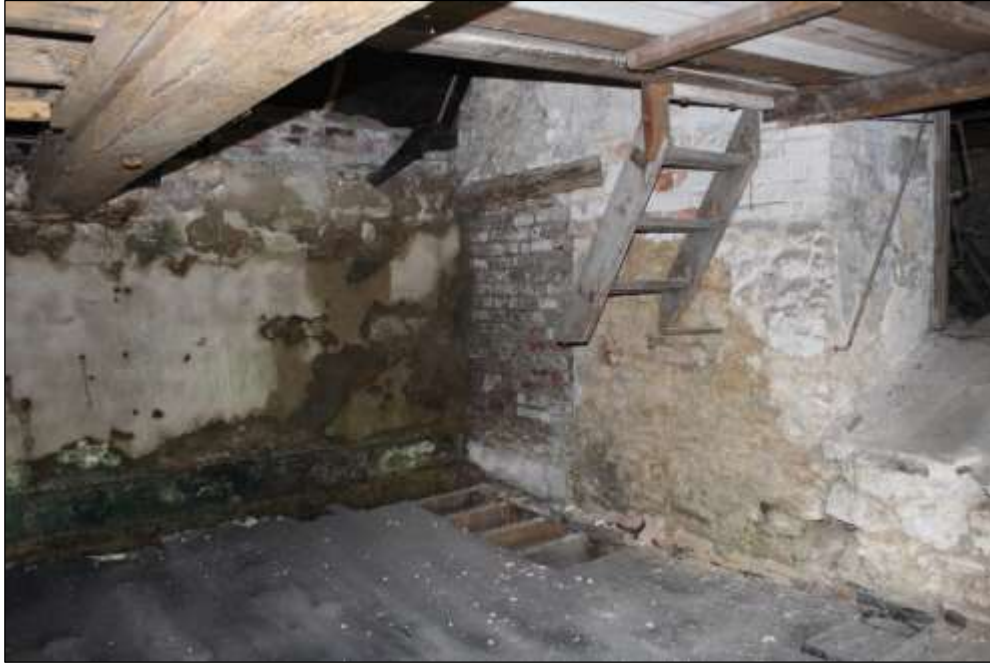
Fig.78 Truncated stairway to upper floor and filled in doorway, possibly predating the kiln
