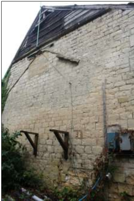
Fig.12 View towards the west elevation of Maltings 1 showing scar of attached building and other accretions
