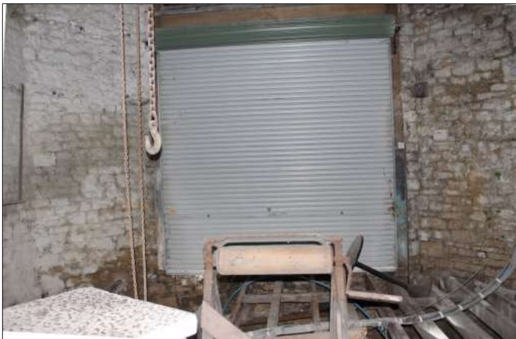
Fig.47 Kiln chamber, showing modern inserted garage doors, half the floor surface is missing
