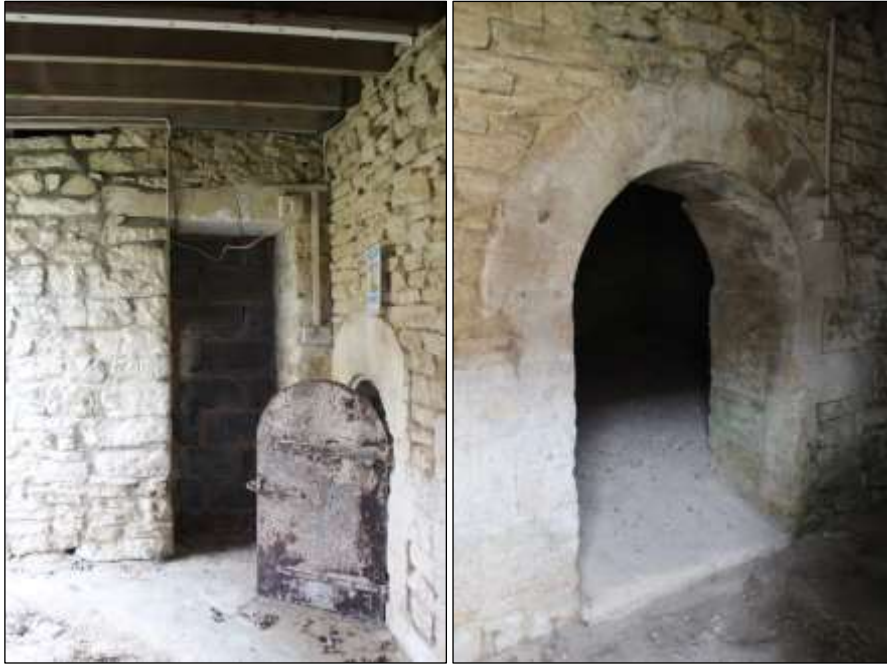
Fig.84 details of openings to the kiln to Maltings 2, doorway from the north elevation providing light from the left (note blocked doorway)
