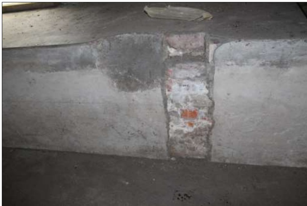
Fig.28 View of middle hacked wall of steep (the steep divider), showing concrete lining
