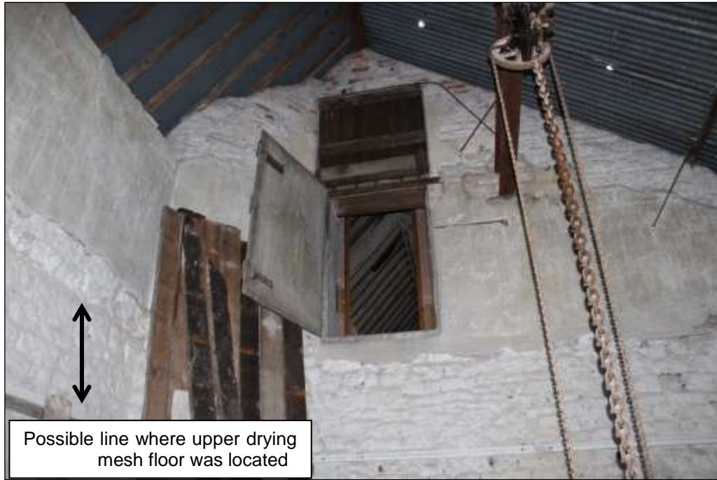
Fig.48 View up to kiln roof area showing altered areas of walling, and doorway into upper drying floor (attic space)
