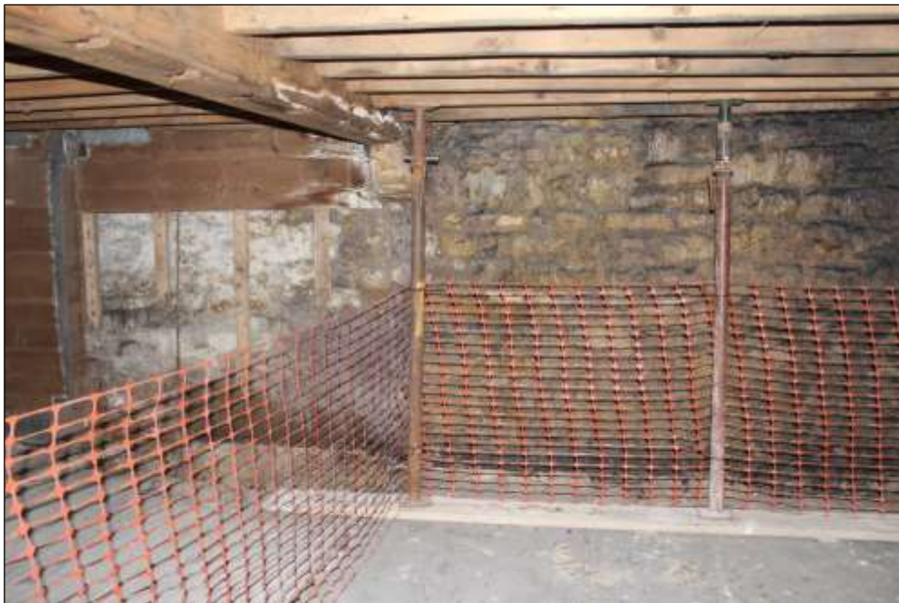
Fig.73 View of upper growing floor, south wall with some timber boarding removed
