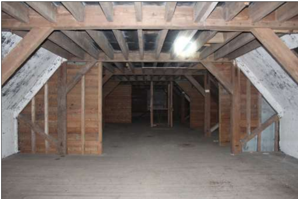
Fig.37 View of lower storage floor (first floor) of Maltings 1, view to the west
