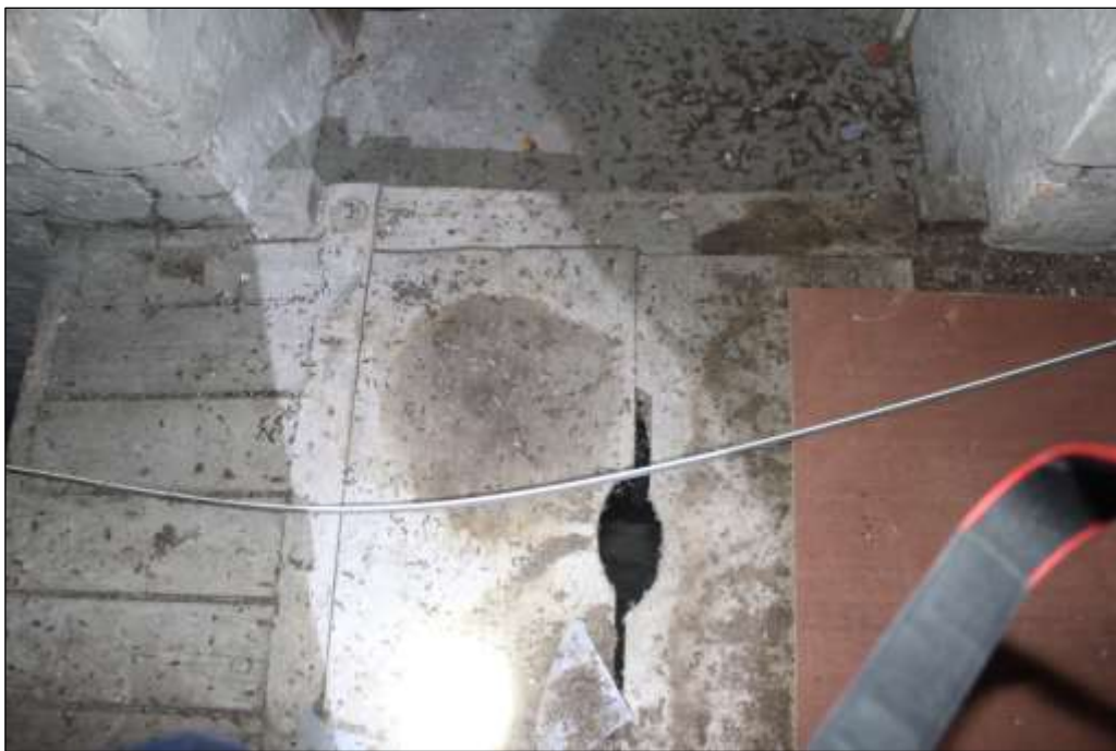
Fig.45 Hatch to lower drying floor with grab holes located by the doorway to the kiln in the attic
