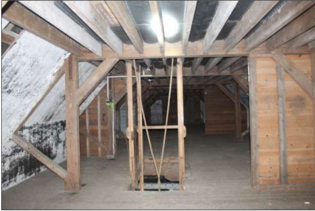
Fig.38 View of hoist and lower storage floor of Maltings 1, view to the east
