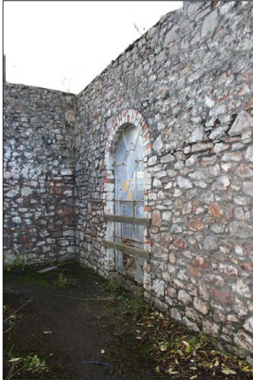
Photograph 27 Sample shot of the internal view of Building B with the rough-cut stone work
