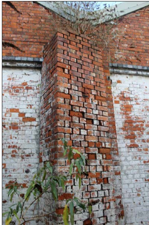
Photograph 13 Sample view of the irregular buttress located in the centre of the west recess and between the west and central
