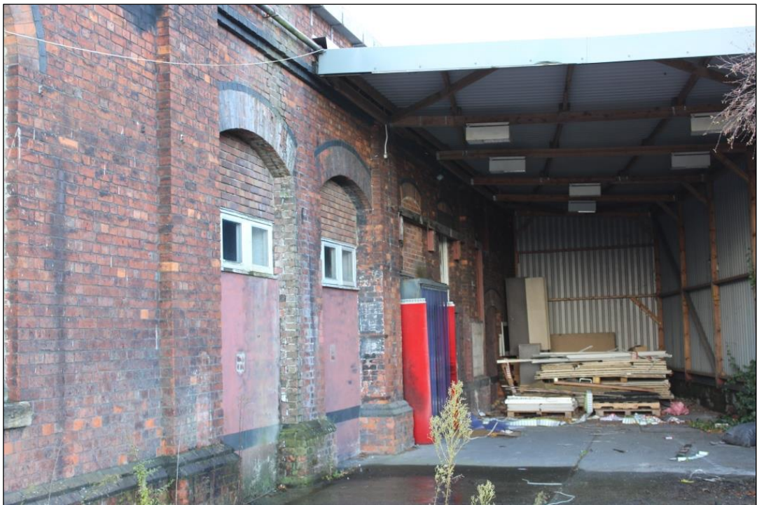
Photograph 16 Sample shot of the features continued under the canopy on the west elevation
