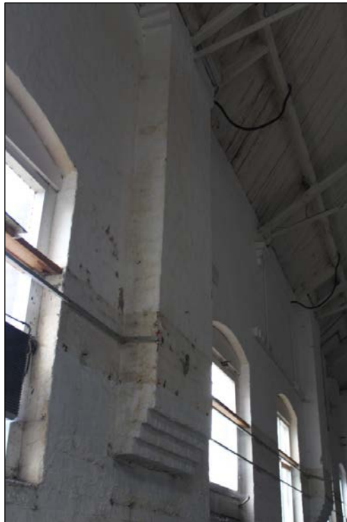
Photograph 24 Detailed view of the stepped base on the pilaster between each window in room 5
