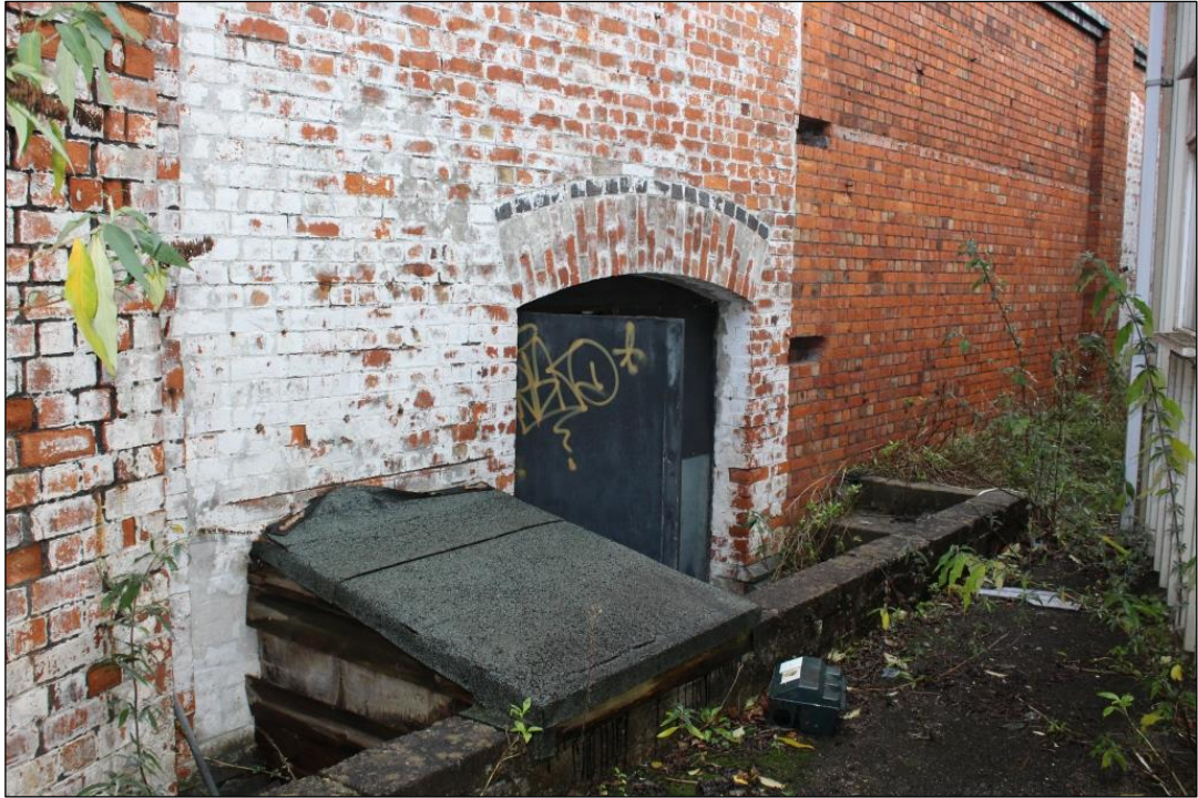
Photograph 12 Central recess with the door and steps leading to the exterior of the building
