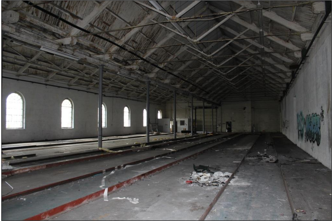
Photograph 18 General view of room 1 looking to the north-west with the row of pillars and bricked in north wall and pedestrian door
