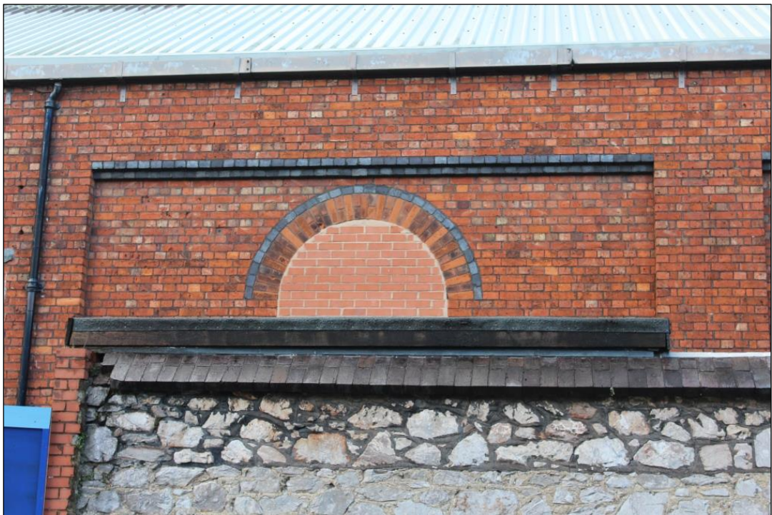
Photograph 8 Bricked in arched window in the eleventh recess from the north with a porch beneath
