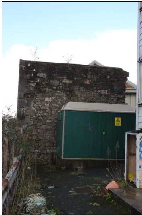
Photograph 26 General view of the south elevation of Building B with the sub-station obscuring a section of the elevation
