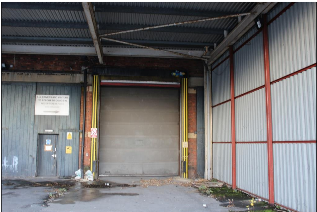
Photograph 3 Later inserted metal roller door with the remains of the stone dressings still in place
