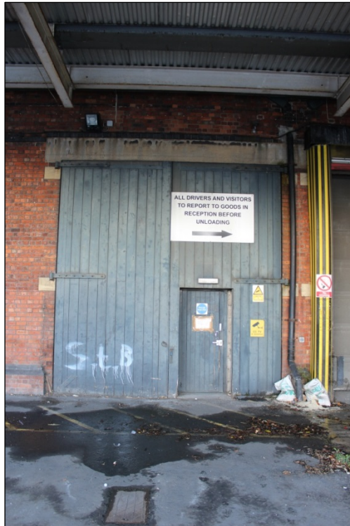
Photograph 2 Sample of the former carriage doors now blocked up on the interior with a pedestrian door inserted and stone dressing
