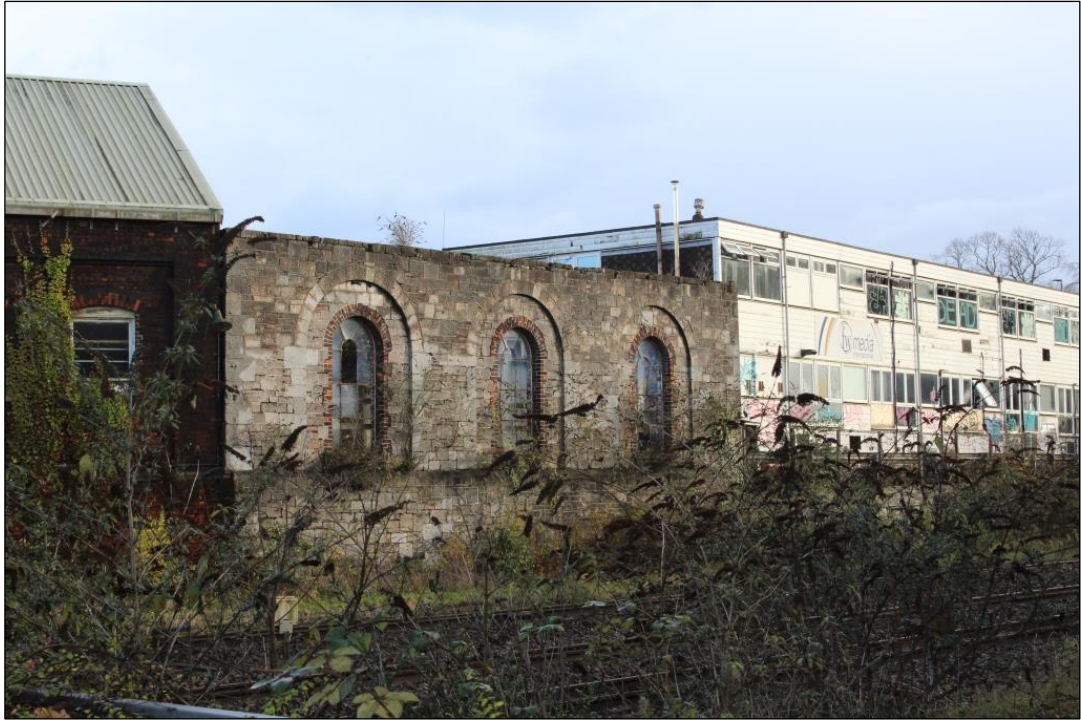
Photograph 25 General view of the west elevation of Building B as seen from the Station car park with the three arched windows
