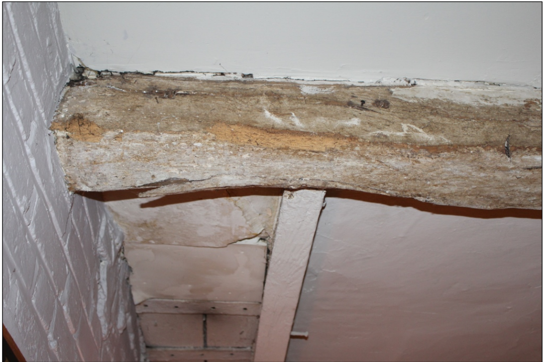
Photo 15: The northern extent of the timber beam.
