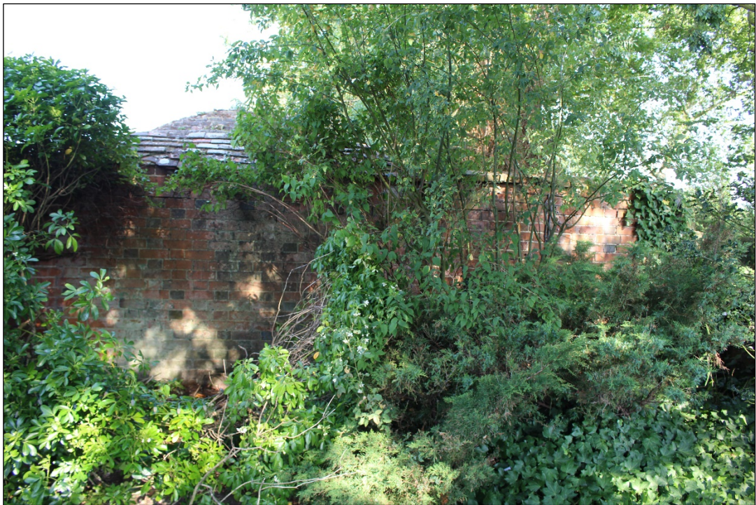
Photo 40: The section of wall at the northern extent of the beer garden.
