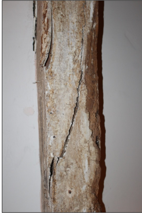
Photo 20: The underside of the northern half of the beam.
