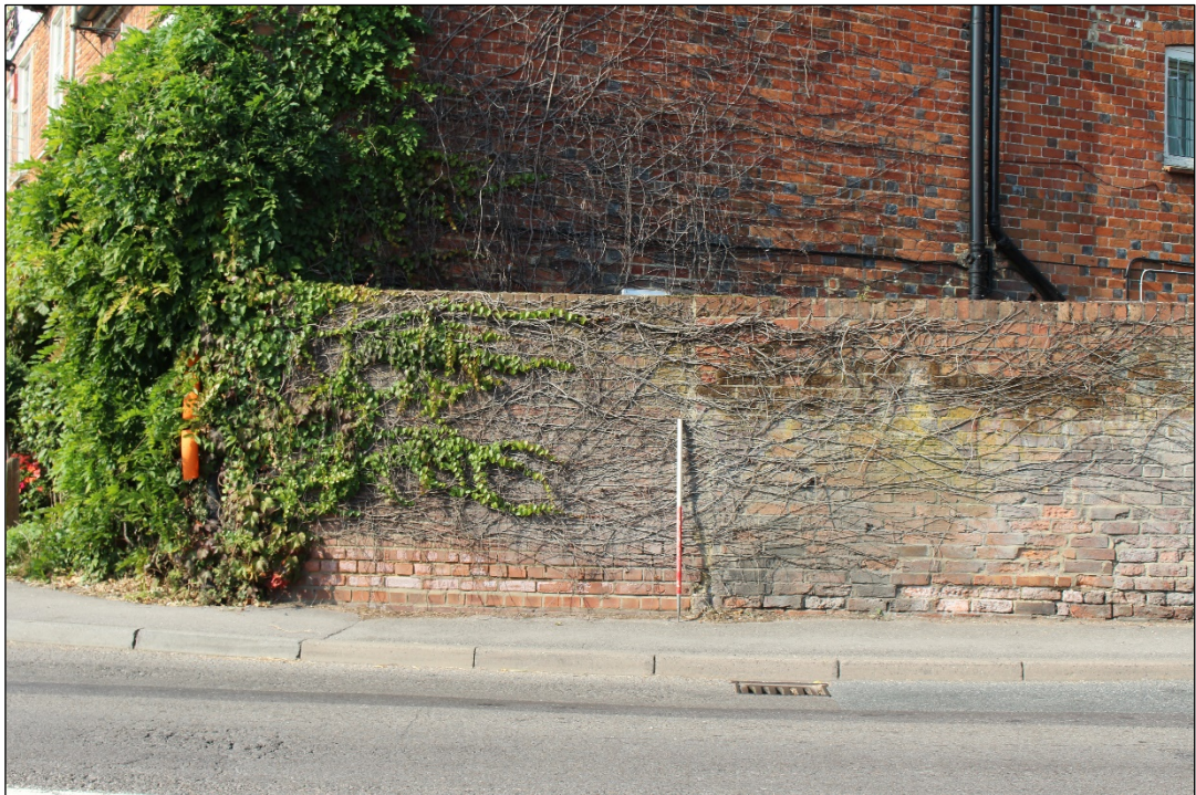
Photo 25: Detail of the re-built section (Section 1) at the southern extent of the eastern elevation.
