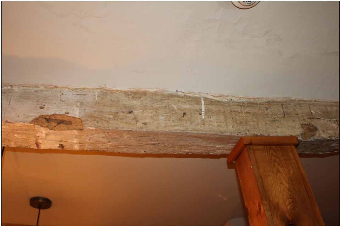
Photo 17: The eastern extent of the centre of the timber beam which is currently propped.
