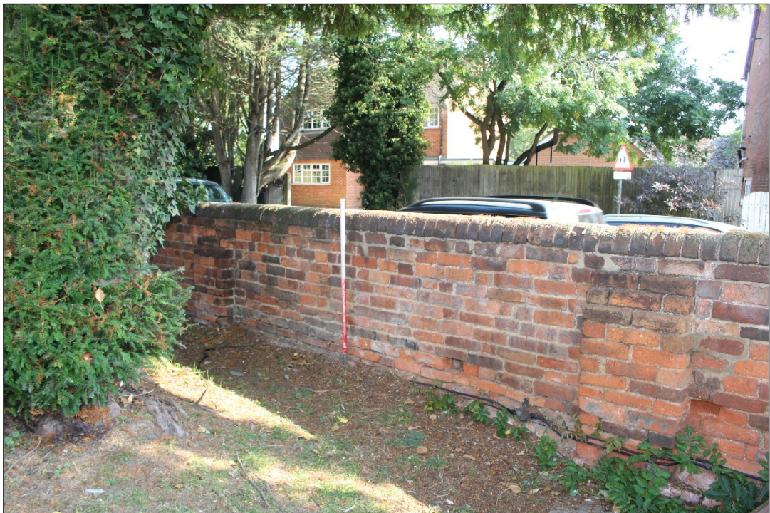
Photo 42: The southern half of Section 7 of the eastern elevation from the south-west.
