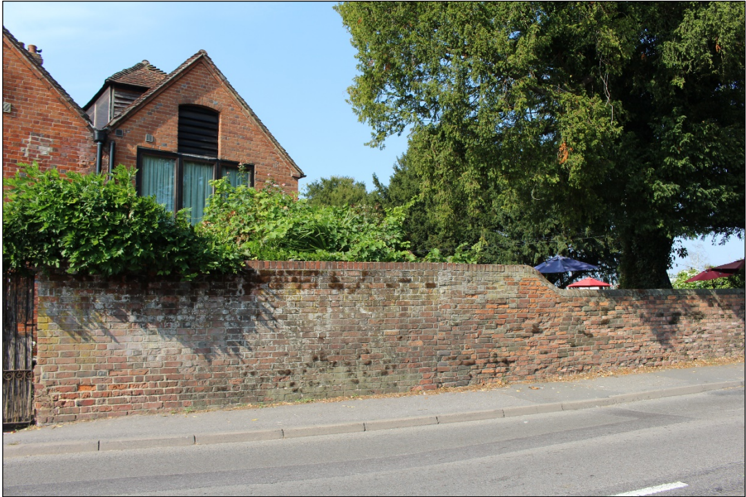
Photo 33: The southern extent of the eastern elevation of the boundary wall from the south-east.
