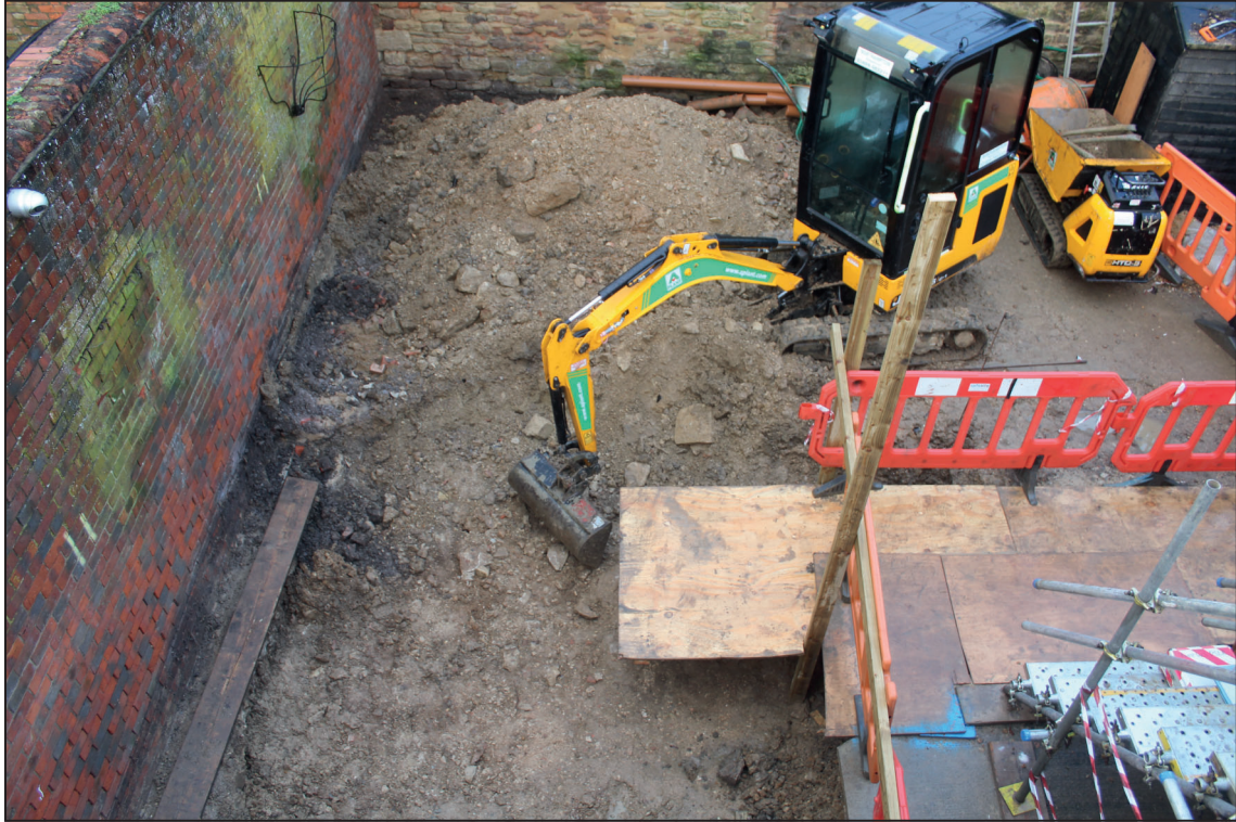
Site photograph, looking south-east towards area to be reduced to foundation level
