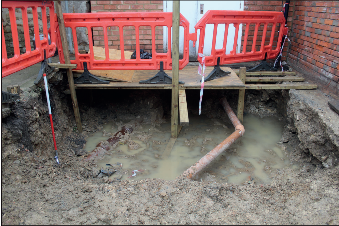
Site photograph, looking north-east showing area reduced to 1m below present ground level
