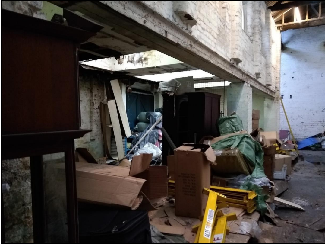
Photo 89 View of the steels supporting the eastern wall of the western linear range, plus the lightwells of the infilled courtyard
