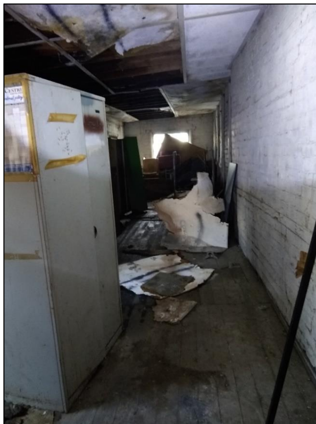
Photo 110 View of rear linear upper floor room of building C of Building 9
