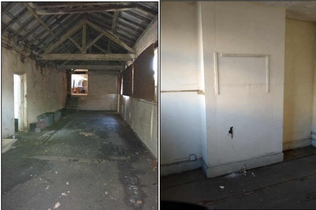
Photo 93 (left) View of the first floor of the frontage range of Building 8 Photo 94 (right) View of the chimney breast of first floor room in Building 8
