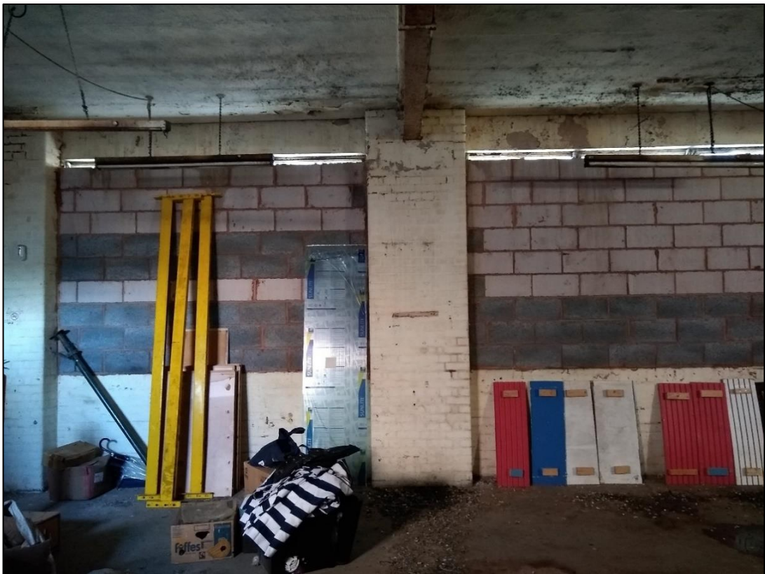
Photo 84 View of blocked windows to the front of Building 7
