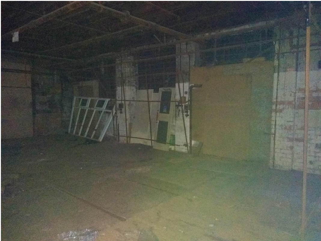
Photo 20 View of the rear (west) wall of Building 3 showing the large industrial windows fronting towards Great Hampton Street
