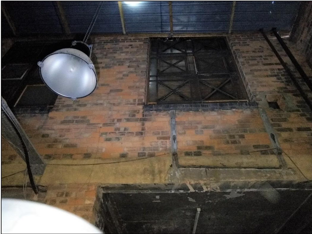
Photo 4: The rear façade of No.33 Great Hampton Street in the corridor, showing industrial window to upper floor
