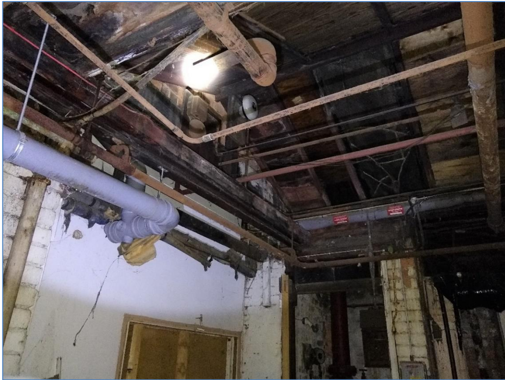
Photo 67 View of the ceiling of the west area of Building 5, this is seen externally in Photo 59
