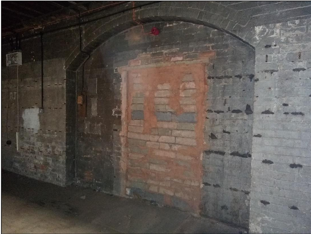
Photo 23 View of flank wall in Building 3 with blocked up opening
