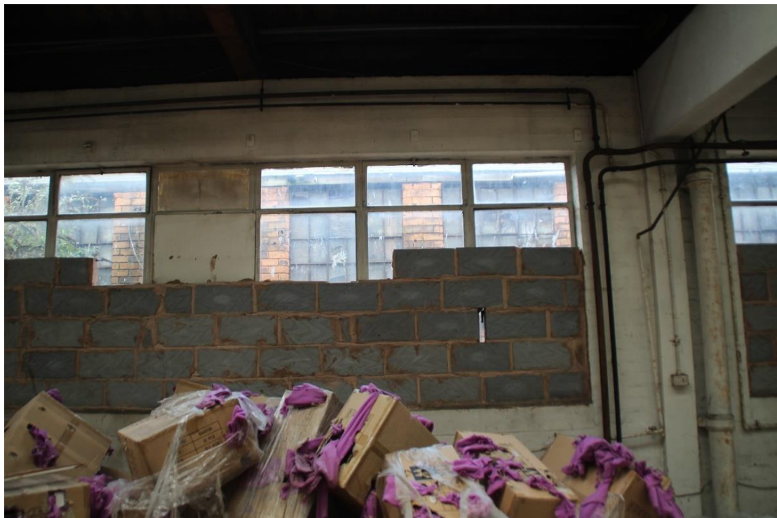
Photo 107 View from Building 6 through to the windows of building B of Building 9
