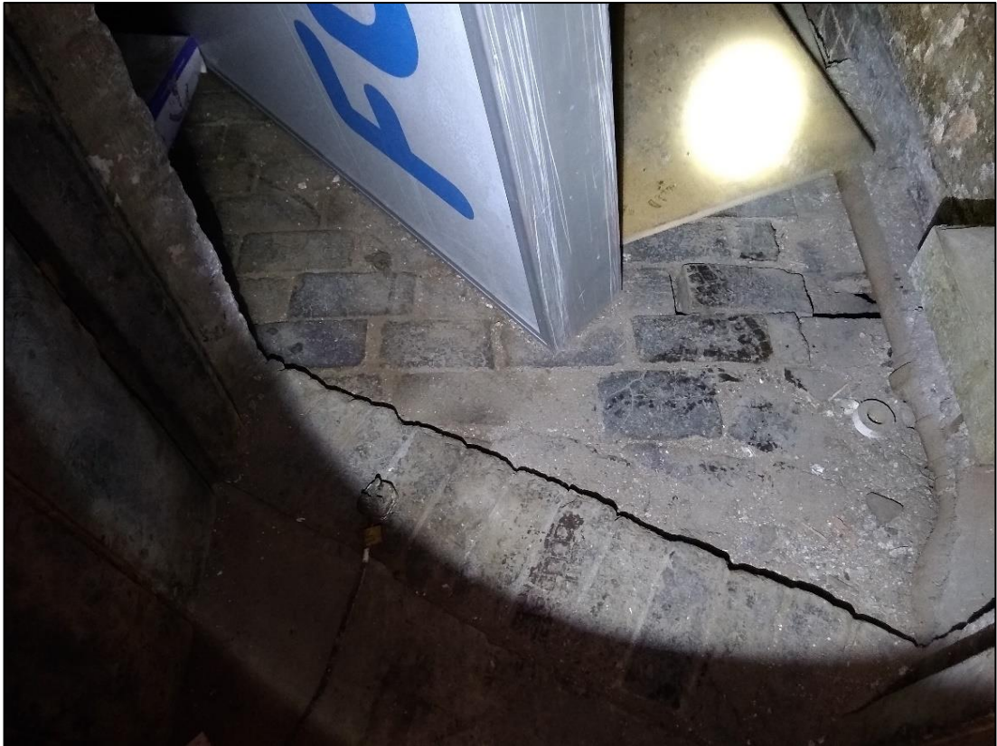
Photo 46 Floor with setts within the former yard (now interior of Building 3) connected to No.29 Great Hampton Street
