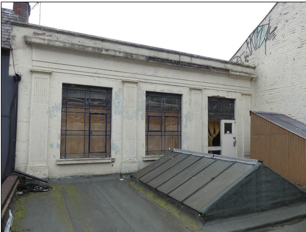
Photo 5: The flat roof element of No.33 Great Hampton Street, looking towards the original façade
