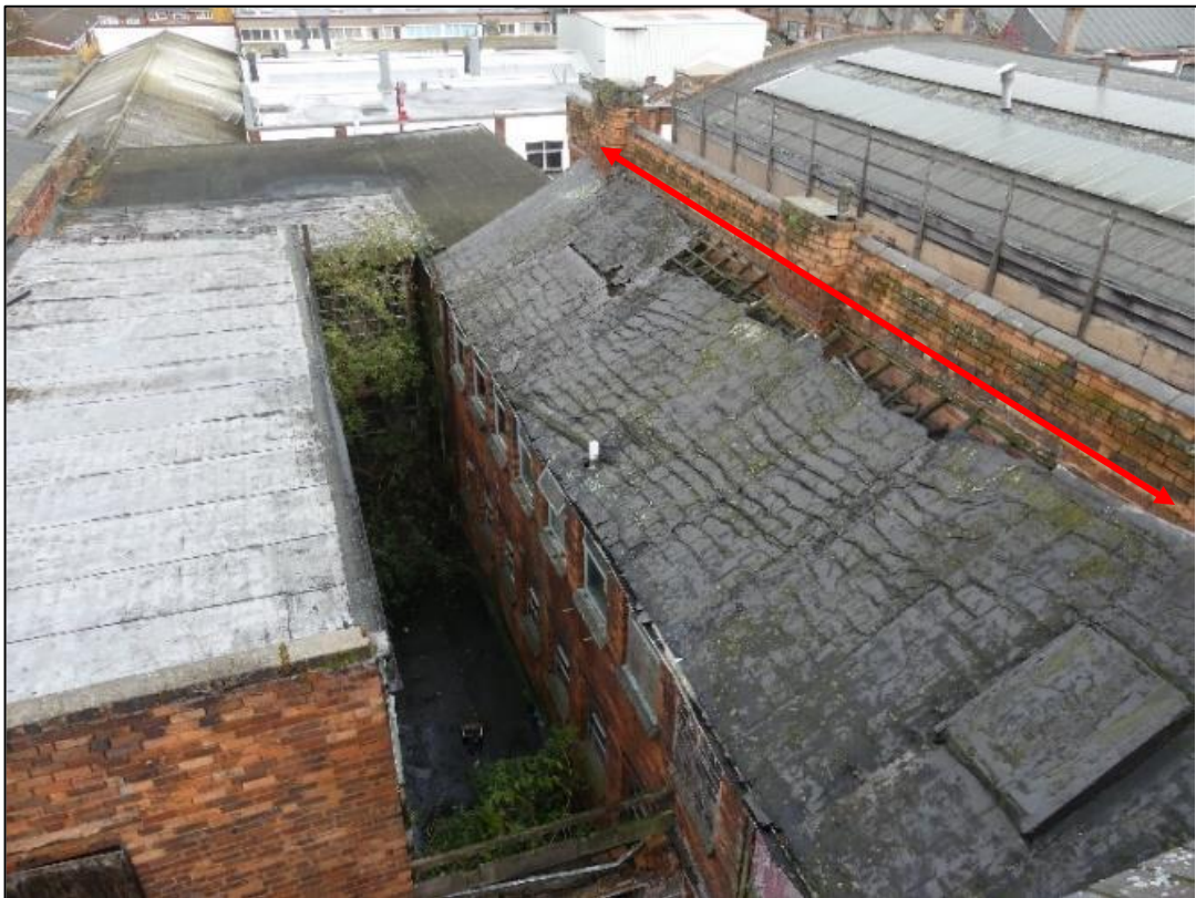
Photo 112 View of the slipped tarmac roof of building C of Building 9, with original spine wall arrowed
