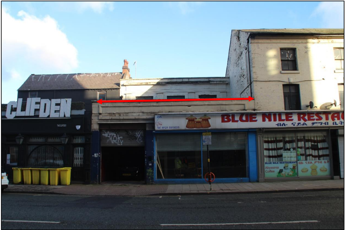
Photo 1: Principal (west) façade of No.33 Great Hampton Street, flat roof is arrowed
