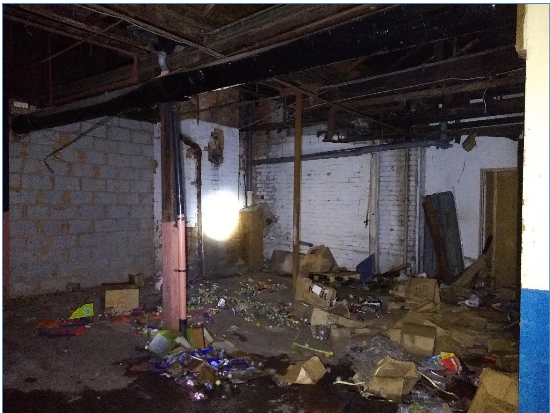
Photo 66 View of the rear (west) of Building 5 where the former yards to No.27-29 Great Hampton Street were located
