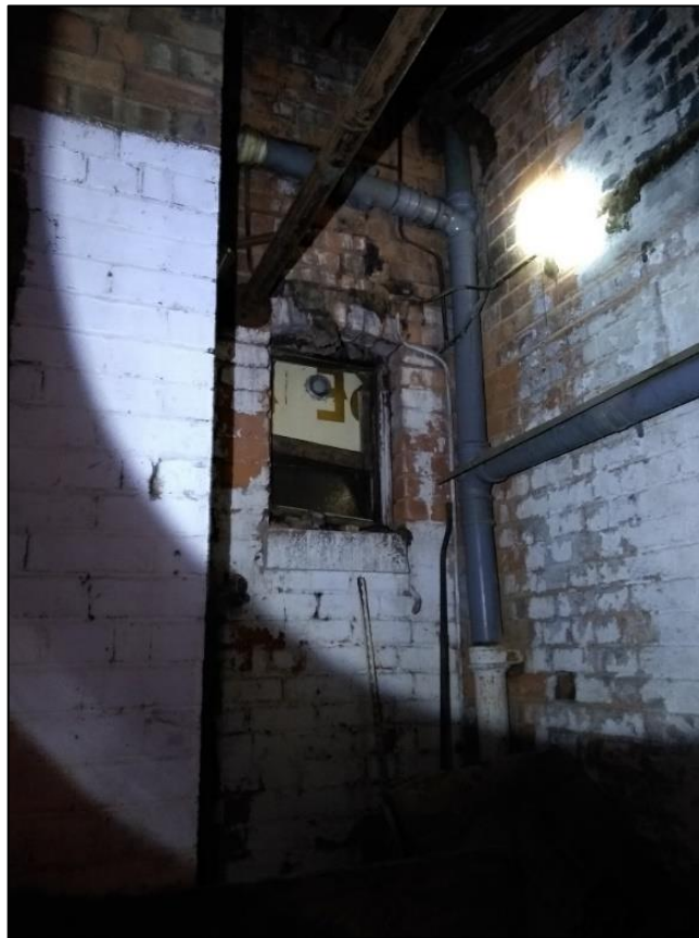
Photo 68 View of former window to the rear of No.28 Great Hampton Street
