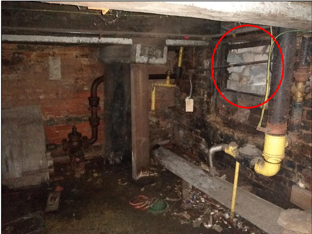
Photo 55 View of the west wall of the basement with blocked light well (circled)
