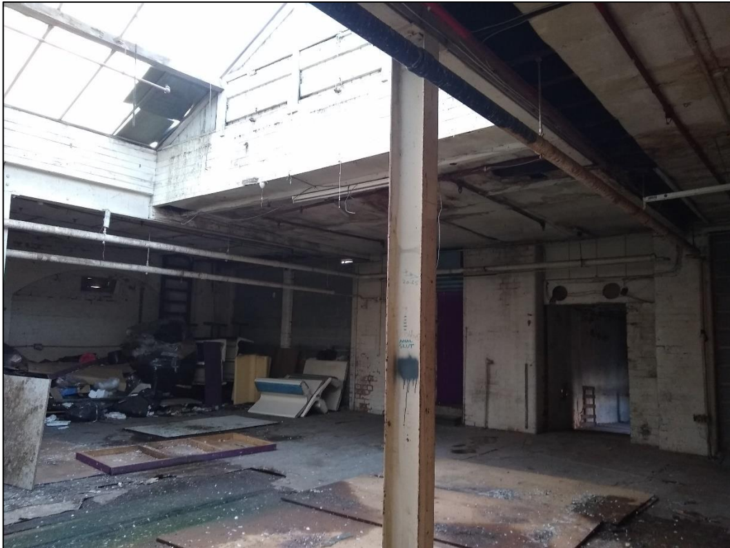
Photo 26 View of the second floor in Building 3 looking towards No.,30 Great Hampton Street
