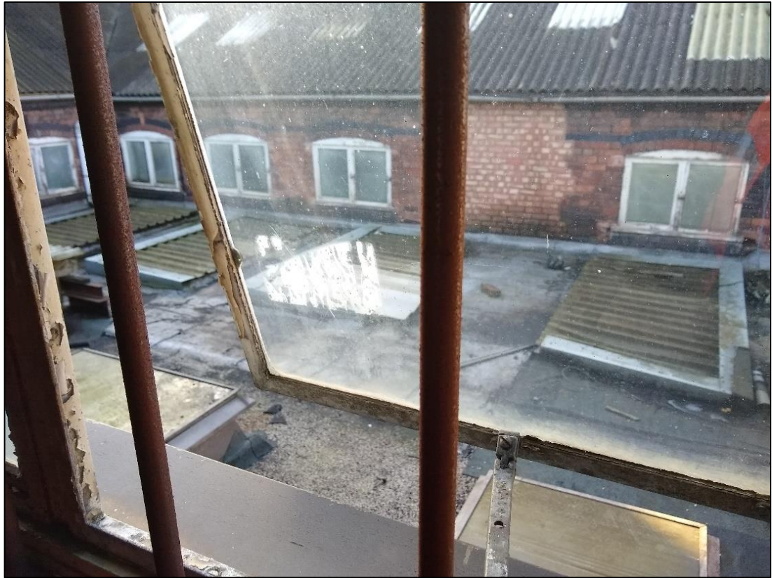
Photo 97 View of the first-floor windows of the linear ranges encircling the former (now covered) courtyard in Building 8
