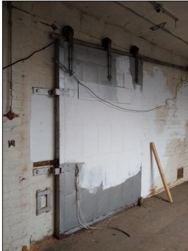
Photo 9: The large metal door between the first floor of Building 1 accessing No.30 Great Hampton Street
