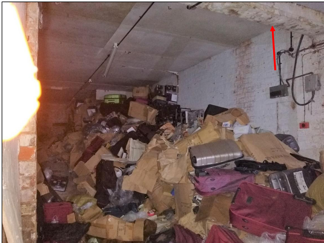
Photo 102 View of interior room of No.56A Barr Street viewed from passageway (chamfered beam arrowed)
