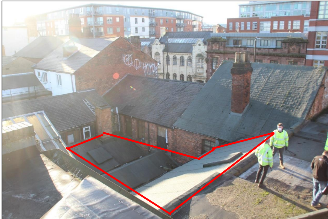
Photo 59 The ad hoc roof coverings of Building 5 at its western end, which comprise the former yards of No.27 and 28 Great Hampton Street
