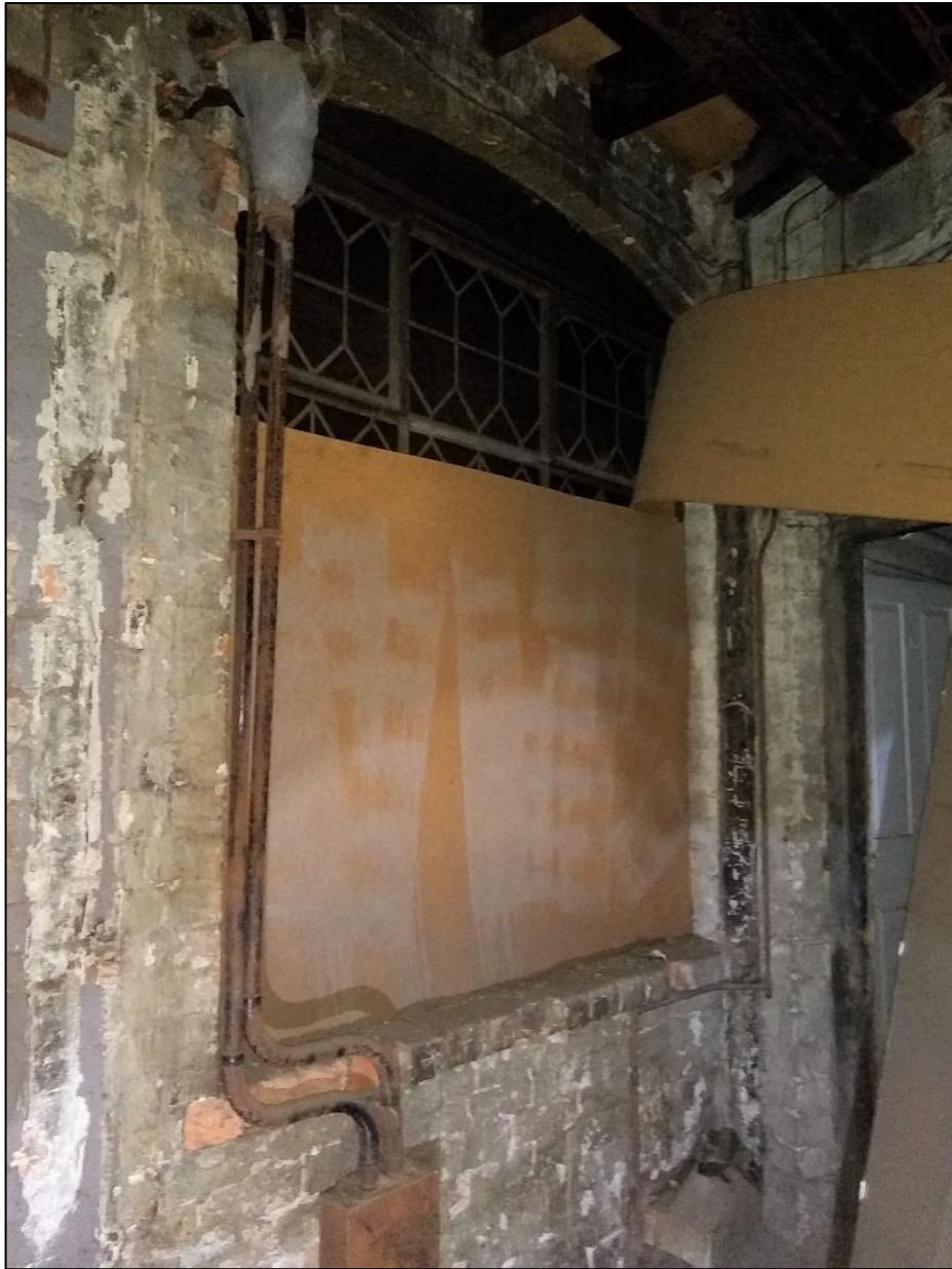
Photo 47 View of partially blocked window overlooking a former external area in No.29 Great Hampton Street (now seen internally in Building 3)
