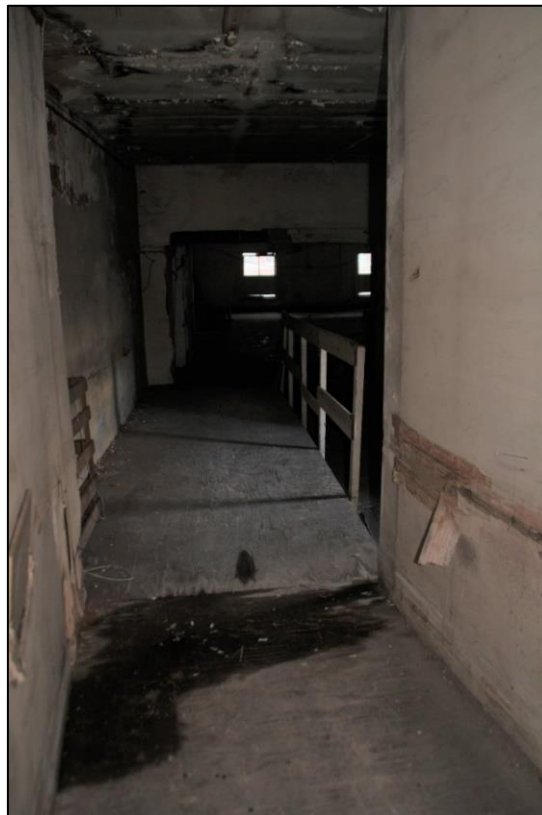
Photo 27 View of the ramp arrangement extending eastwards from Building 3 to No.30 Great Hampton Street
