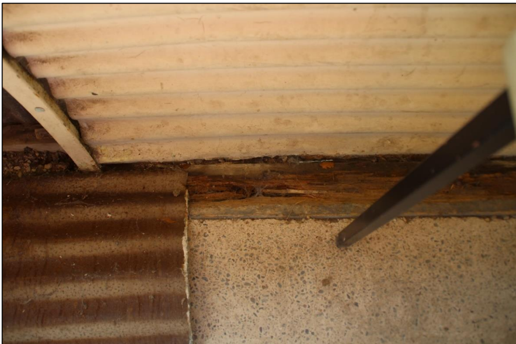
Photo 32: View of timber plinth to concrete floor and gapping to the exterior
