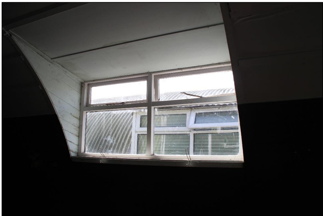
Photo 35: View of dormer with timber window and tongue and groove cheeks (Hut 77)
