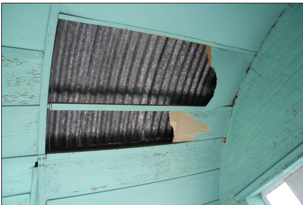
Photo 49: View of cladding and void, hut 72
