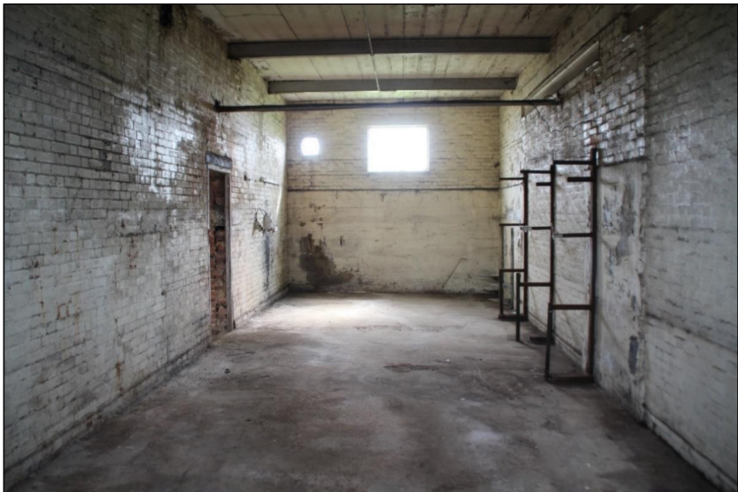
Photo 55 View of the pump room looking east
