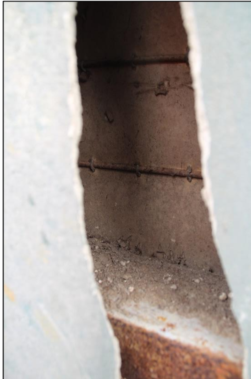
Photo 18 Detail of the internal void and materials on store block 2
