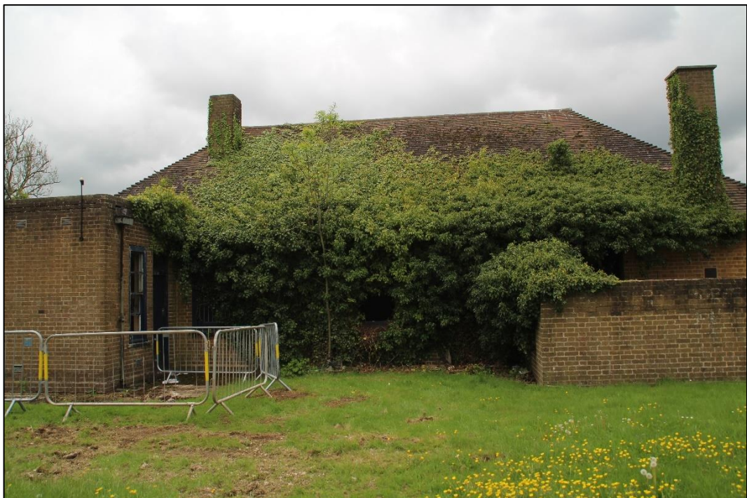
Photo 65 View of the rear of the Warden's Building showing the two outshot, the right being a small rear yard
