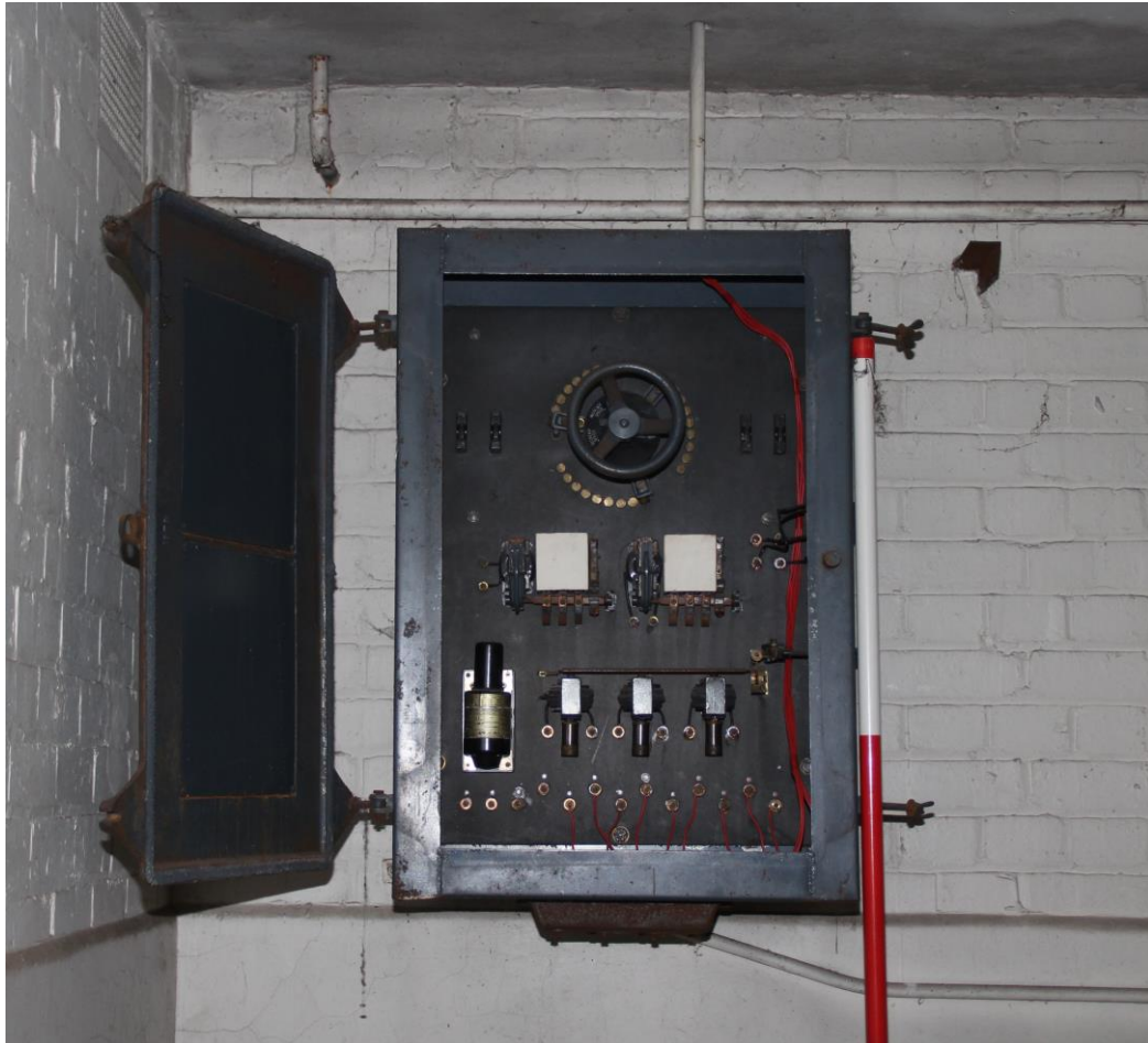
Figure 13 Room G8 in Building 1, the electric motor control box
