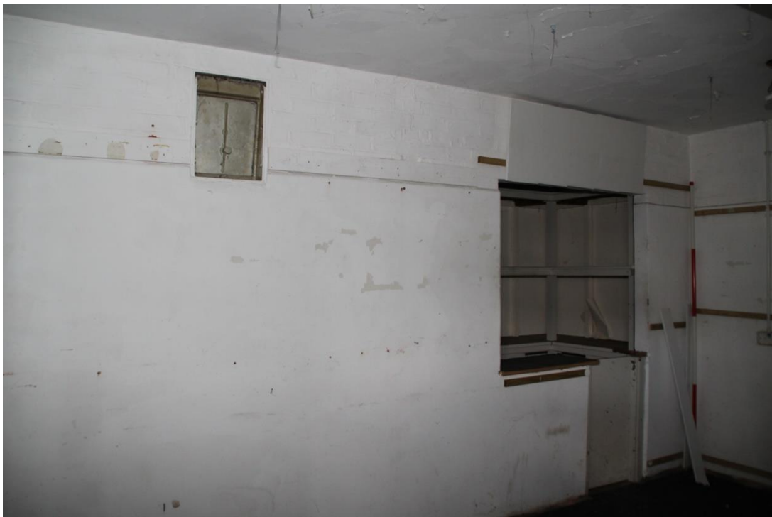
Figure 10 Room G2 in Building 1, the recess G4 and the steel lined duct from G3, looking south-east (scale 2m)
