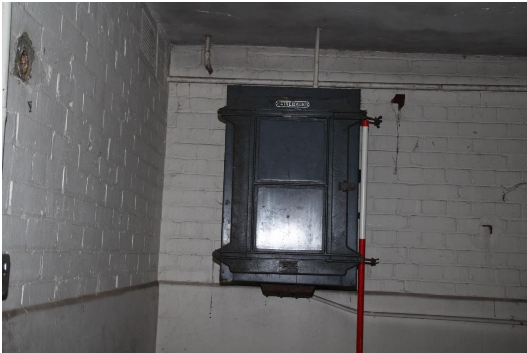
Figure 11 Room G8 in Building 1, the electric motor control box and half height plastering (scale in 0.5m divisions)
