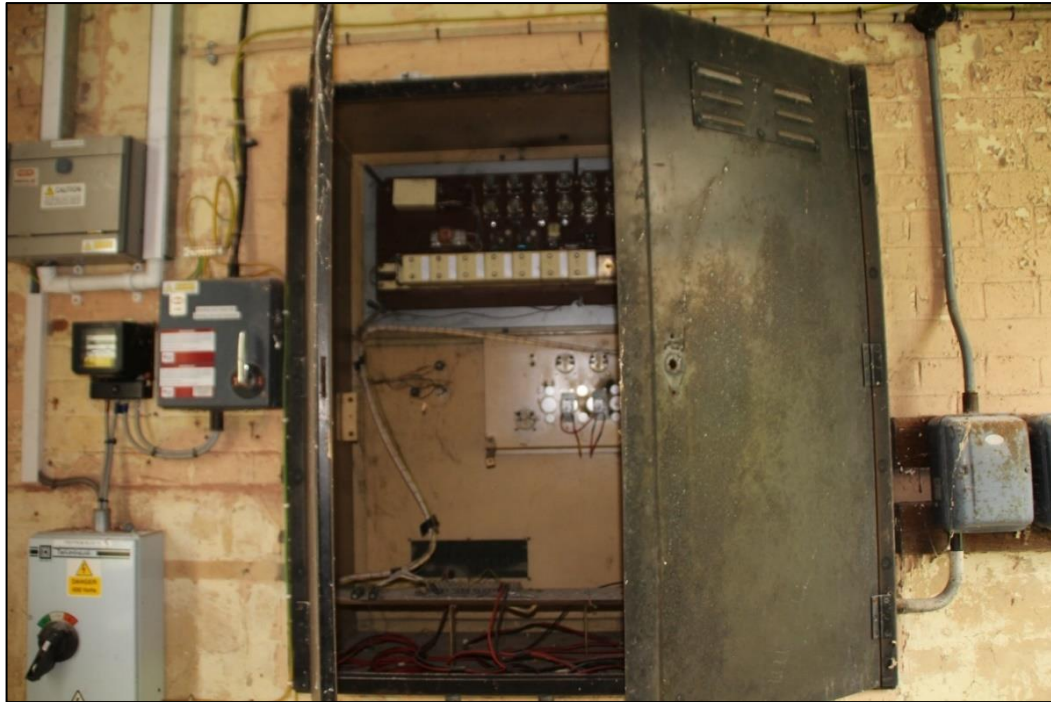
Photo 70 View of remains of electrical circuit board, Warden's Building
