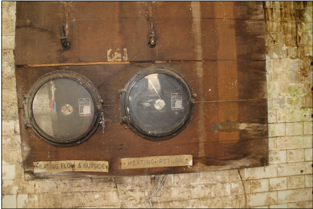
Photo 54 View of remains of heating control equipment
