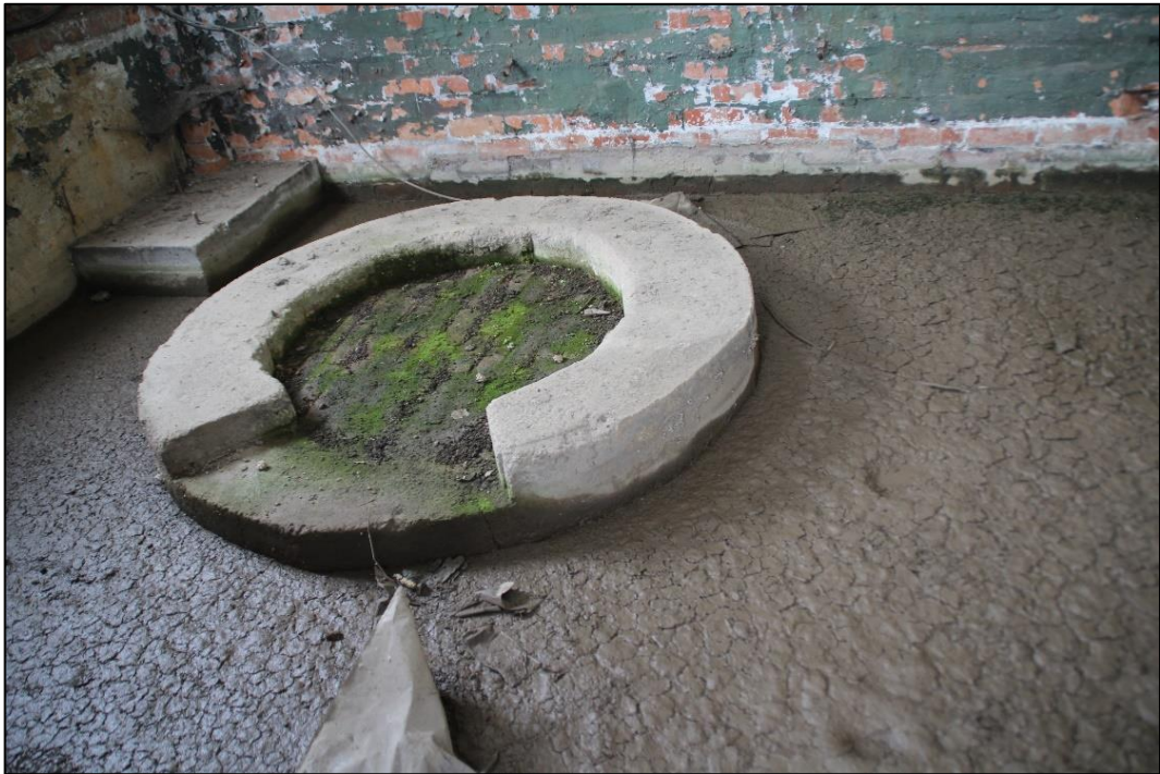
Photo 30 View of the circular concrete plinth in the full-height corner room of store block 2
