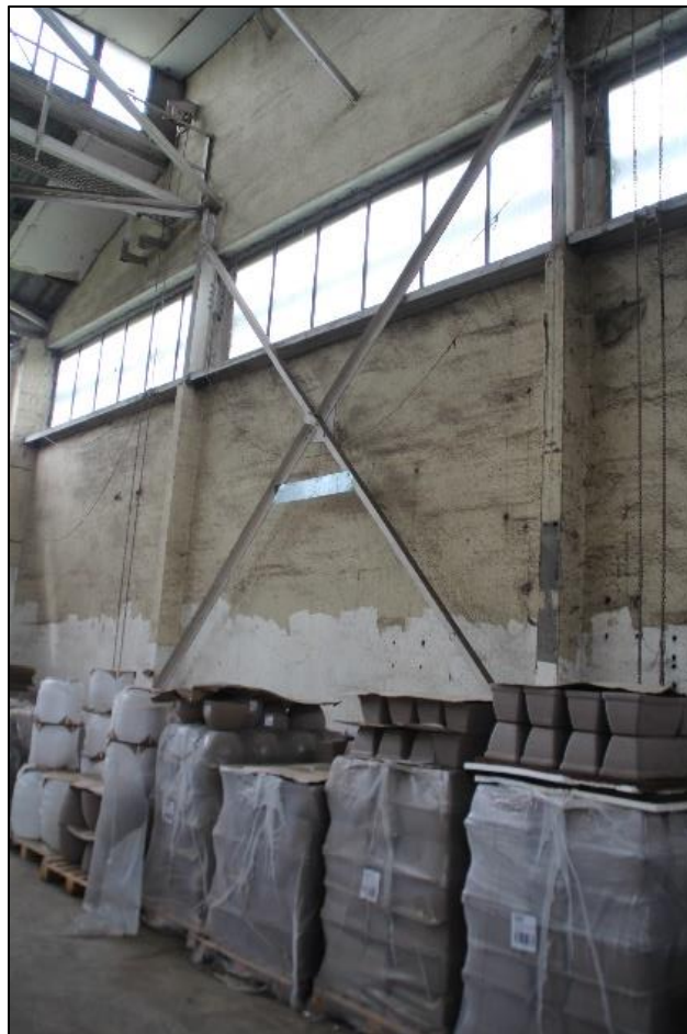
Photo 23 View of a cross brace on an internal wall face on store block 2
