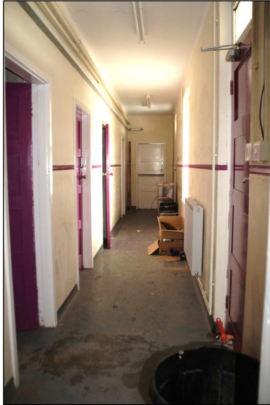
Photo 71 View of the internal spine corridor of the Warden's building with the reception area at the far end with a stable door arrangement
