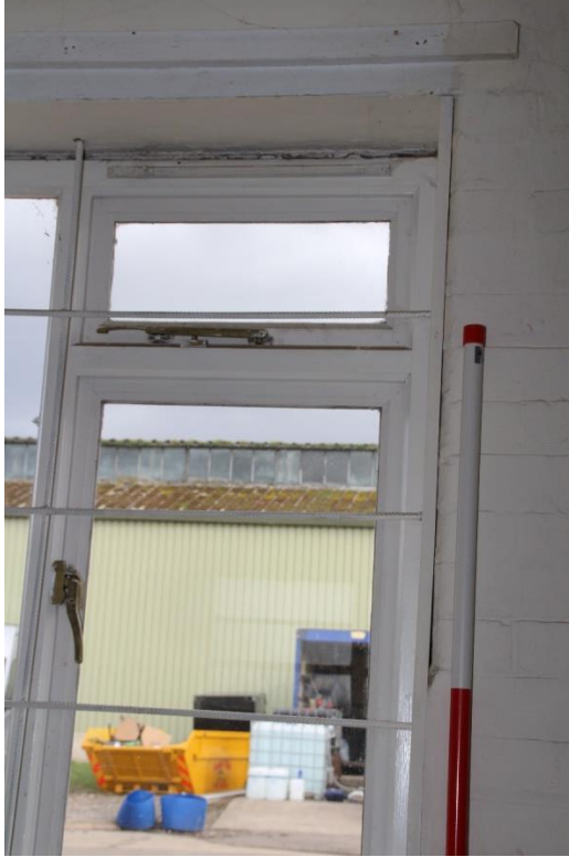
Figure 34 Building 3, detail of extended windows in Room G2, looking west (scale 0.5m divisions)
