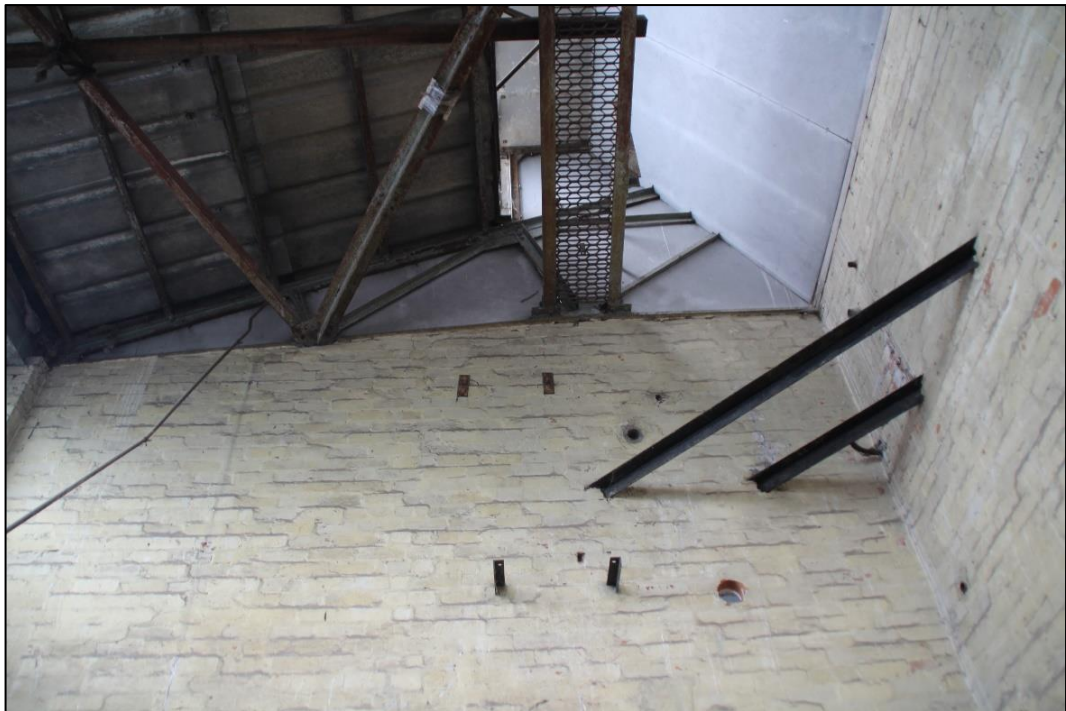
Photo 32 View of structural ties in the upper parts of the corner room of store block 2
