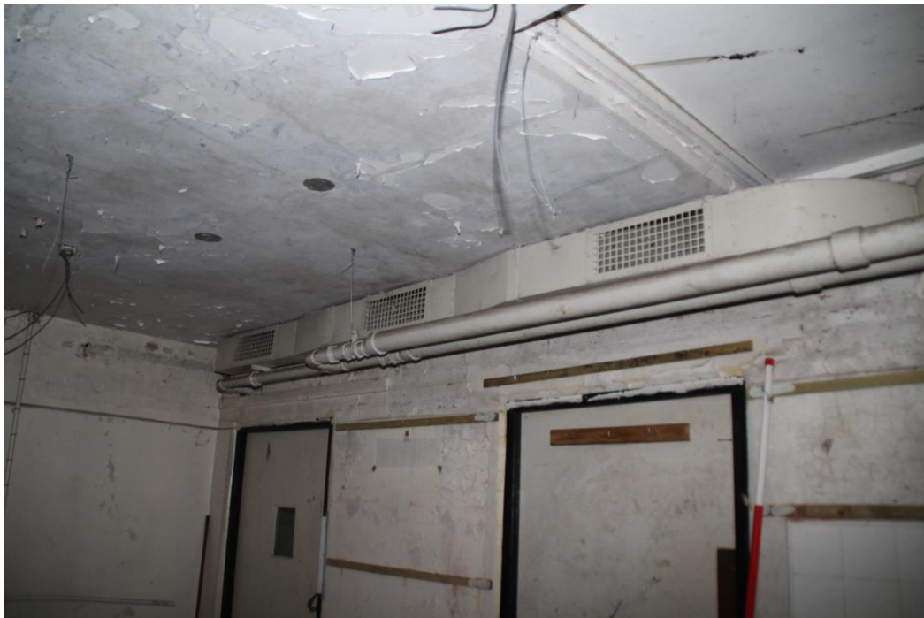
Figure 12 The pipes and ductwork in Room G6 in Building 1, looking south-west
