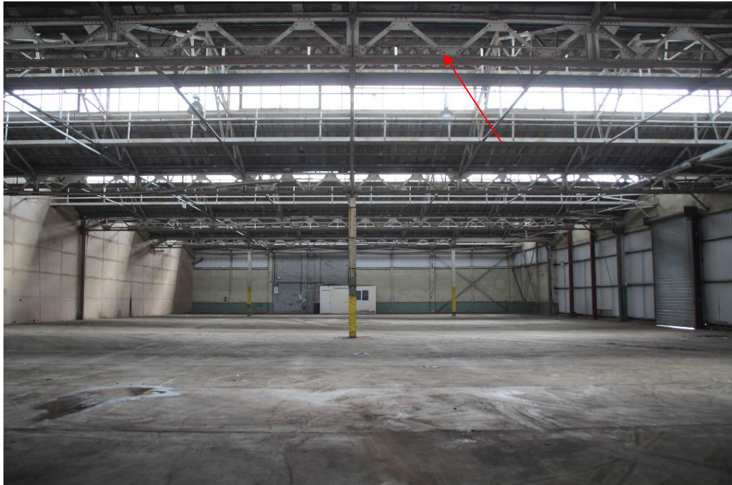
Photo 5 Internal view of store block 1 looking east (arrow showing the lattice steel structure at the nadir of each linear roof structure)
