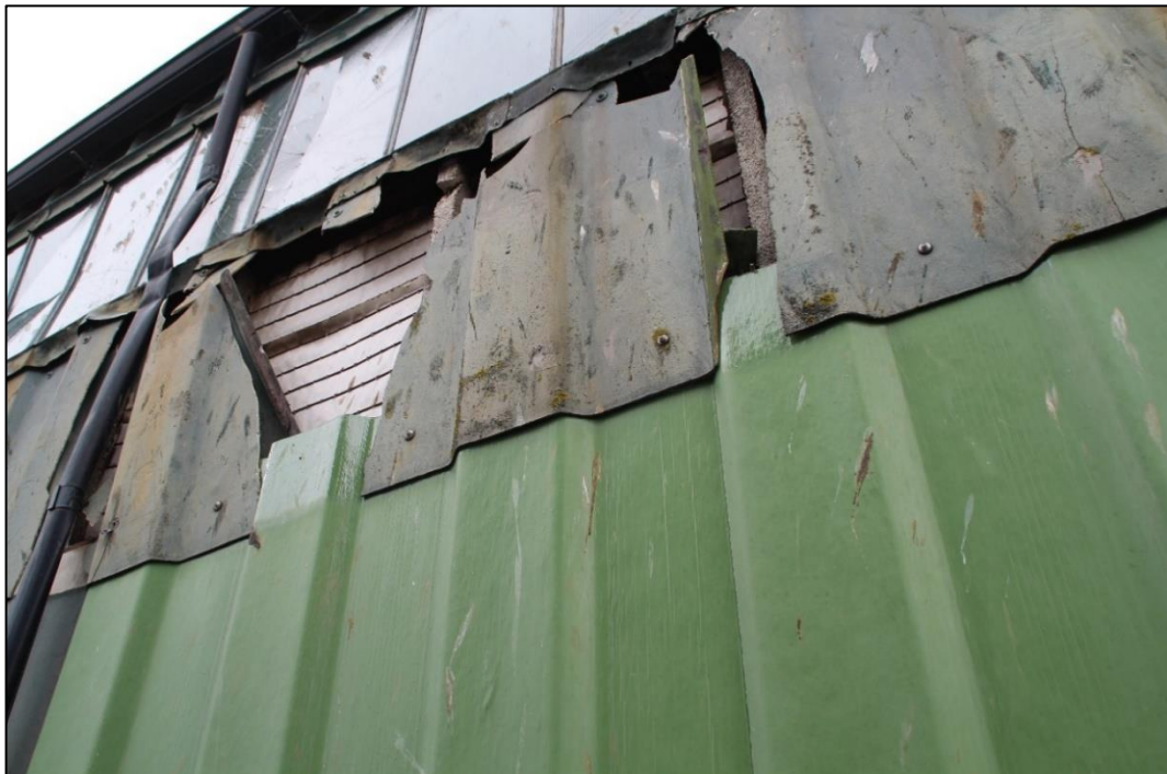
Photo 19 View of broken cladding, internal fabric and under eaves glazing of store block 1
