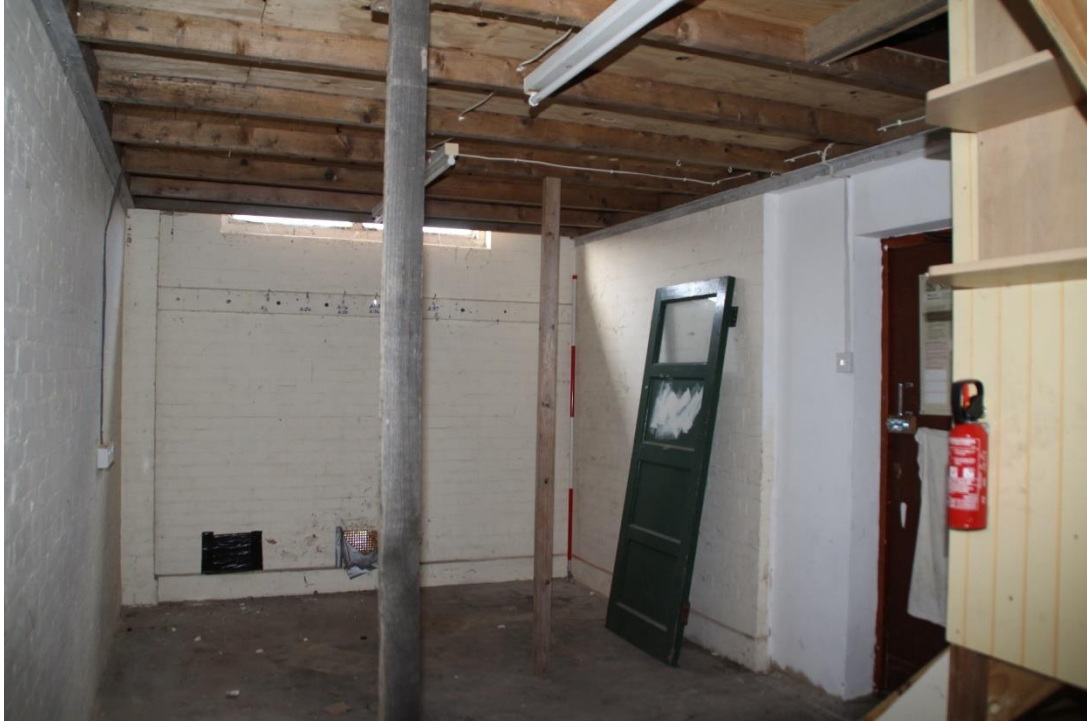
Figure 23 Room G1 in Building 2 showing the inserted first floor. The stair is just visible on the right (scale 2m)
