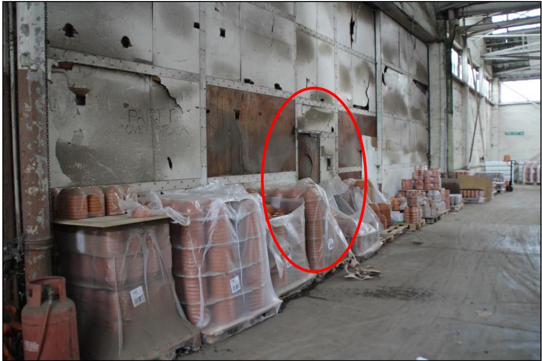
Photo 21 Internal view of the sliding metal framed doors (wicket door encircled in red)
