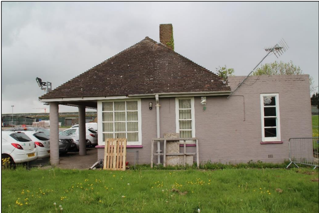
Photo 69 View of the eastern elevation of the Warden's building, incorporating the electrical room to the rear
