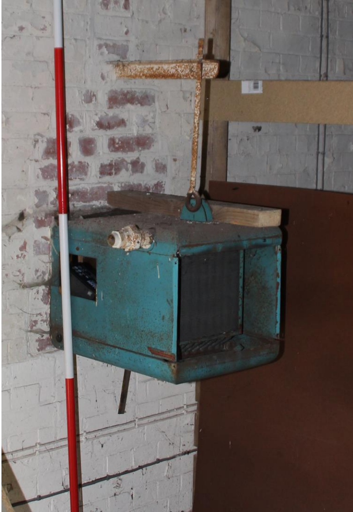
Figure 27 The interior of the ducting on the north gable of Building 2 (cf fig. 21) Scale in 0.5m divisions
