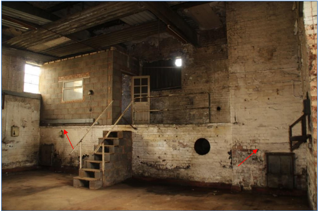
Photo 52 The interior of the CHS main boiler room with early coal chutes arrowed
