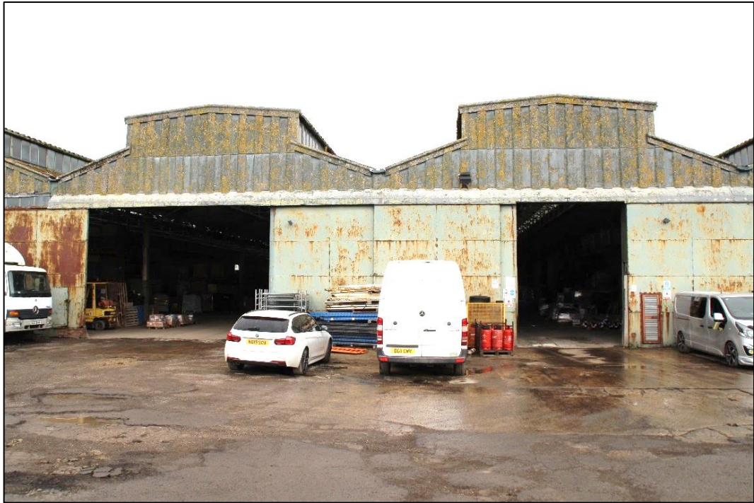
Photo 37 View of the sliding doors in use on store block 3, southern elevation
