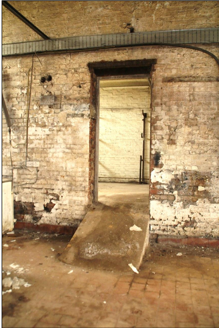
Photo 56 View of the sloped access between the main boiler and pump rooms
