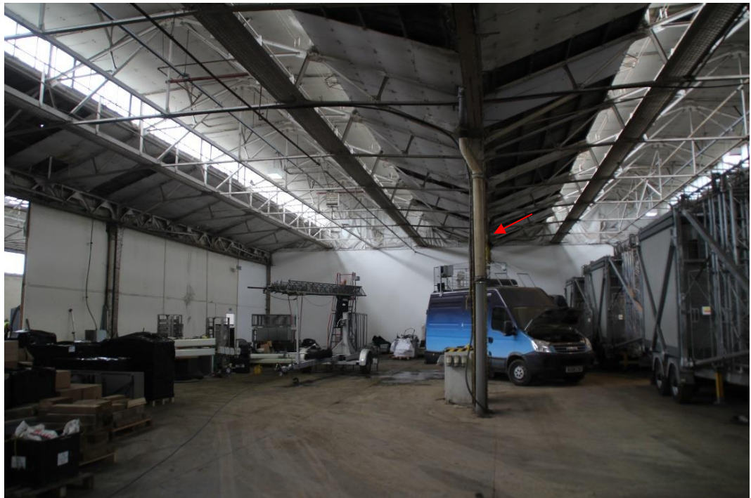
Photo 26 Internal view of eastern half of store block 2, looking east to the central wall (drainpipe arrowed)
