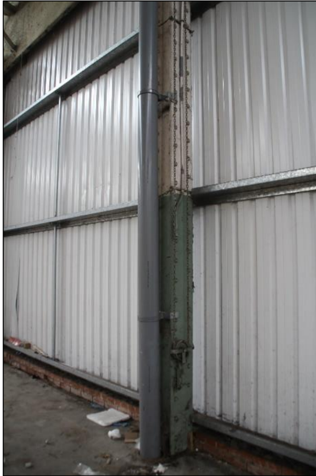
Photo 10 View of internal drainage pipe and winching equipment on stanchion – store block 1
