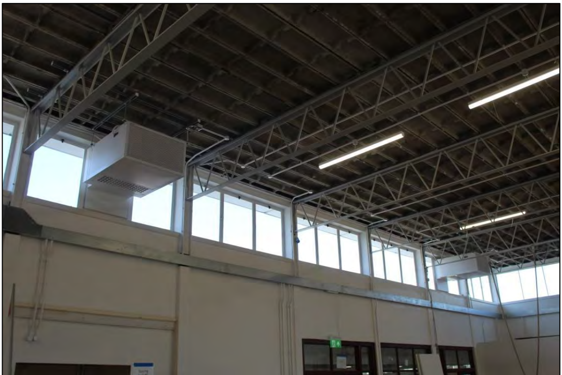
Photo 57: Ventilation units at Clerestory level in Room 8
