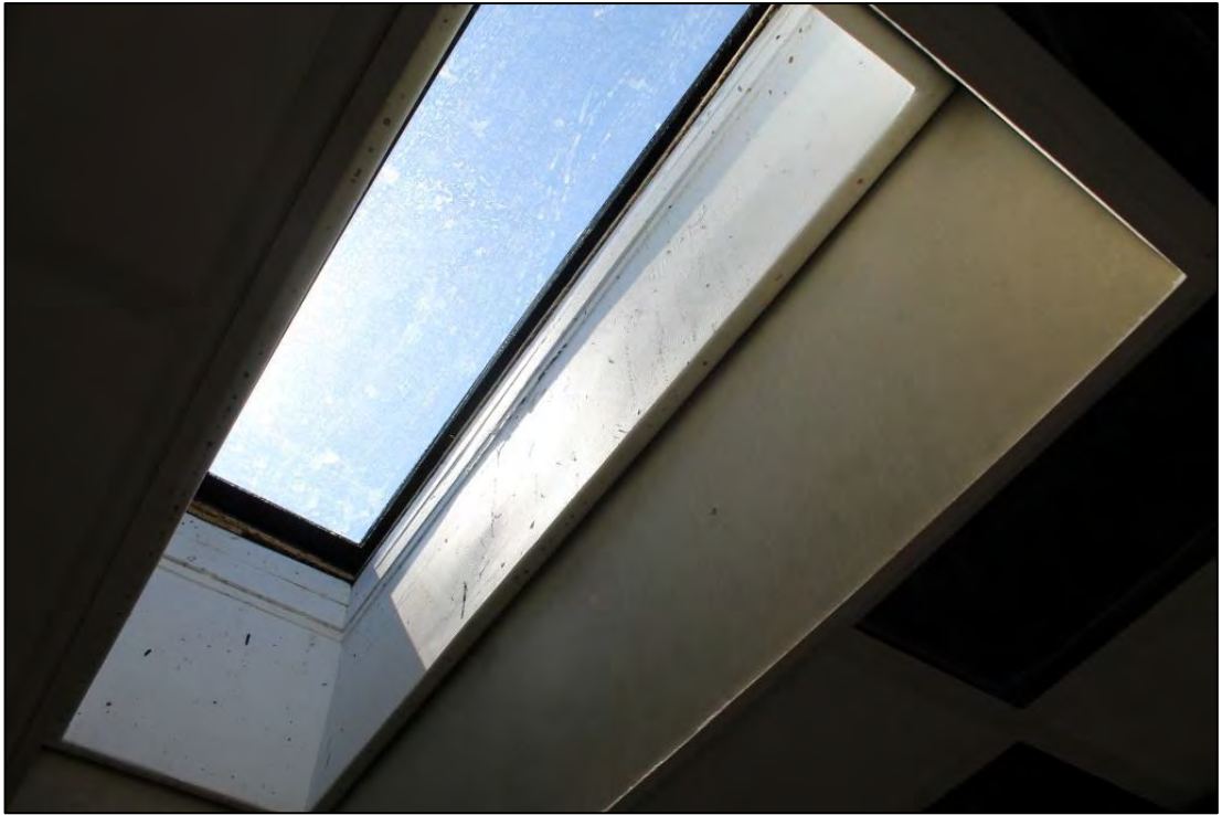
Photo 44: Replacement rooflight in Comms Room adjacent to Room 10 (ceiling glazing panel not in situ )
