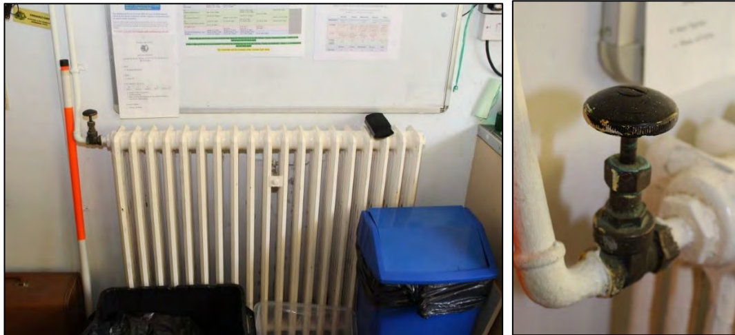
Photos 18 and 19: Detail of radiator in Room 5
