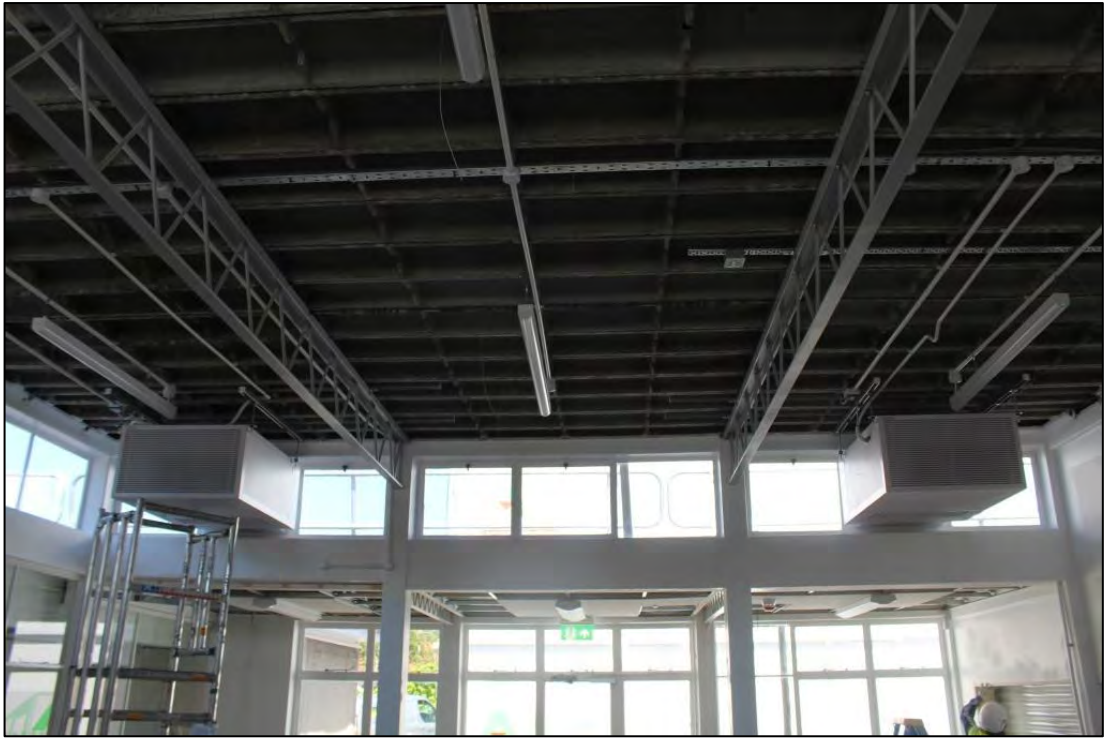
Photo 56: Ventilation units at clerestory level in Room 6
