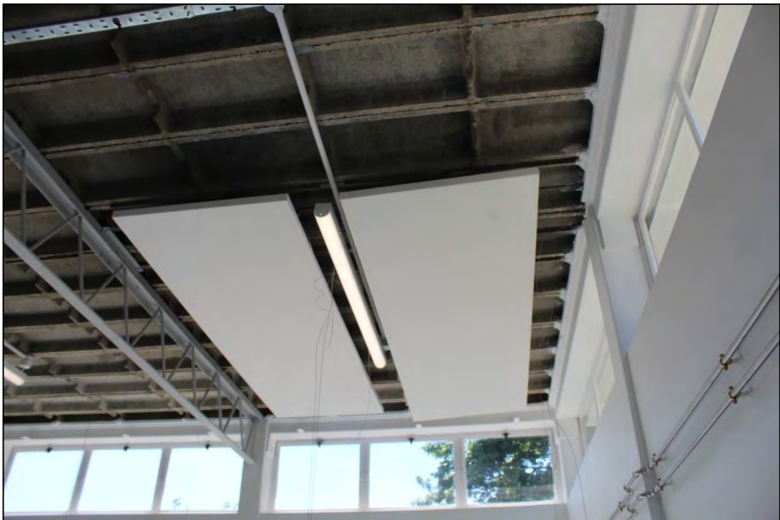
Photo 52: Acoustic panels in Room 14
