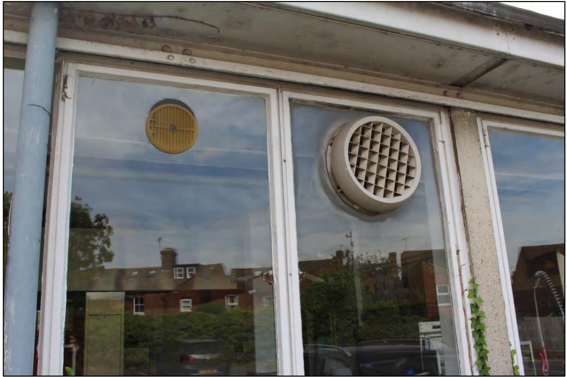
Photo 4: Detail of extraction unit within kitchen glazing
