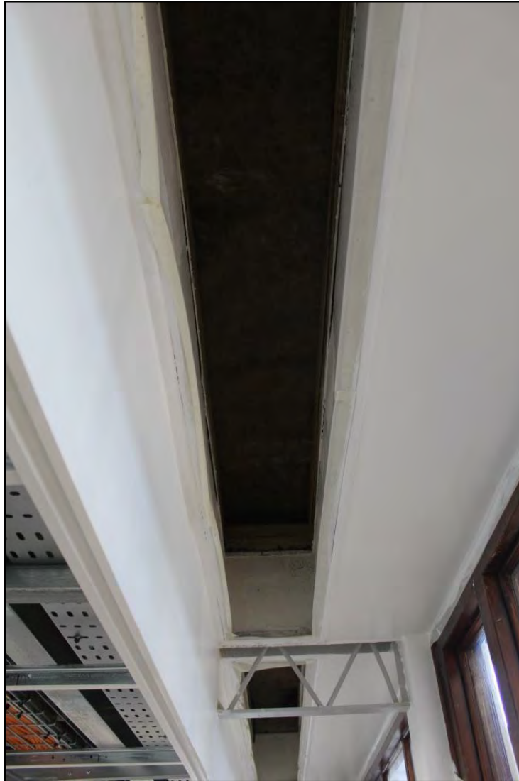
Photo 45: Position of ventilating rooflights in Room 1
