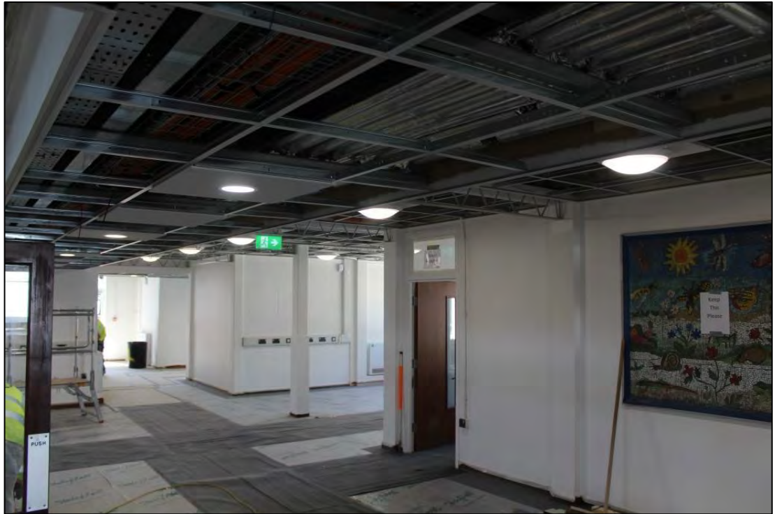
Photo 61: Electrical services in Room 1
