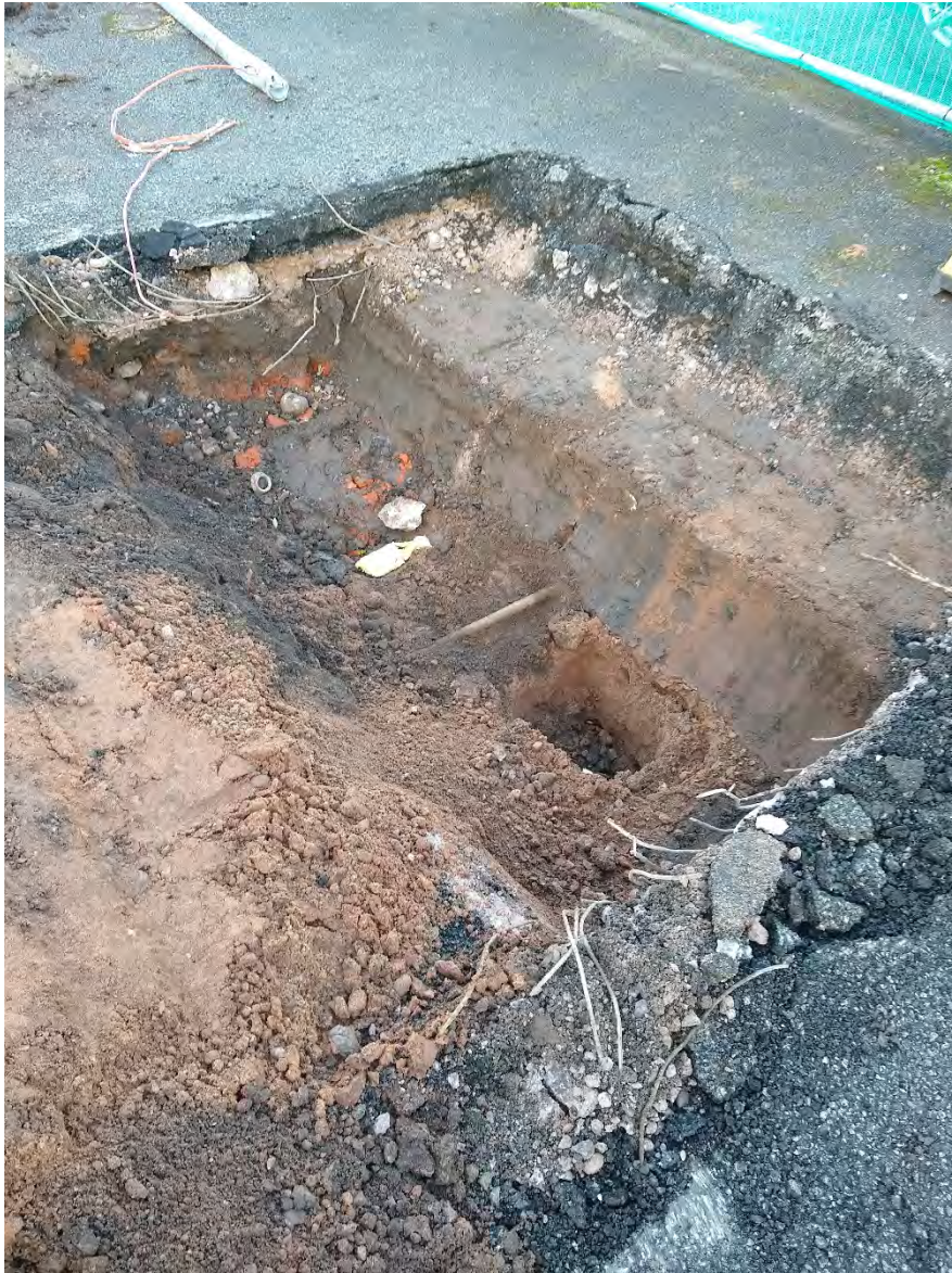
Fig. 14. Forecourt area showing service trenches and modern hard surface and sub-base directly overlaying natural sand geology
