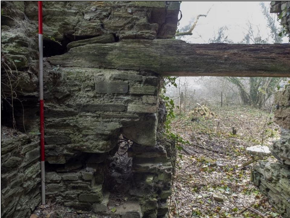
Figure 23.06 – Rotting internal lintel and hole through wall.
