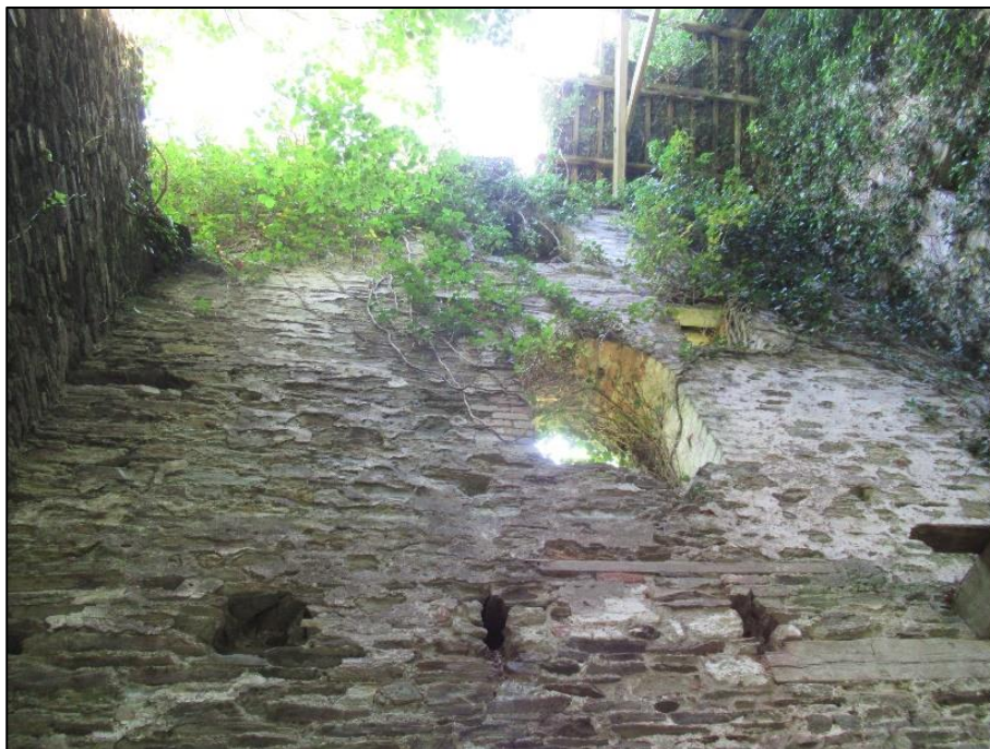
Figure 23.08 – East elevation openings, joist pockets, and lintel bearing for south intermediate level opening.
