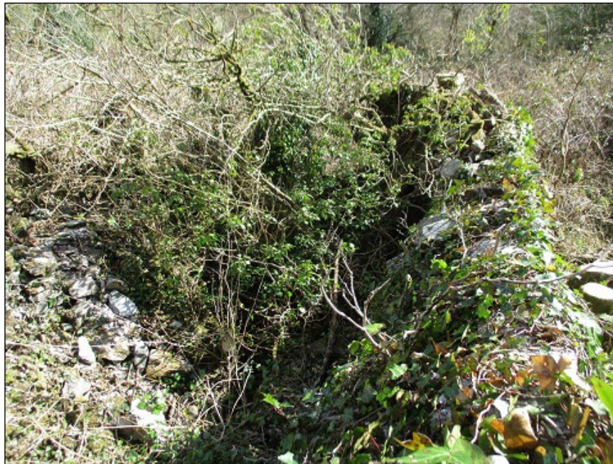
Photograph 15. Looking along the top of the Boiler House west wall at the south gable end wall obscured by vegetation and fallen masonry
