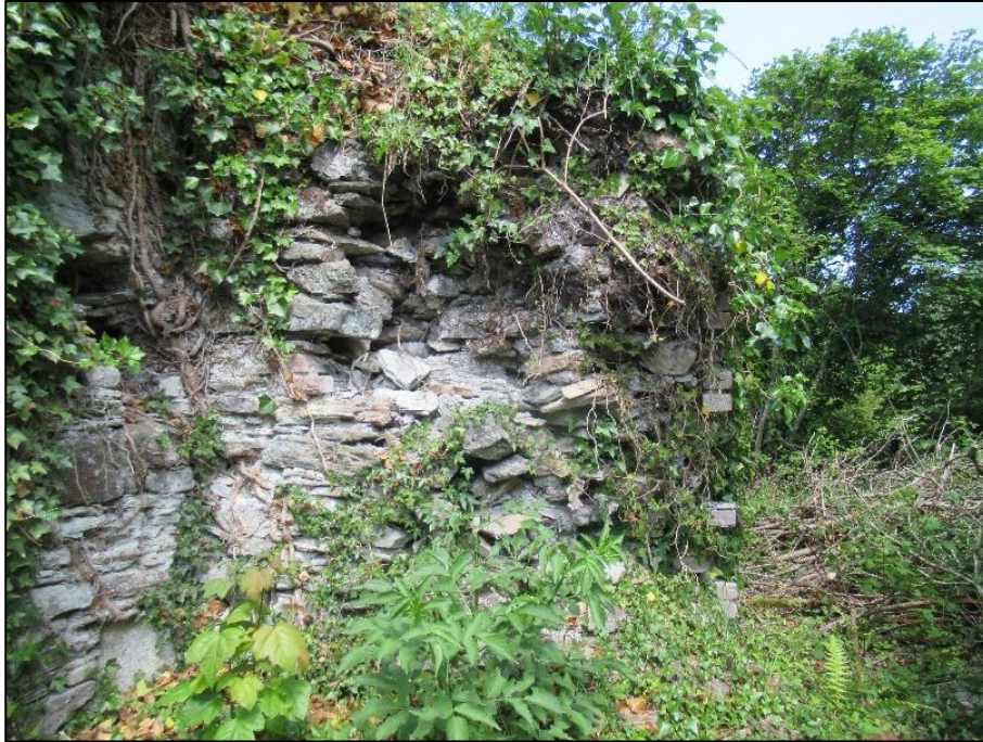
Figure 24.03 – Failed veneer at north end.
