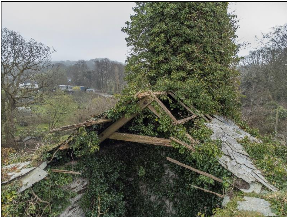
Figure 23.12 – Remaining roof structure.
