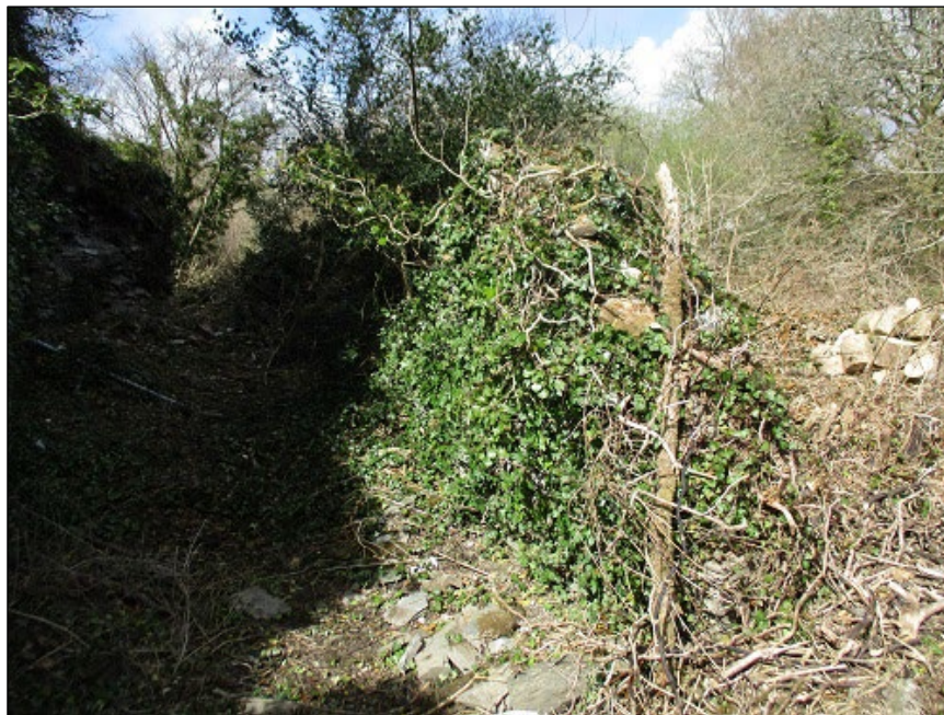
Photograph 14. East wall leaning inward, looking north from beside collapsed opening
