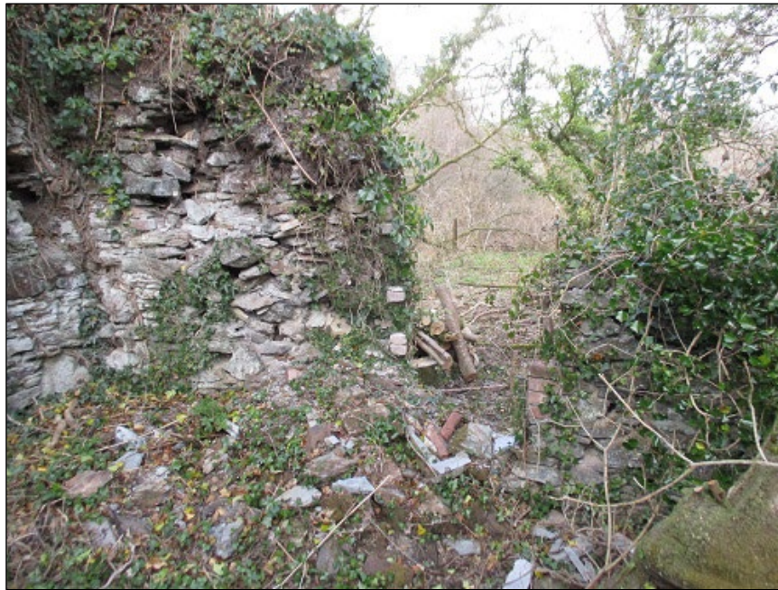
Photograph 13. North gable end wall of the Boiler House, showing failed veneer
