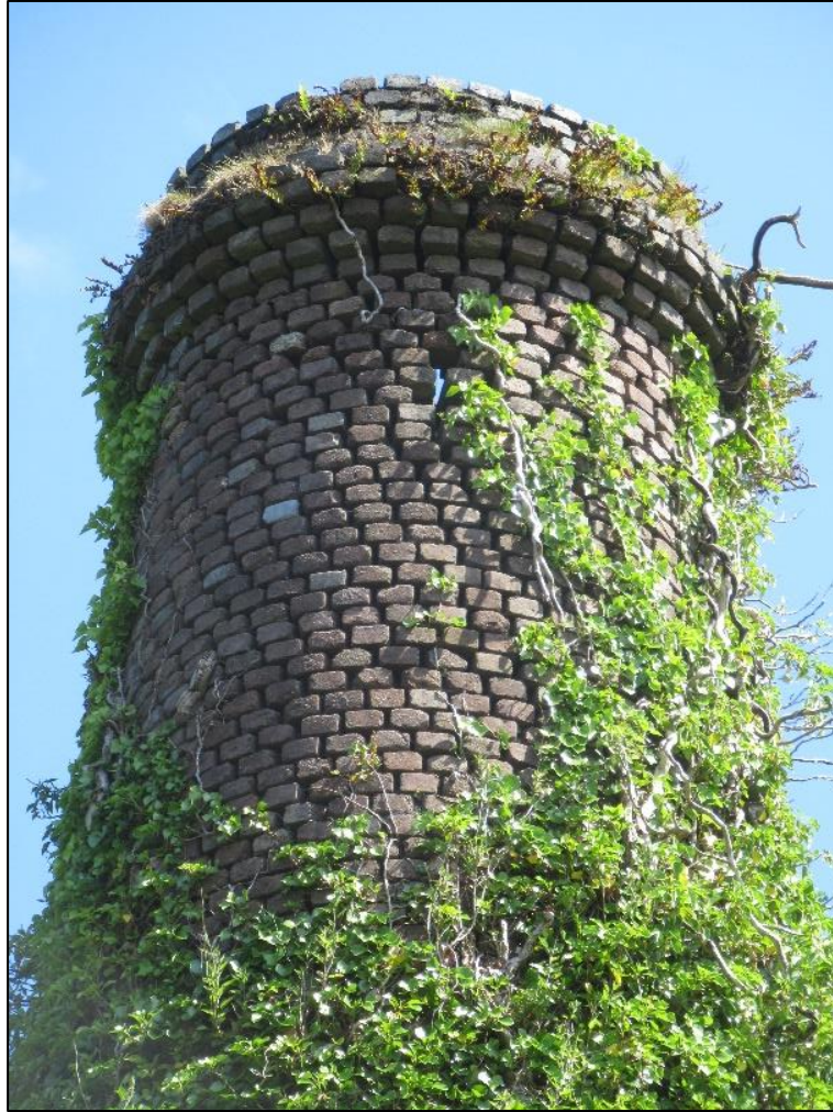
Figure 25.02 – Open jointed brickwork at upper levels of chimney
