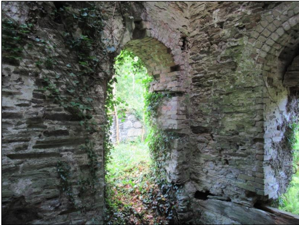
Figure 23.04 – Loose and missing bricks in reveals.
