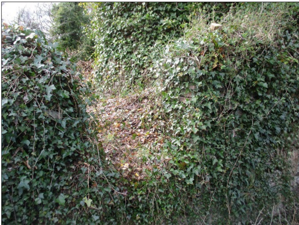
Photograph 17. Boiler House opening in west wall (ivy covered chimney base in background)
