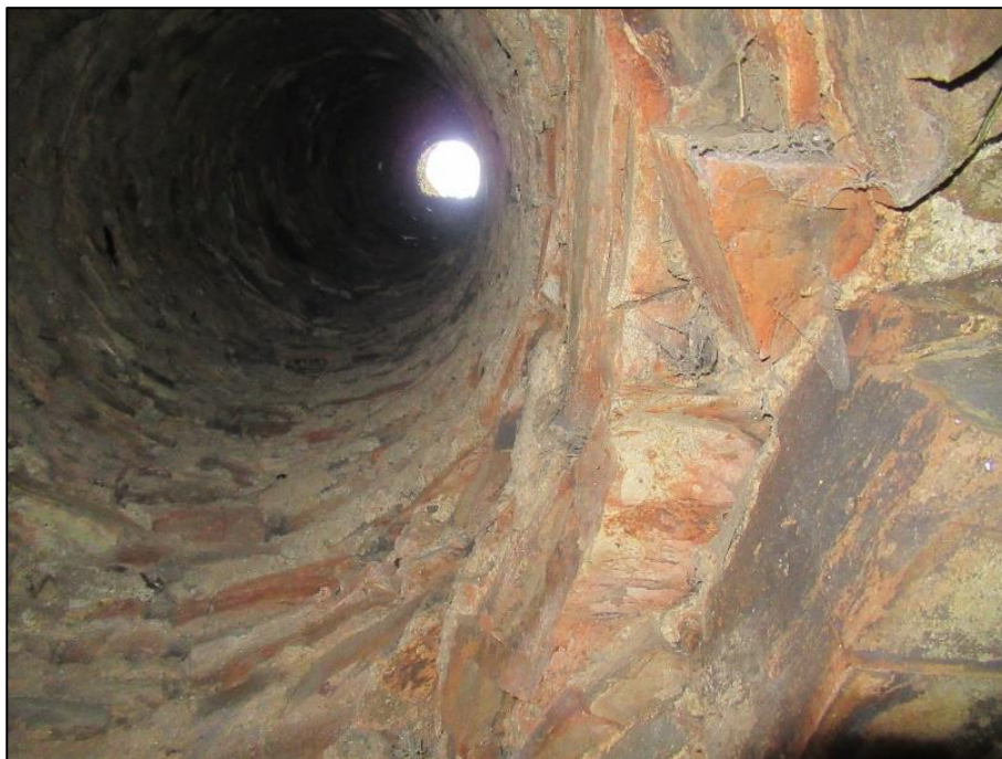
Figure 25.03 – Chimney internal showing condition and high-level vegetation
