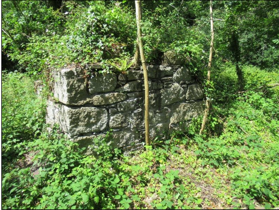
Figure 23.13 – Plinth with vegetation
