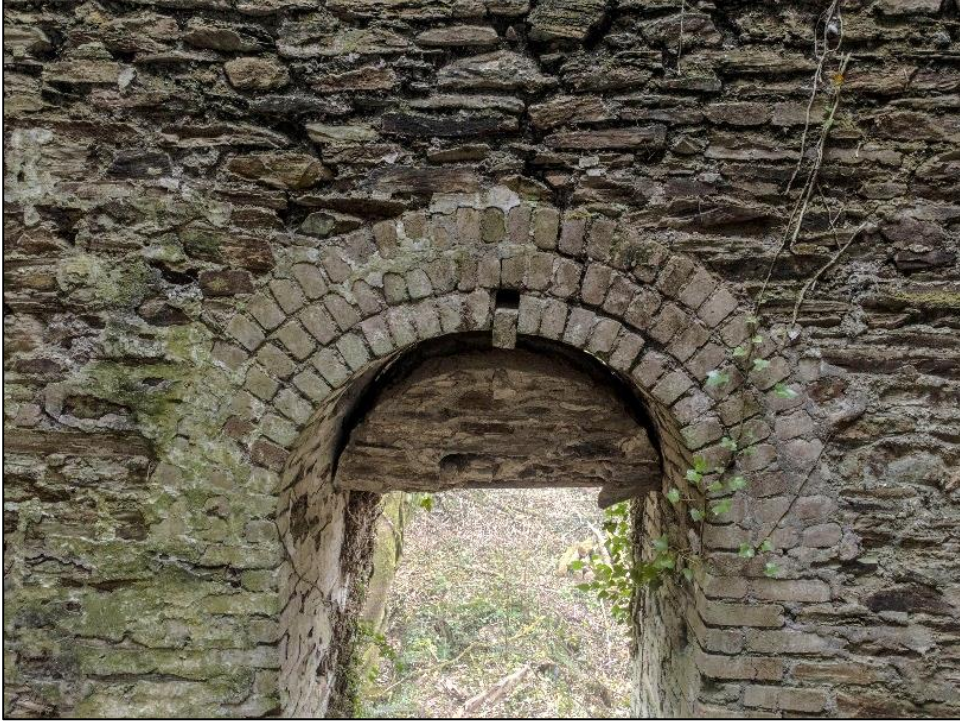
Figure 23.05 – Loose masonry local to arch crown
