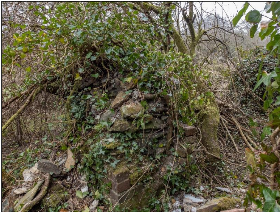
Figure 24.02 – Collapsed brick quoining and stonework with trees growing from wall head.
