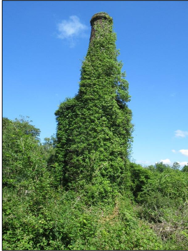
Figure 25.01 – Full length of chimney with heavy vegetation covering.
