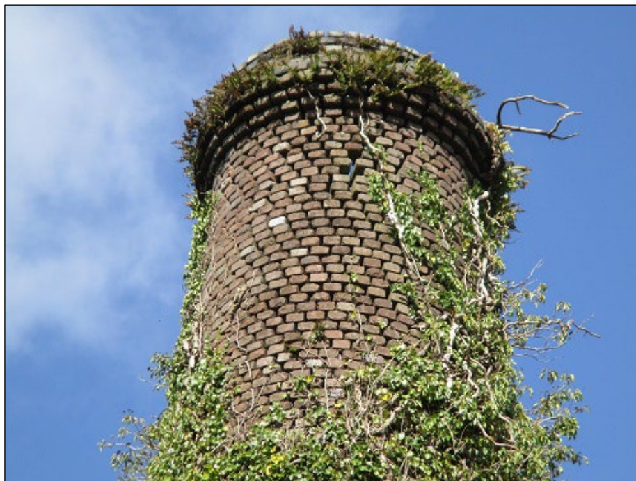
Photograph 20. Open jointed brickwork on the Boiler House Chimney brick capping course
