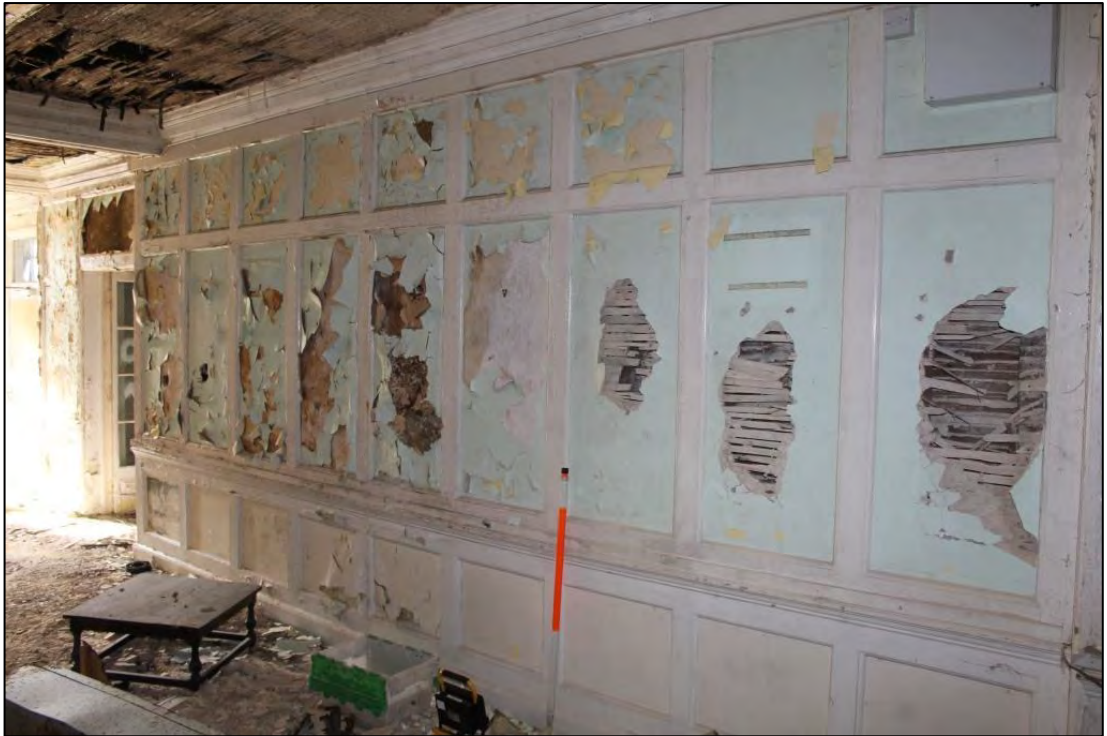
Photo 12: Detail of panels within Room 1, showing damaged portions
