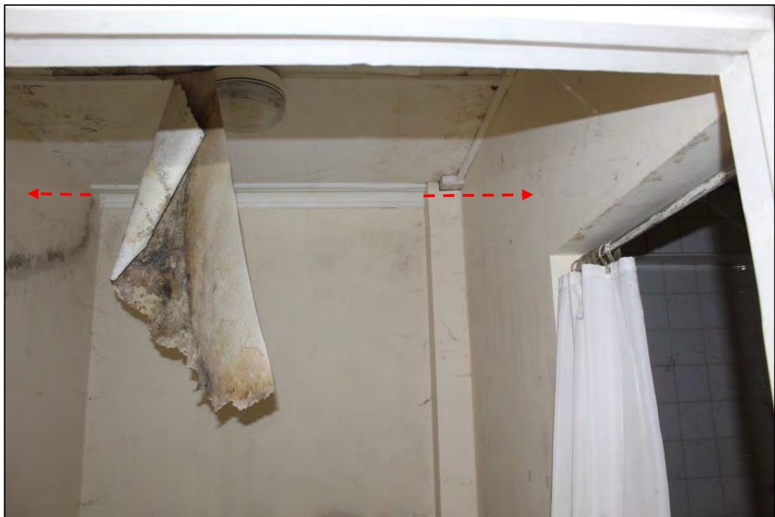
Photo 37: Detail of cornice remains within the WC of Room 42, looking north-west
