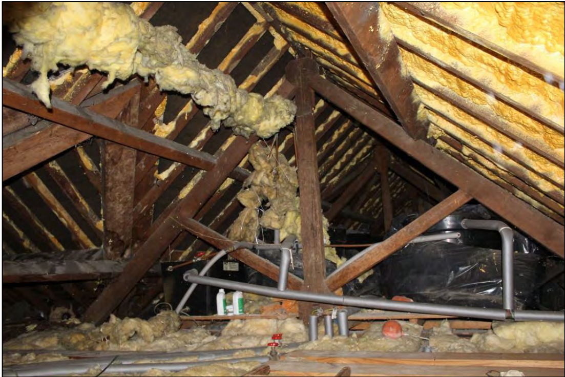
Photo 56: King-post roof trusses within roof space of Phase A, looking south from Room 47
