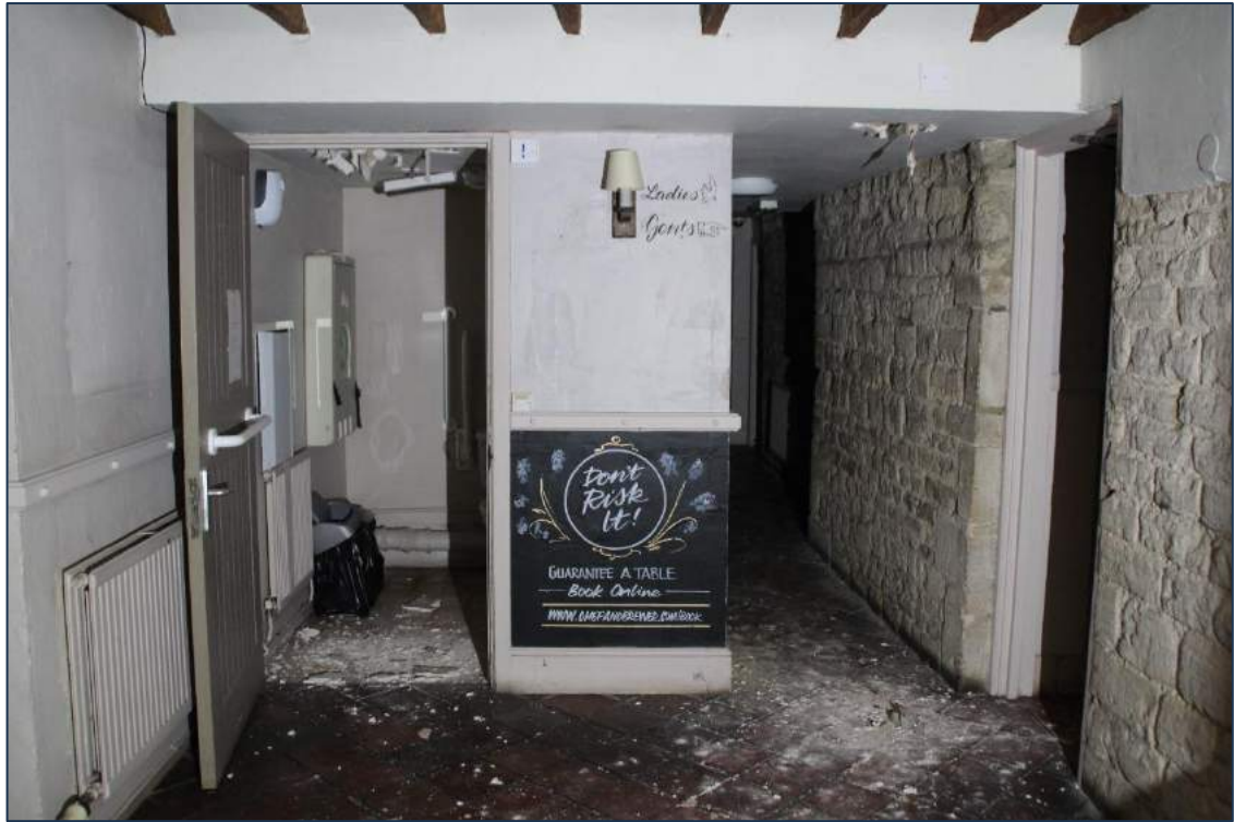
Photo 22 View looking west in Room 2 towards the ancillary spaces of the modern extensions
