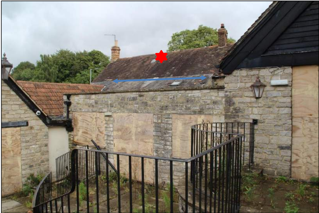
Photo 15 1980s/90s additions to the rear of the historic Building (starred) with the mid-20th century extension arrowed
