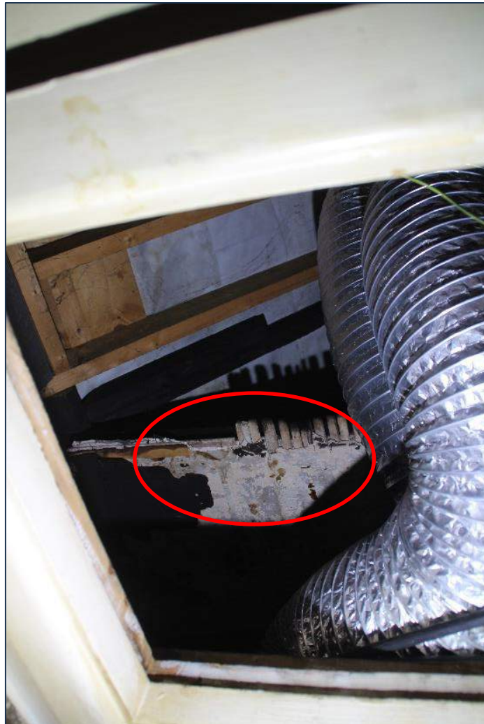
Photo 21 View of the roofspace of the kitchen with remnant lathe and plaster
