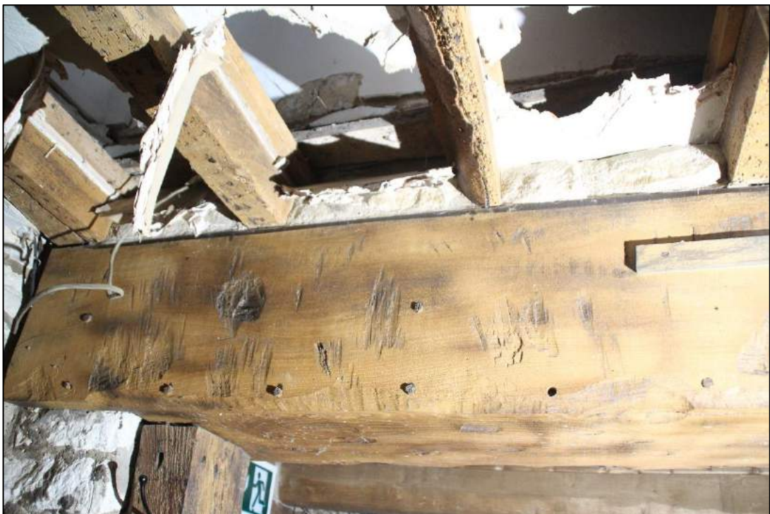
Photo 32 Detail of the modern central beam to Room 3 with replaced joists above
