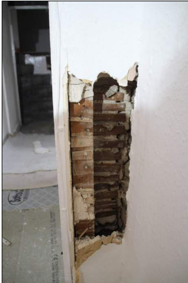
Photo 63 Remains of lathe and plaster in corridor
