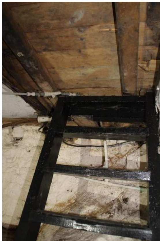
Photo 69 The underside of the ground floor surface, showing what appear to be historic timber floorboards and joist
