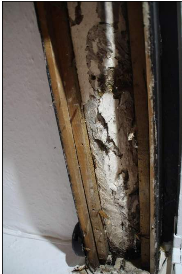
Photo 62 An historic timber beam in poor condition ‘sandwiched’ by modern timbers
