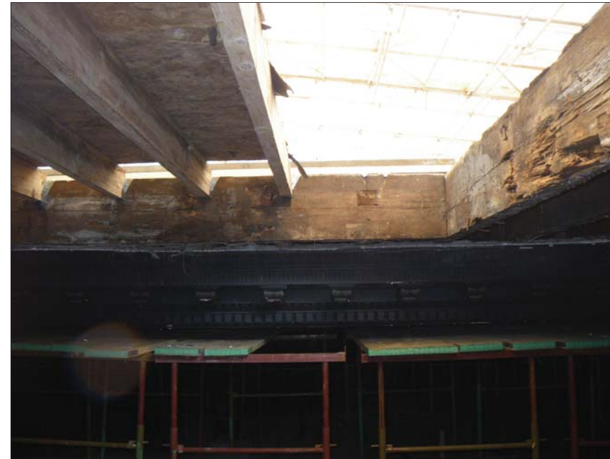
23 The raised ceiling section were the rose was. New joists to left, frame to raised section, rear and right
