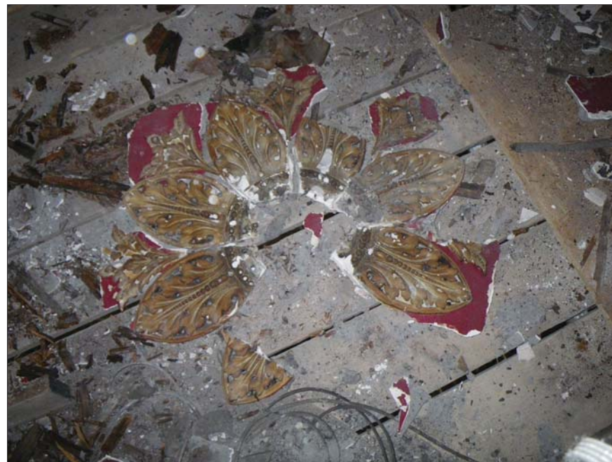
18 The centre of the section of the rose in cell F2 reassembled from falled fragments. The total diameter is c.0.76m
