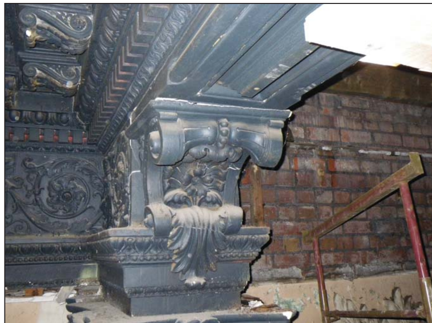
20 A preserved column-top console and its surviving beam soffit moulding in cell F2/G2. Contrast plasterwork on left and right
