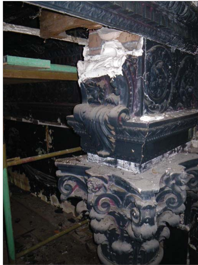
22 Typical damage to column-top consoles caused by insertion of crash decking
