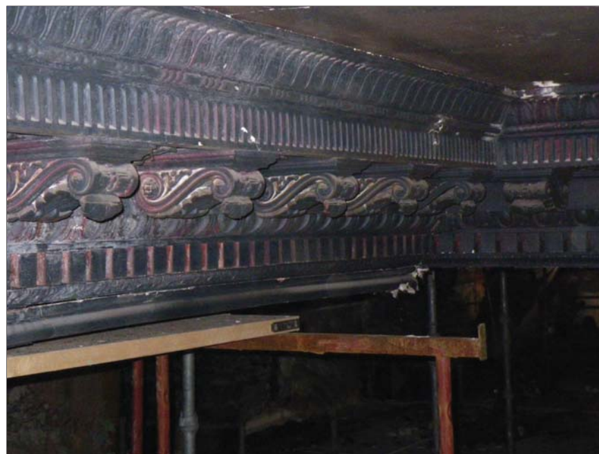
11 Typical length of plasterwork on ceiling beams. Note red paint shadowing. Cell D2, looking south-west
