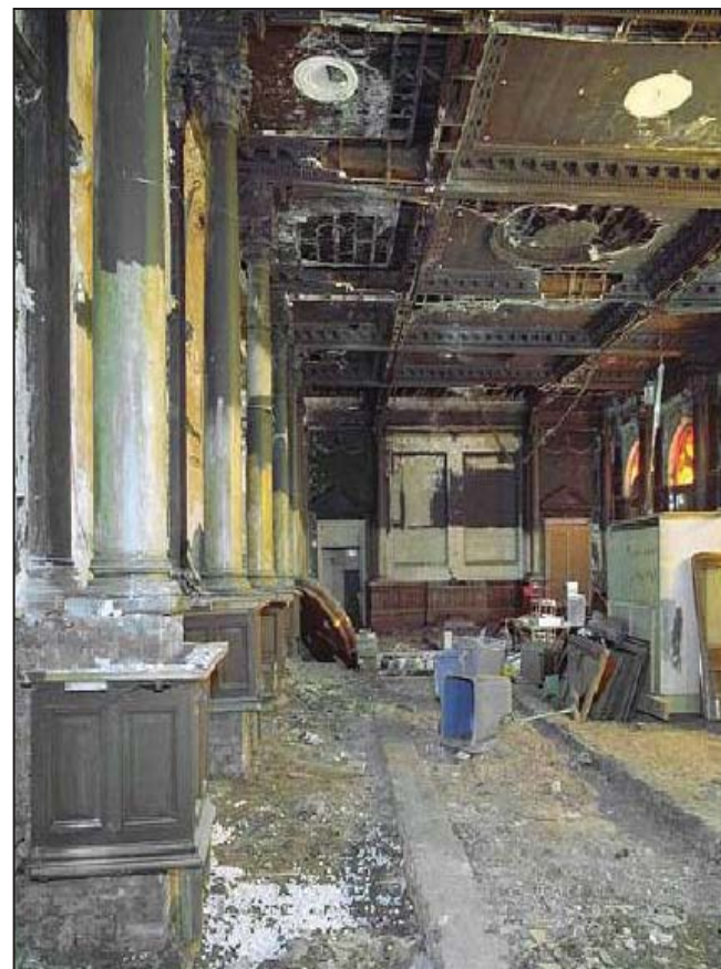
5 The interior just before the erection of the internal scaffolding in early 2010, looking south
