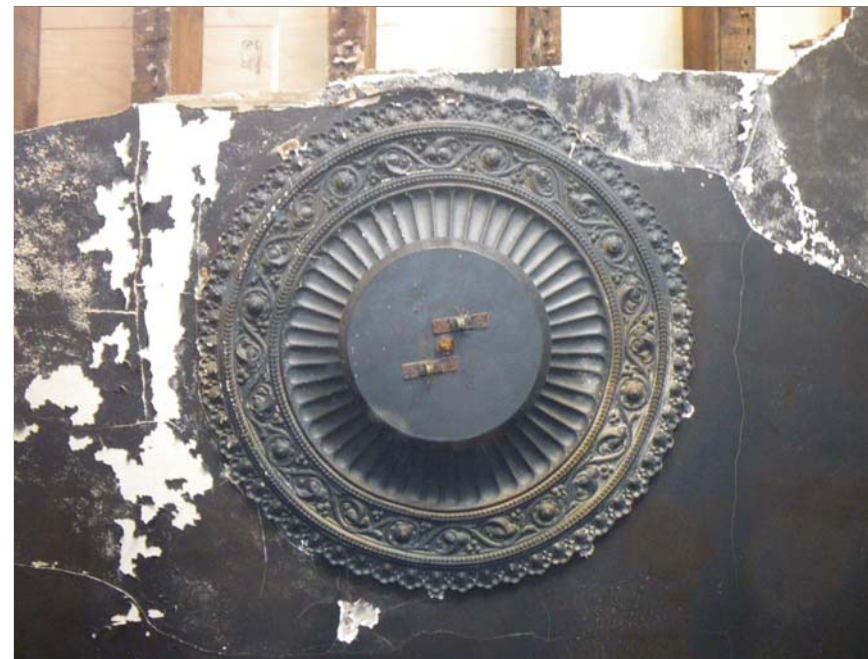
19 One of the smaller roses, 0.97m diameter. The boss is covered by a modern light fitting
