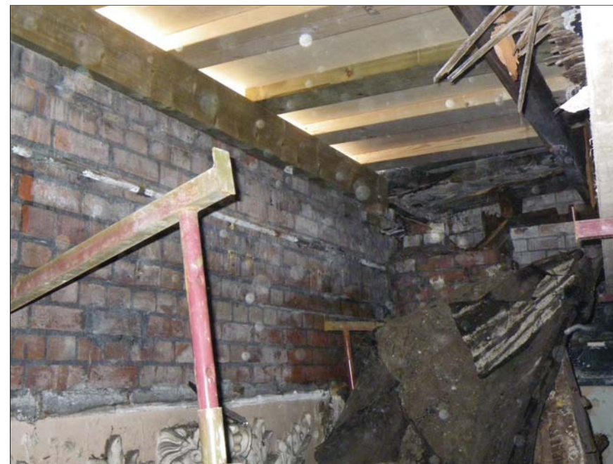
24 The southern end of the building where the plasterwork is most damaged or, indeed, missing. Cell G1, looking south-east
