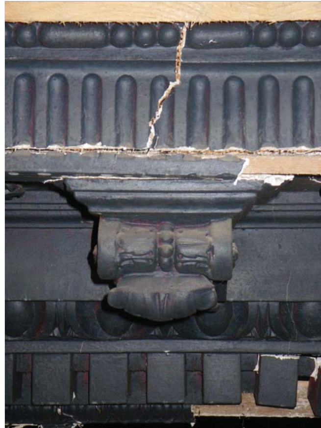
13 Detail of end of console bracket on ceiling beam (note prefabricated elements parting at joints)
