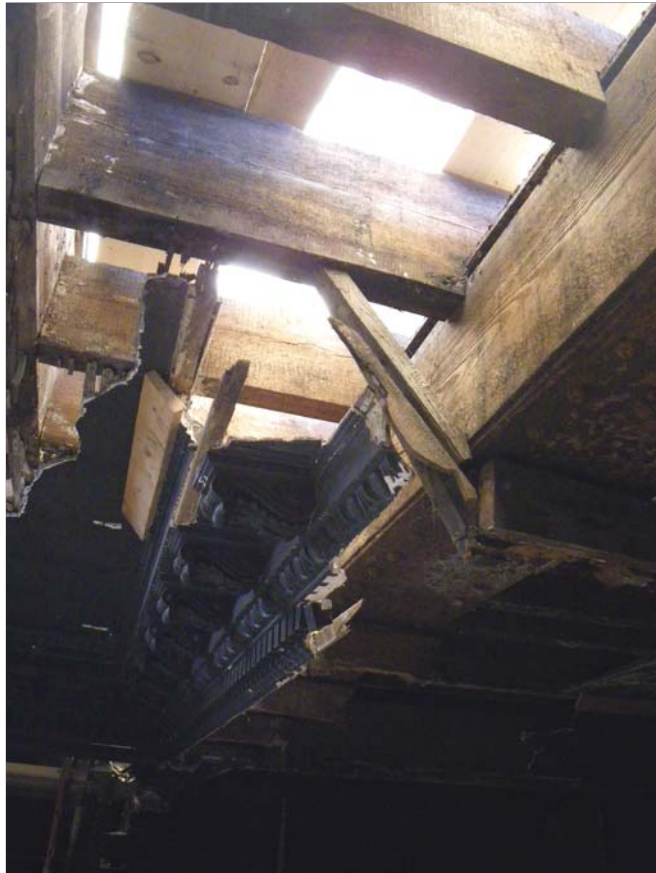
9 Main roof beam on south side of Cell D2 showing timbers of raised central section on left and attachment of plasterwork, looking east
