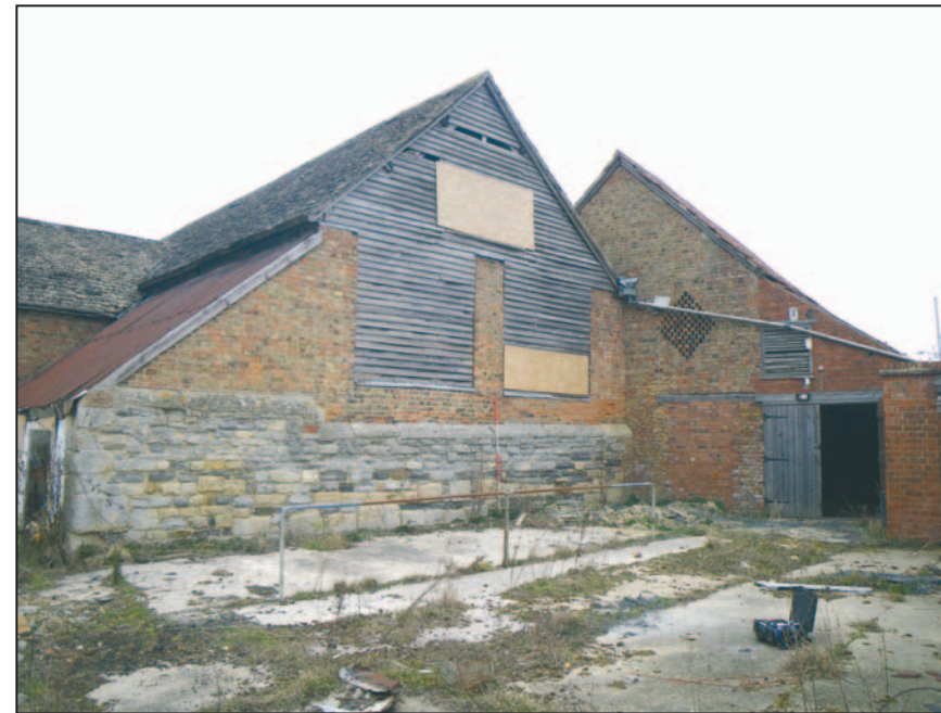
11 South-east elevation of Building 1 and south elevation of Building 2, looking north-west. Scale 2m.
