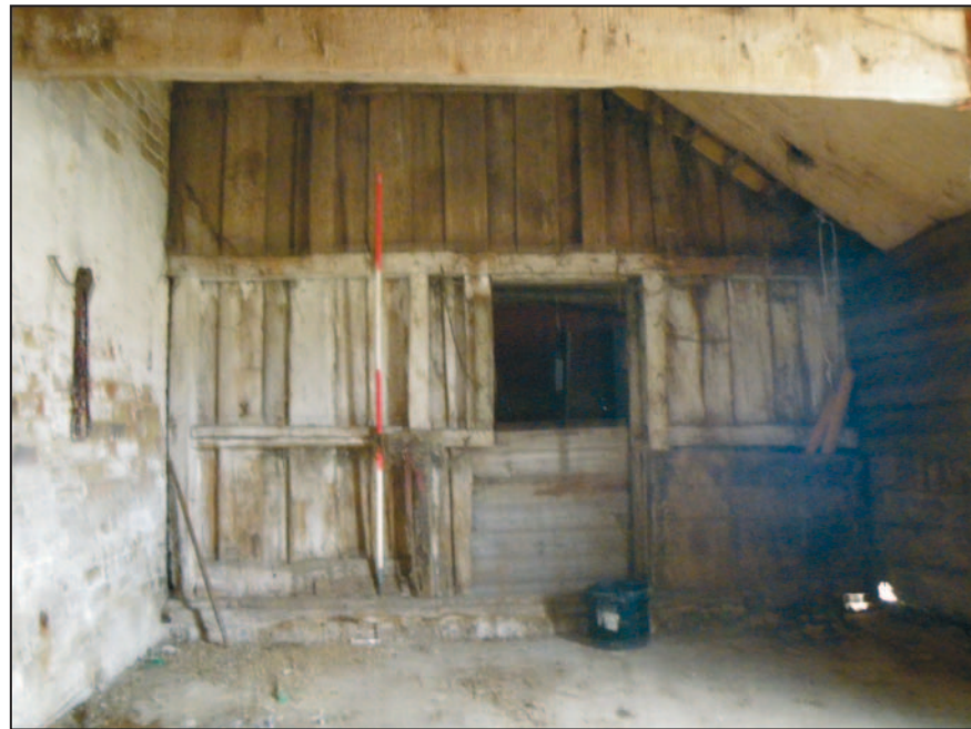
25 The south wall of the lean-to along the east side of Building 3, looking west from within Room 5. Scale 2m.
