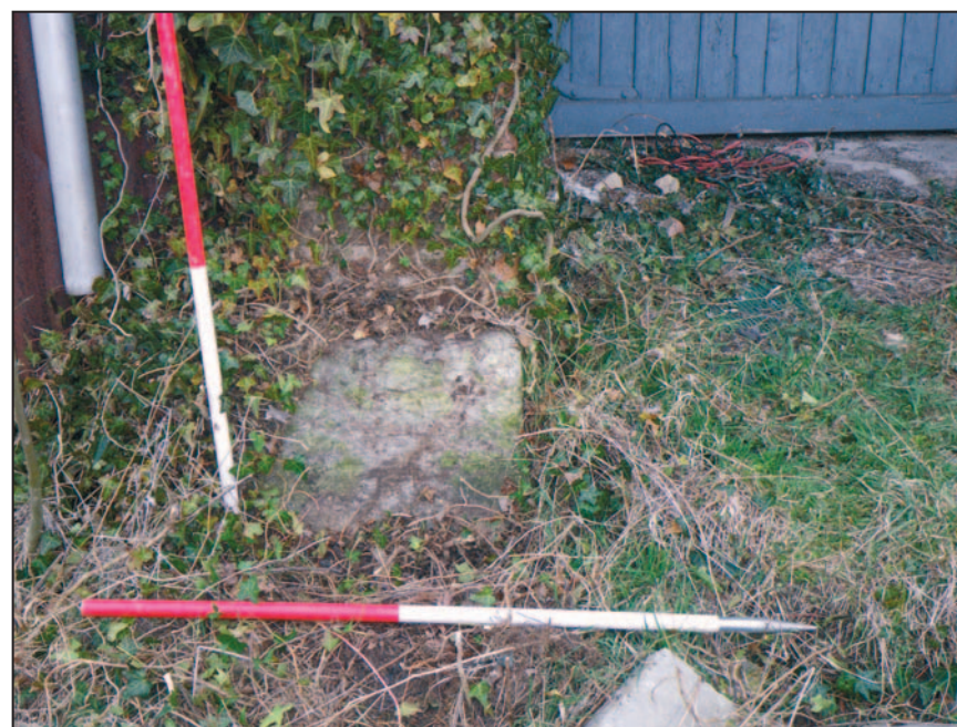
9 Stone block under end of west porch wall of south porch, Building 1, looking north. Scales 1m.
