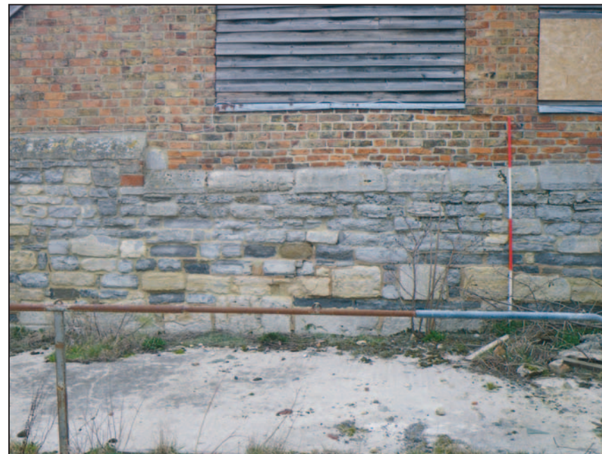
12 Detail of old bricks in south east gable end of Building 1. Scale 2m.
