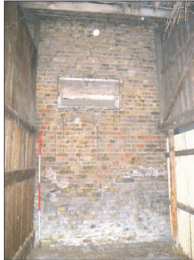
26 The east wall of Building 2 at the north end, inside one of the loose boxes. Scale 2m.
