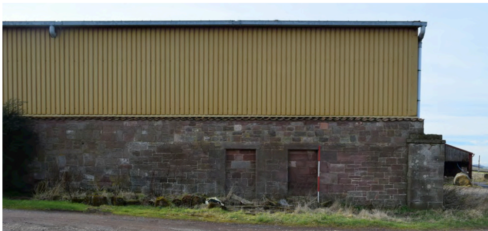
Plate 1: View of the east exterior elevation of Yard 2 – with two blocked entries; pier; pantile coped wall and the corrugated barn structure. Note also the differential masonry sections.
