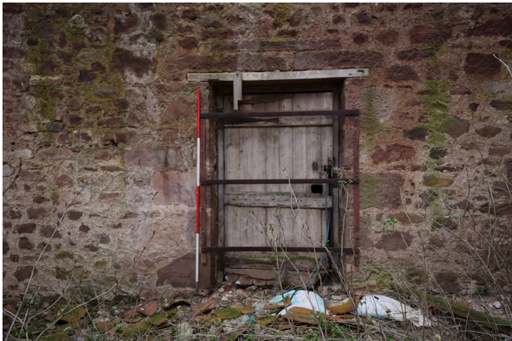
Plate 7: Detail of original door within the north portion of west range of Yard 2.
