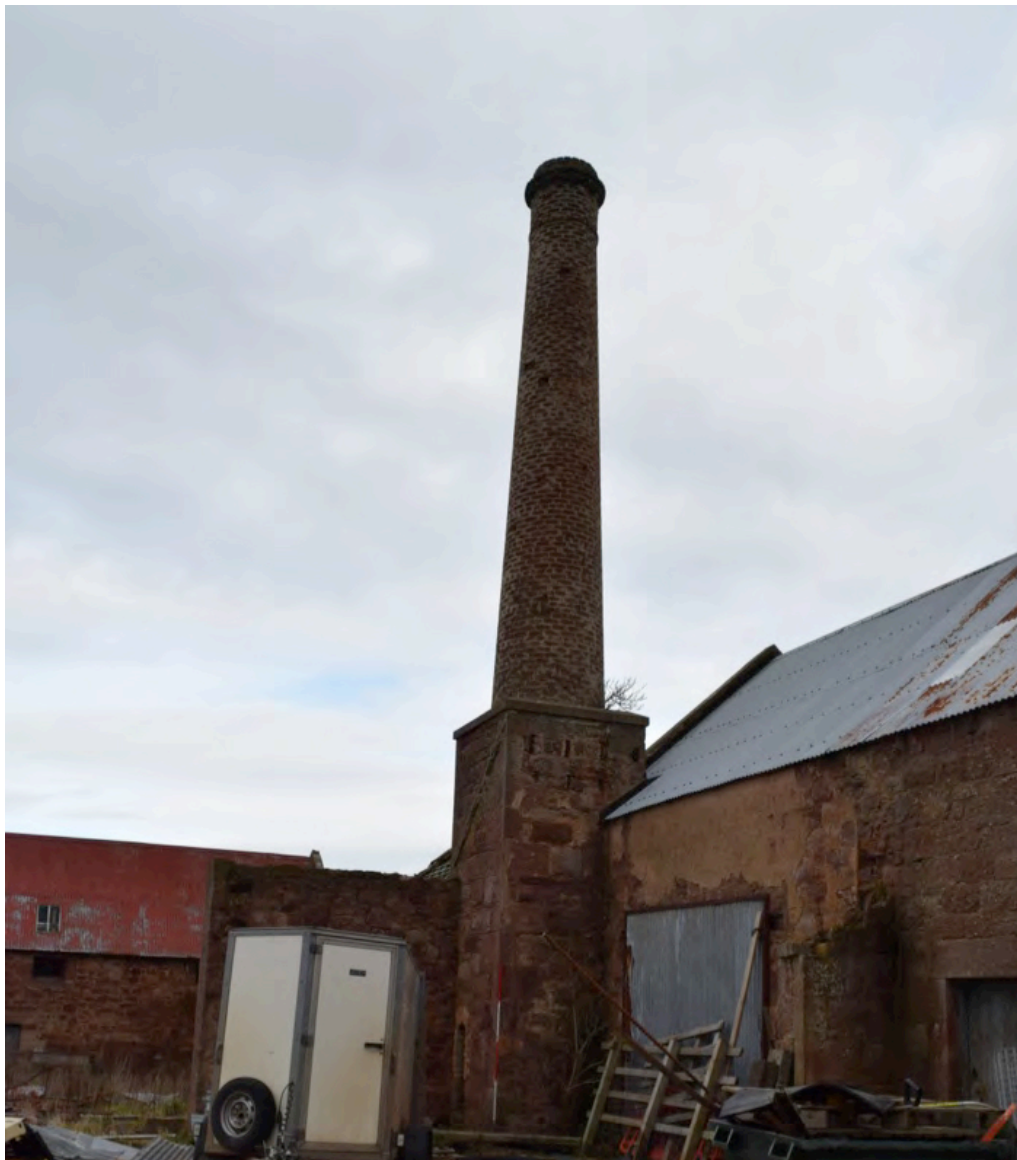
Plate 8: View of chimney stack, with raggle line scar on its west face and joist holes on its south face.
