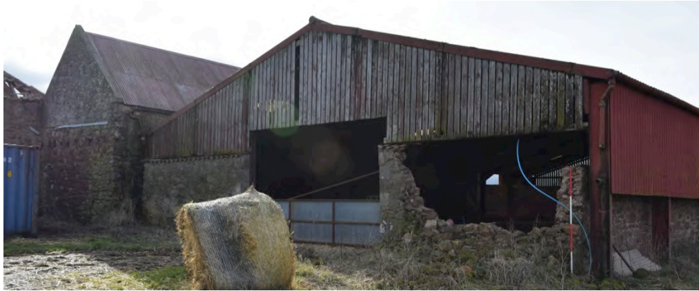
Plate 3: View of the east and partial north elevation of Yard 1– with flashing and joist holes in gable end of south range, wall stump and metal girder superstructure over the cattle court.
