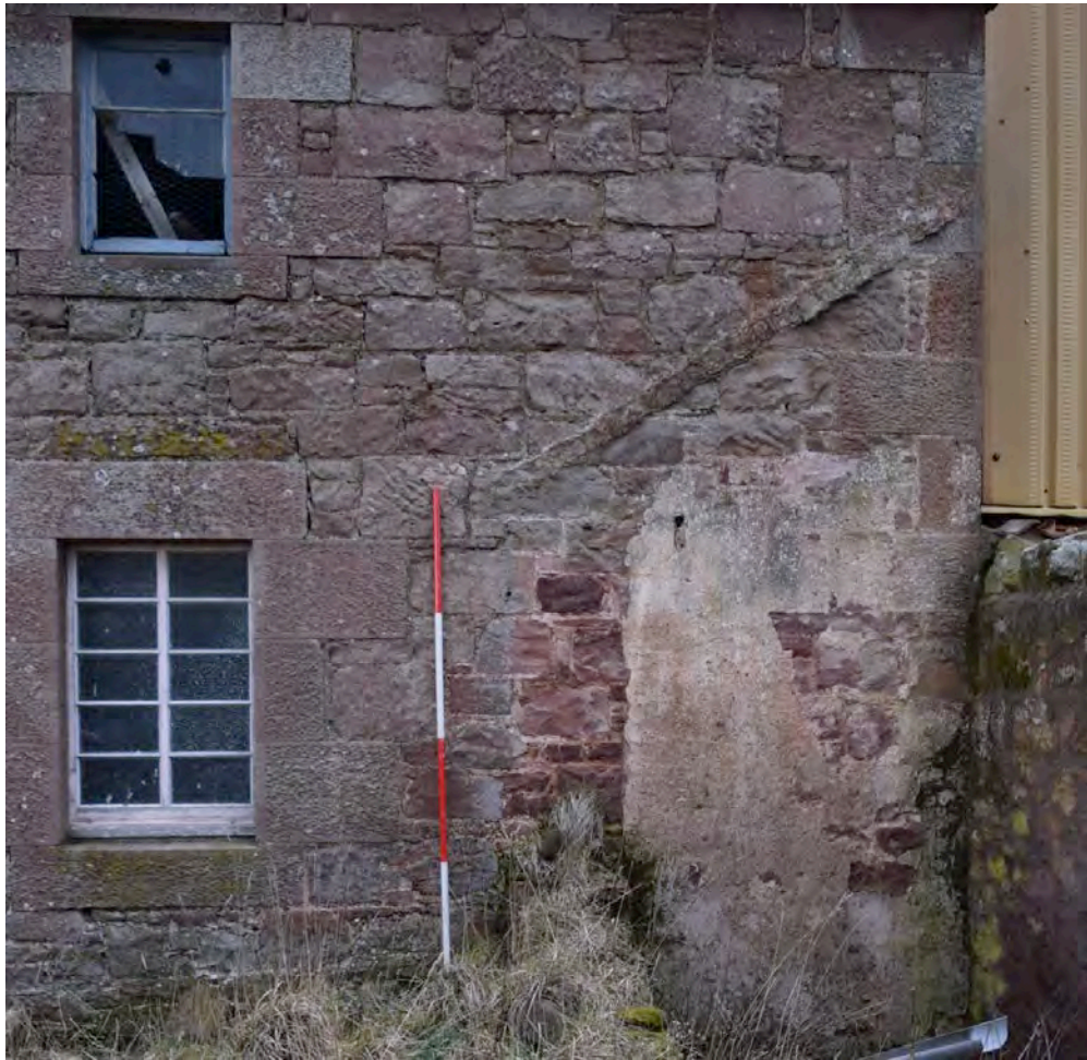
Plate 9: Yard 2; south range—detail of raggle line scar of a former pitched roof and wall scar visible on the same façade; note also turf covered wall stump extending from the façade towards south.
