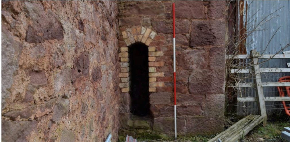
Plate 8: Yard 2; west range– detail of fire hole within the base of the chimney stack.
