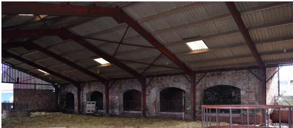
Plate 4: Yard 1– detail of five arched cart openings set into the south range. Note also the modern metal girder superstructure.
