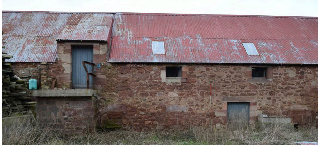
Plate 5: Yard 1; South range– detail of south exterior elevation with blocked ground floor windows, ground floor entrance, upper floor windows and cat-slide dormer door.
