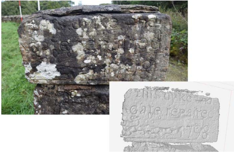
Plate 18: Inscription on the stone inserted into the eastern gate pier; "This dyke and gate was repaired 1798".
