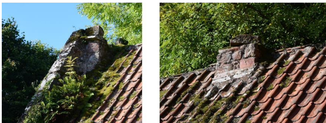
Plate 13: Roof and chimney stack [044] of Structure 4 (left) and Structure 5 [045] (right); note the drip stone on the chimney [044] and the depth of the gable.
