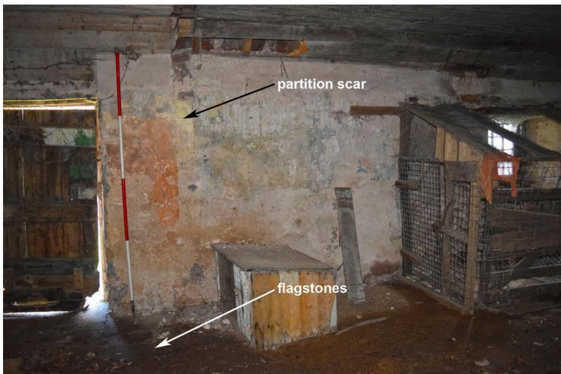
Plate 20: Partial E elevation of Room 5.1, with differential paint scheme and marks and scarring from the former wall partitions visible on the elevation and the ceiling.
