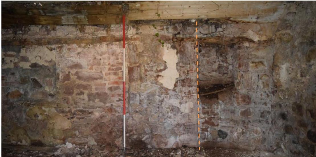
Plate 18: Partial W elevation of Room 5.1, with partial blocked opening [020] on the left and niche [021] to right; also note the former end of the W wall (dotted orange line), marked by quoins later reused as southern jambs of opening/recess [021].
