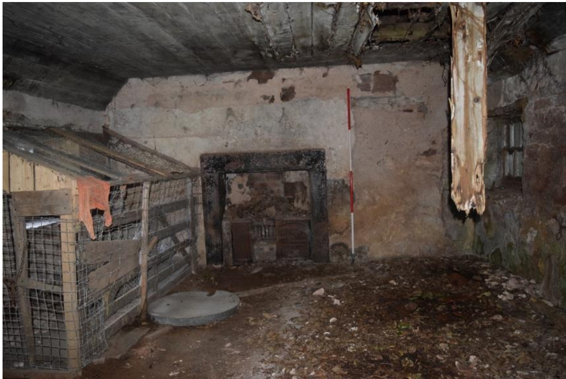
Plate 16: S elevation of Room 5.1, with fireplace/range [018] and blocked former entrance [017] to the left; also note the coved ceiling and cage construction in the corner.
