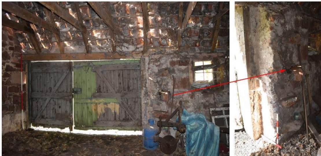
Plate 40: W elevation of Room 3.1, with large entrance [012] and small window [013] (left); tasking stones N of the entrance [012] (right).
