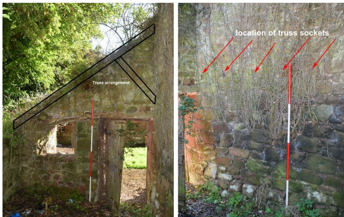
Plate 21: E elevation of Room 6.1, with entrance [006] and window [007] (left); S elevation with line of sockets for former roof trusses (right).
