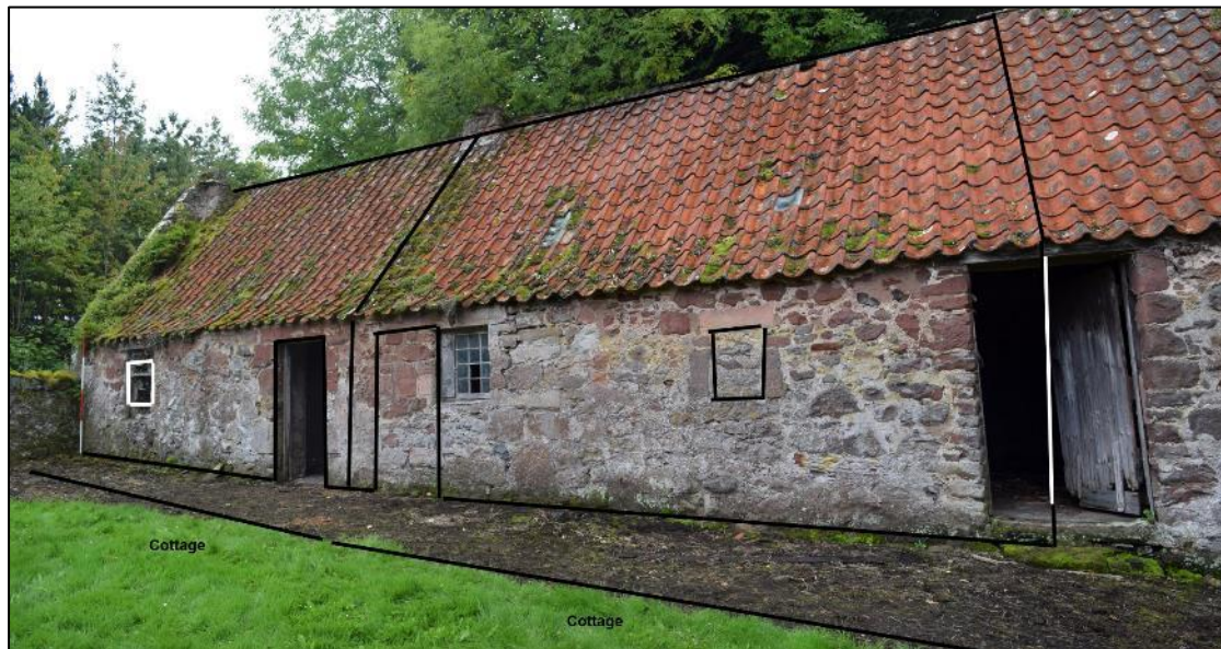
Plate 43: View to SW, showing the original formerly thatched cottage (Structure 4) to left; with abutting Structure 5 to right. Conjectural double hinds' cottage marked with black lines.
