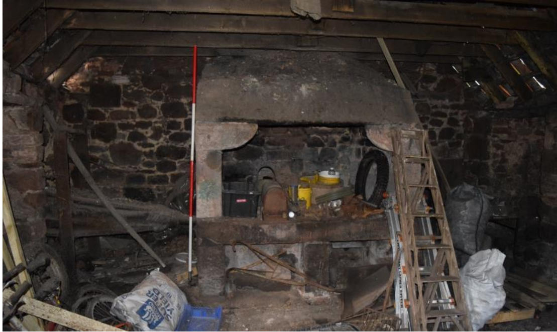
Plate 36: Room 2.1, N elevation with massive lugged hooded forge and bellows to left.
