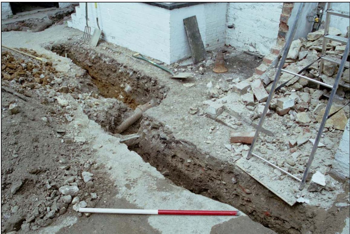
Plate 4: General view of completed foundation trench for new 'sun room' - looking north-west
