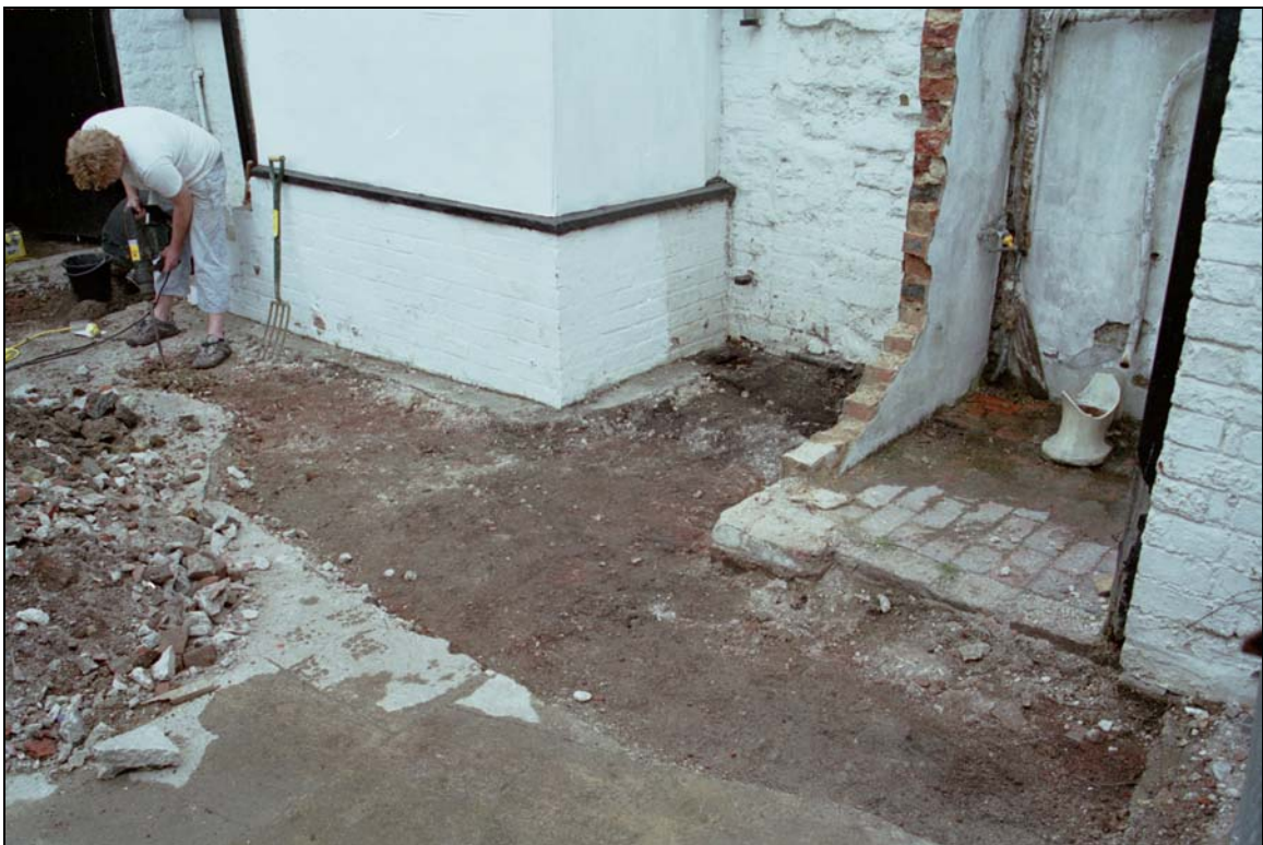
Plate 2: General view of site for new 'sun room', following localised removal of concrete yard surface & partial demolition of existing outside toilet - looking north-west
