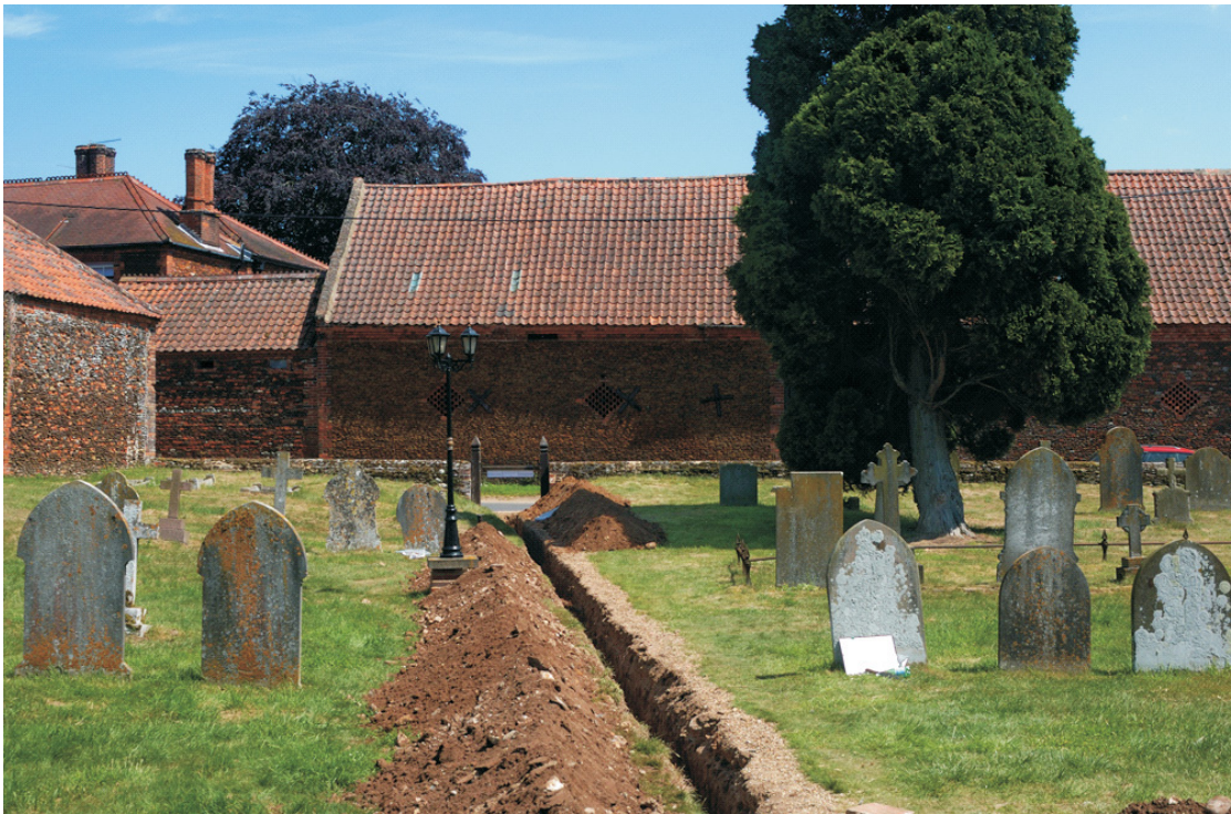
Figure 2. Location of gas pipeline trench (above) and photograph looking east along the trench (below)
