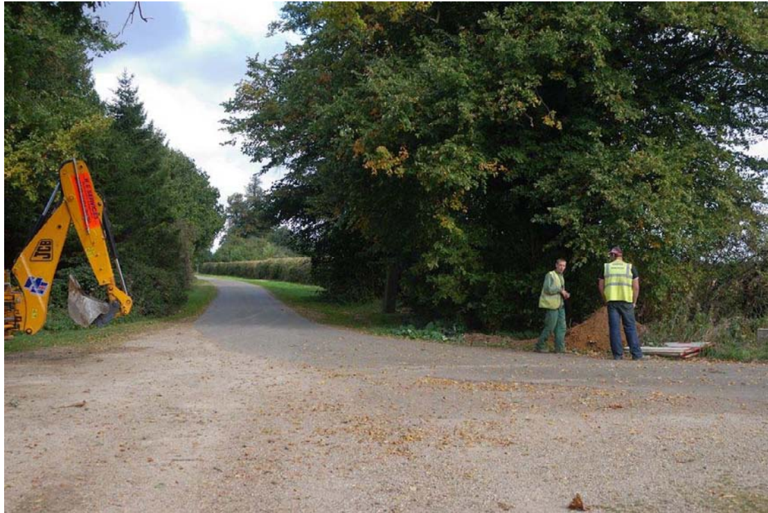
Figure 5. Starting point of pipeline adjacent to the Estate trackway and Depot showing TP 1 to the north (by workmen)
