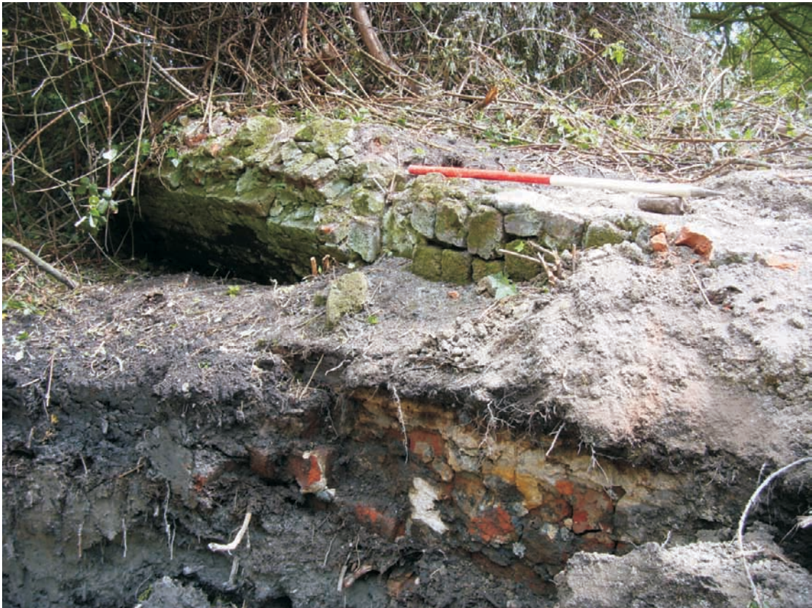
Figure 6. The collapsed moat wall F.4
