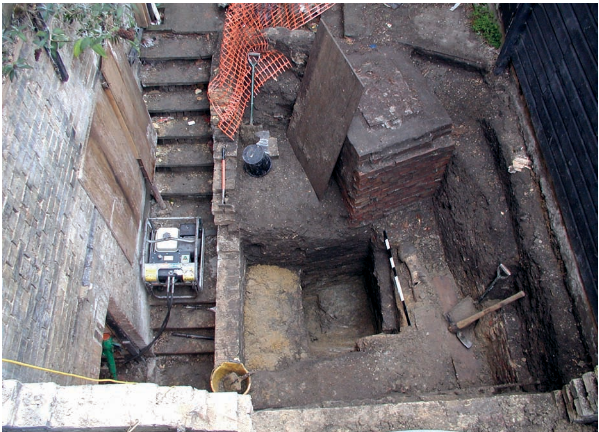
Figure 7. General views of Area 1. Top: vertical shot of area after initial excavation, facing northwest. Bottom: shot after excavation completed, facing southeast
