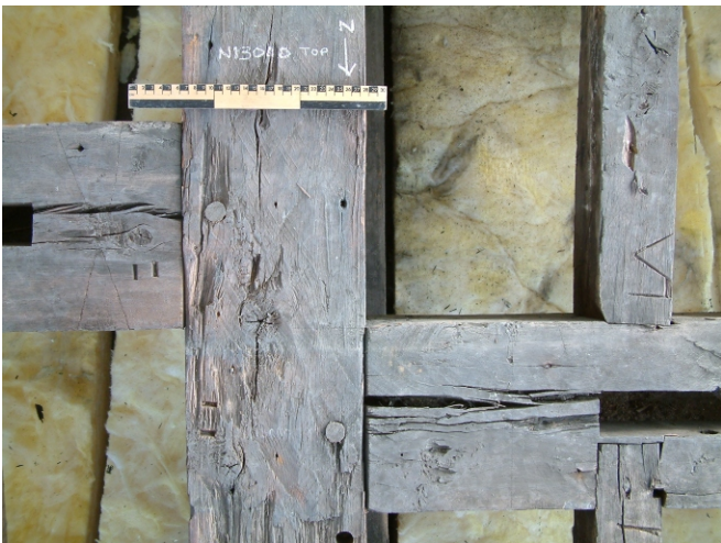
D: Marks where purlins P6 (rhs) and P7 (lhs) meet principal rafter PR6
