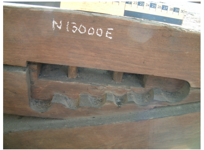
D: Empty mortice in PR6 showing moulding, slot for tenon and pegs still in situ
