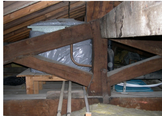
D: Master's Lodge truss showing metal strap at base and brackets securing the added block (6 th truss from tower end)
