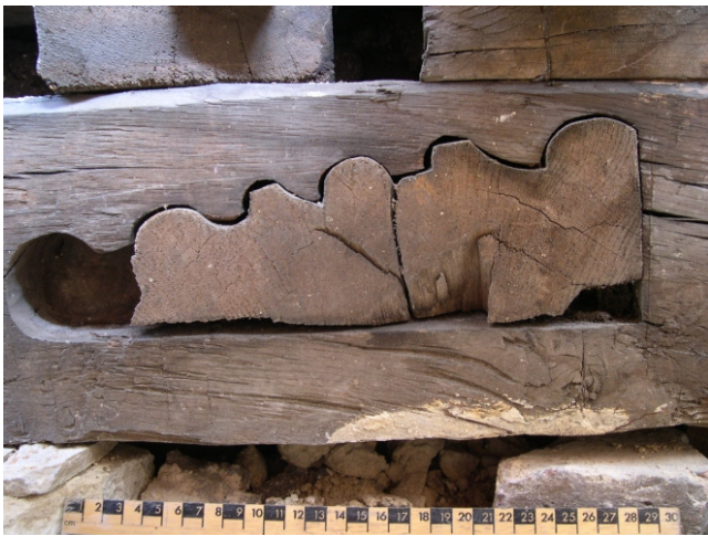
C: Sawn off remnant of moulded purlin in WP4
