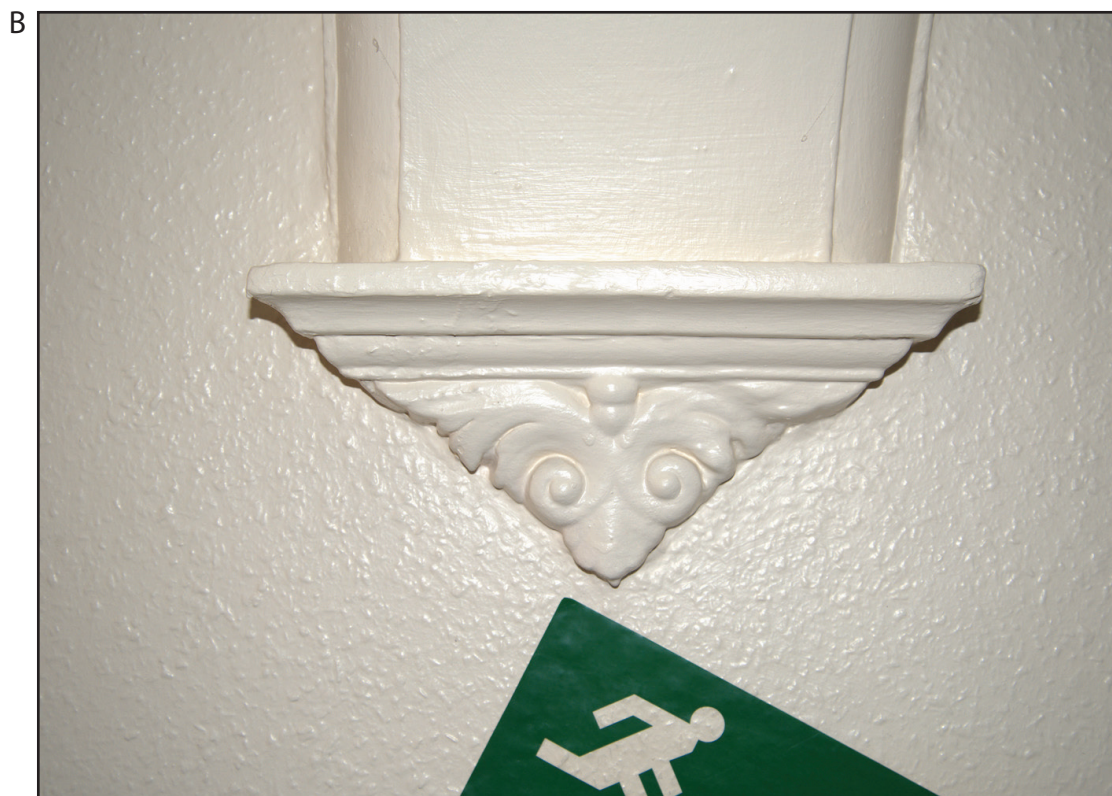
Figure 21. A supporting arch was present on the second storey of all eight properties. Here, the best preserved example is shown (A, from No. 5) with an inset detail of the decorated stop from No. 8 (B).
