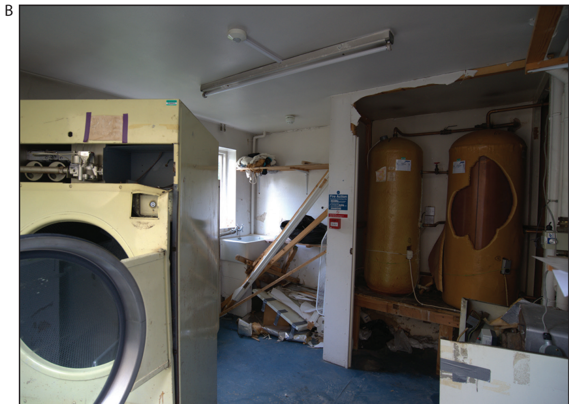
Figure 10. Views of the former kitchen (A) and former scullery (B) in No. 5
