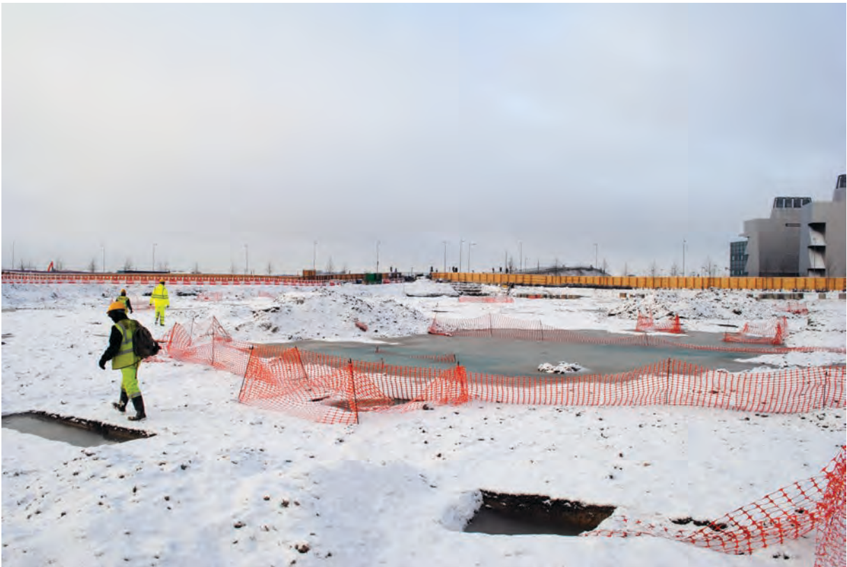
Figure 12. Aerial photograph of the North plot and view of flooding and snow during excavation
