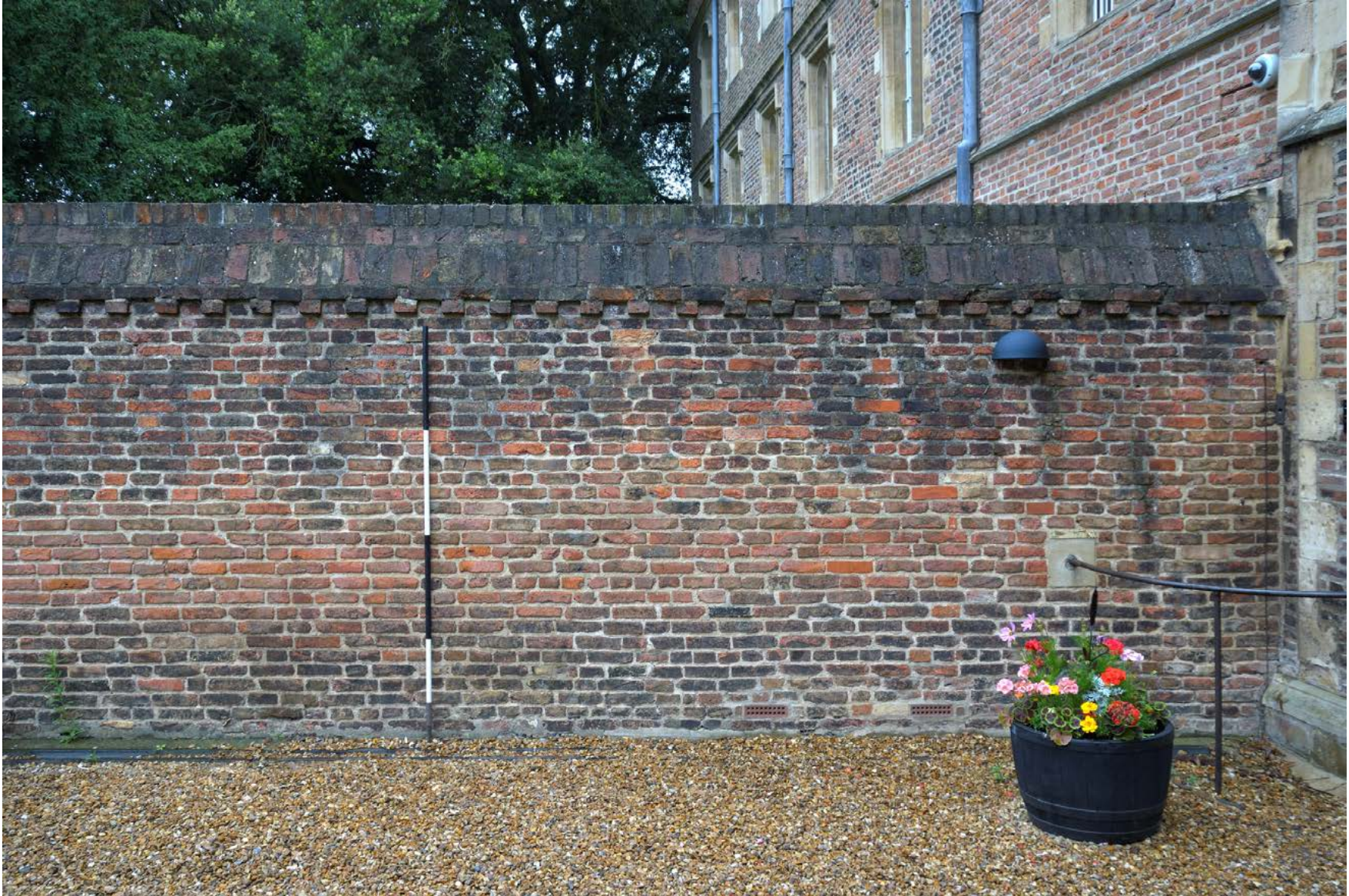
Figure 4. Section of Chimney wall into which a new doorway is to be cut, facing west
