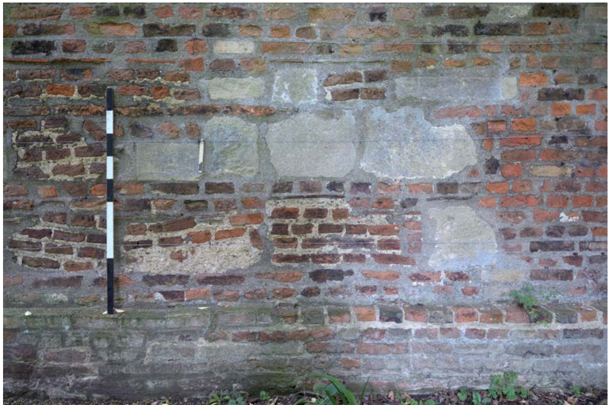
Figure 5. Elements of reused masonry incorporated into the rear elevation of the western Chimney wall (views facing east)
