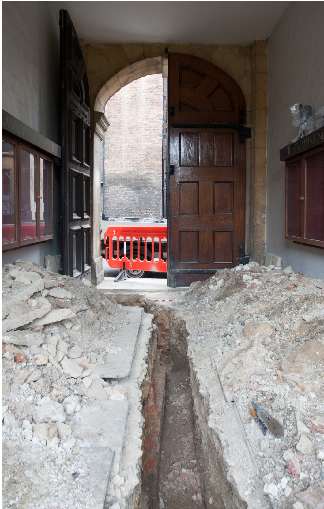
Figure 2. A view facing west along the passageway from Queen's Lane, showing early brick footing [101]
