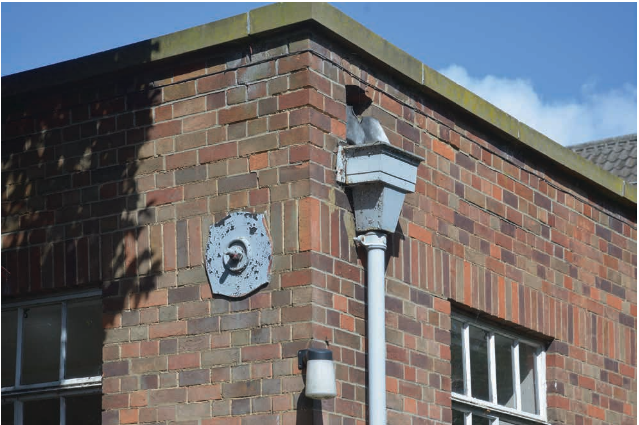
Figure 9. Exterior views of the library, from the rear (top) facing northwest and a detail showing a structural tie on the front façade (bottom) facing north
