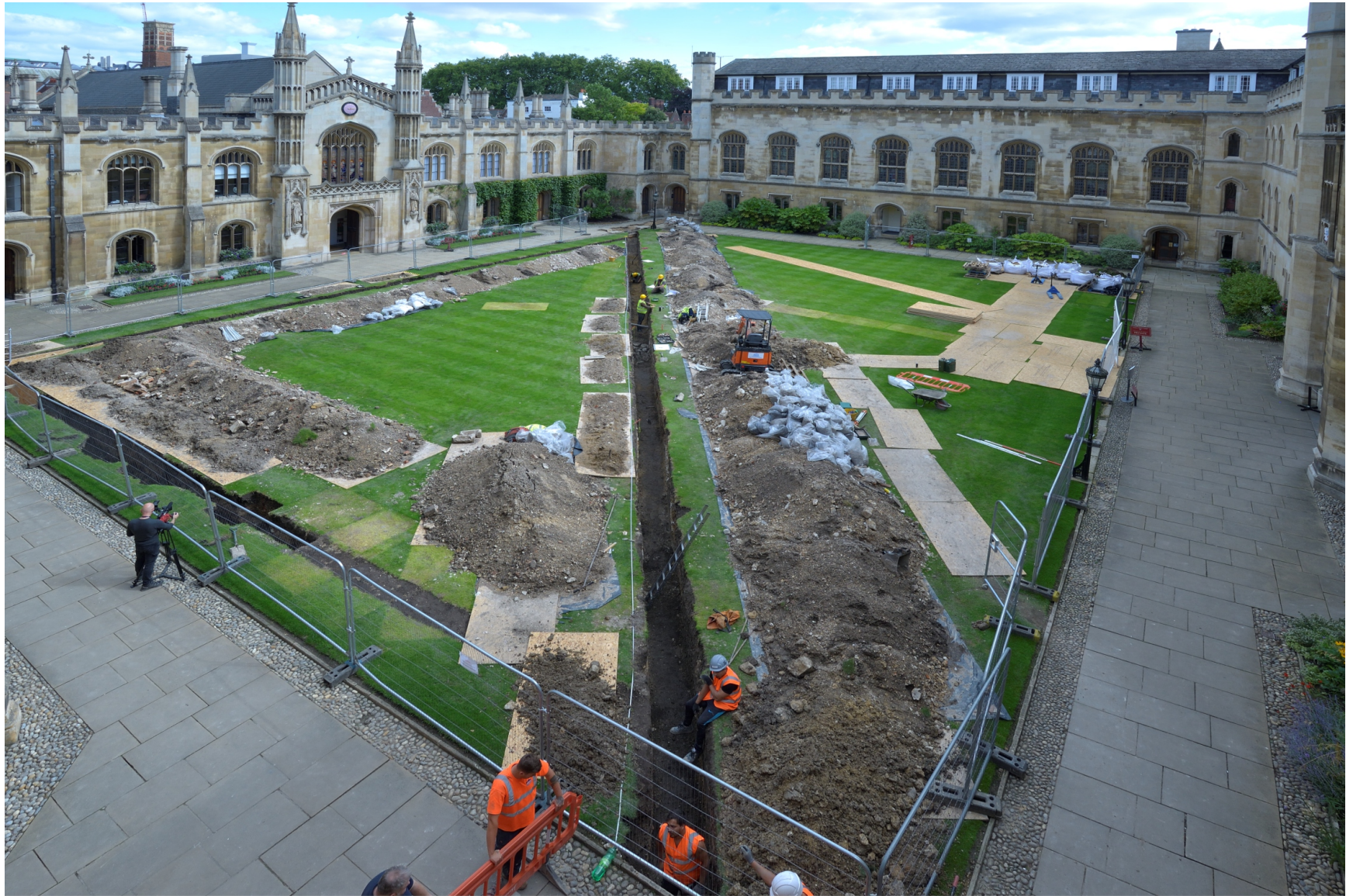
Figure 2. View across New Court, facing southeast, showing the extent of the trenching
