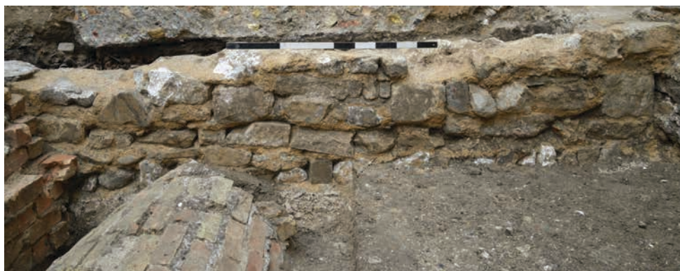
Figure 12. Photographs of the 1833 vestry, showing: top, wall footing F.02 in relation to the building's original doorway, now blocked (facing north, the roof scar pertains to the subsequent vestry of 1878); bottom, the elevation of footing F.02 (facing west)
