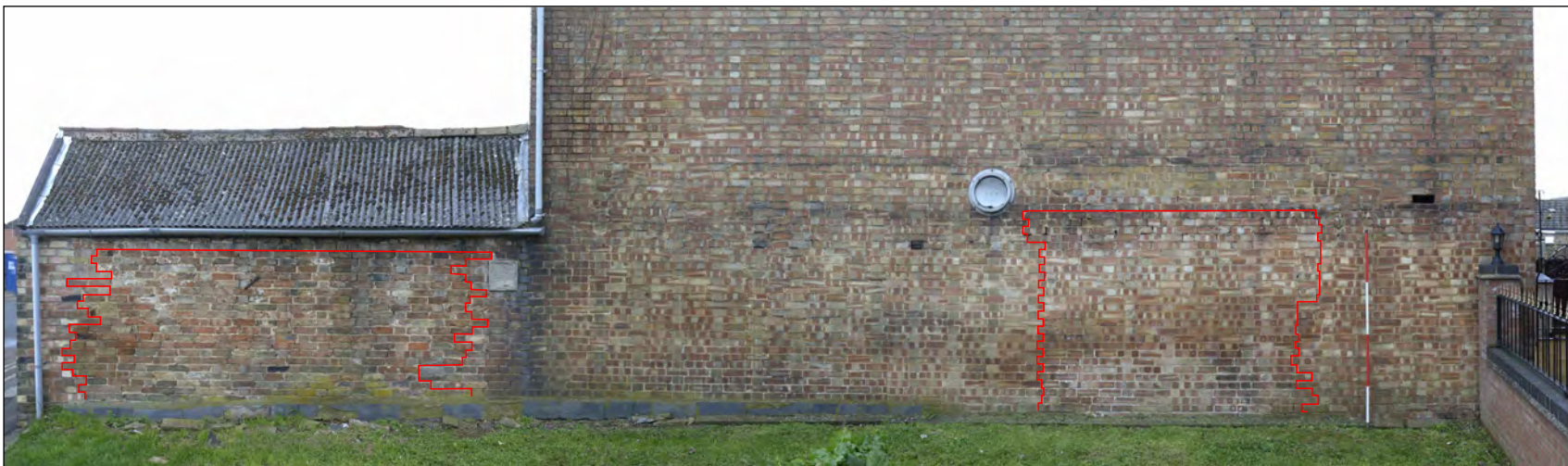
Figure 7: East elevation, lower image shows areas of older build (left) and rebuild (right). Composite image
