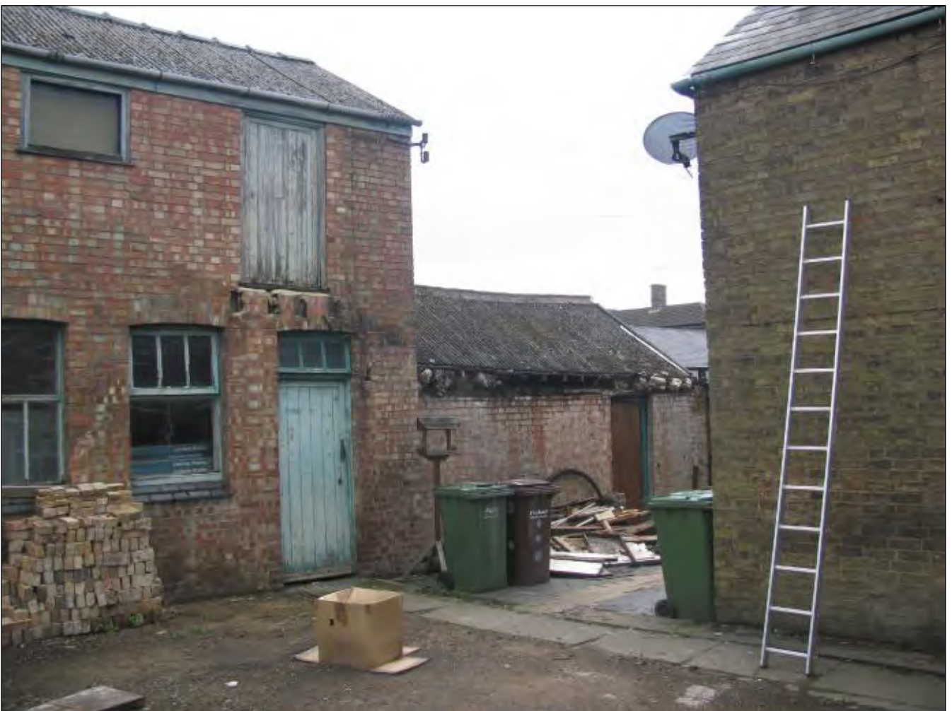
Figure 4: West face prior to restoration of adjacent cottage (from FOX-AD Design & Access Statement)
