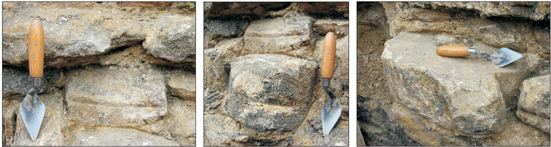
Figure 11. Section and photograph of walls within Thompson's Lane compound with reused Medieval masonry.
