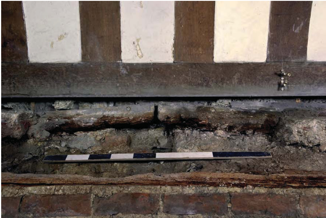
Figure 16: North wall of Fellow's Cloakroom (top) with detail of original sill beam, c.1500 (bottom).
