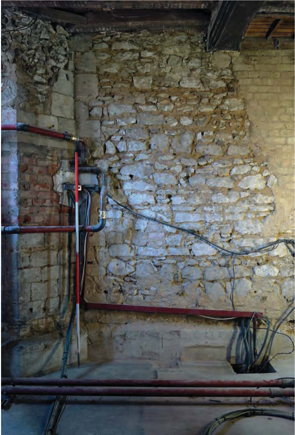
Figure 10: Elevation of south wall of Boiler Room, formerly the north wall of the chapel - not previously recorded.
