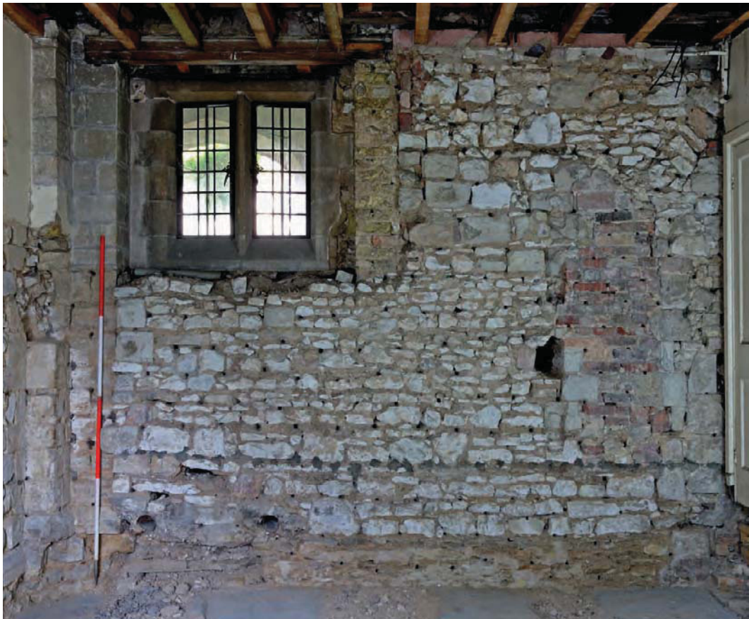
Figure 17: 1995 elevation drawing (top) and re-exposure (bottom) of west wall of Art Store - formerly the sacristy/vestry.
