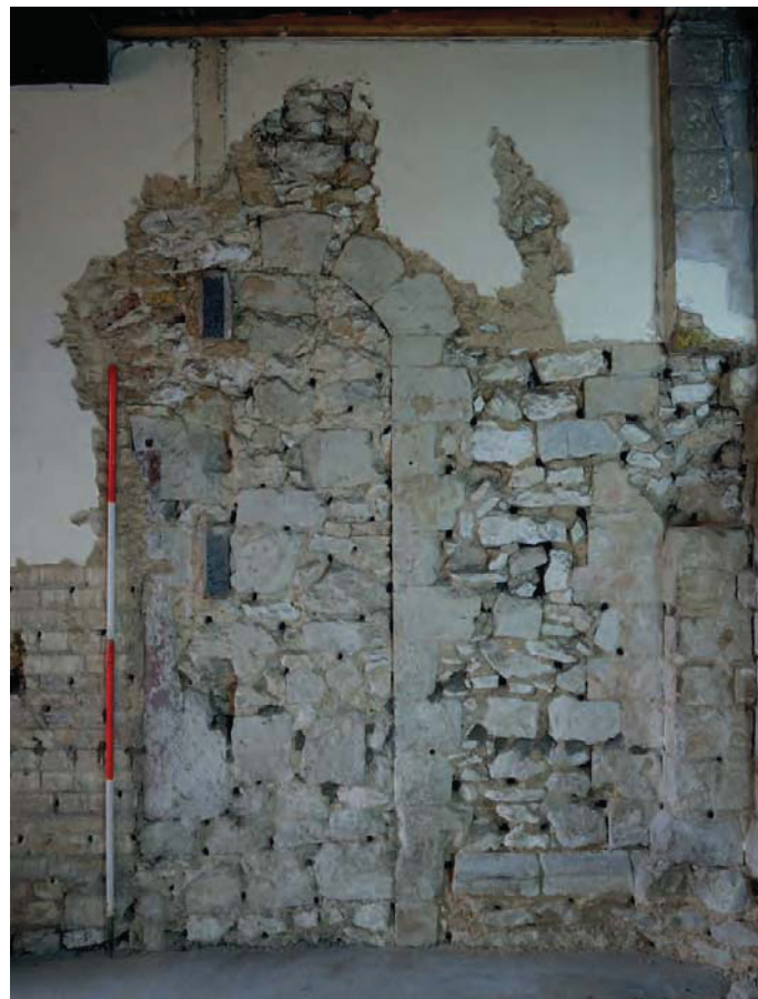
Figure 9: 1995 elevation drawing (top) and re-exposure (bottom) of south elevation of Art Store - formerly the north wall of the chapel.
