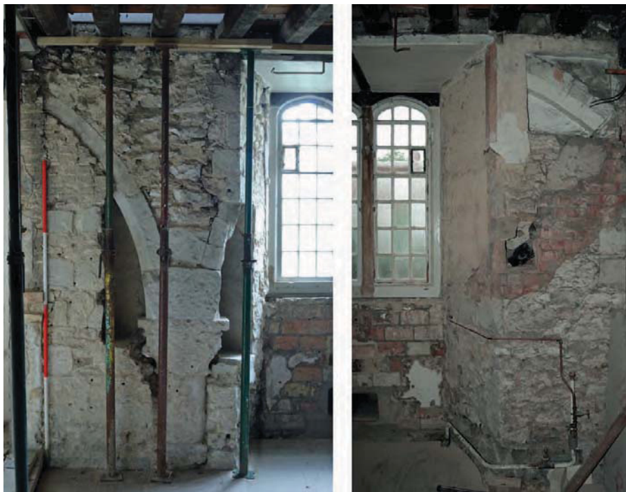
Figure 12: 1995 elevation (top) and re-exposure (bottom) of east wall of IT Store - formerly the chapter house.
