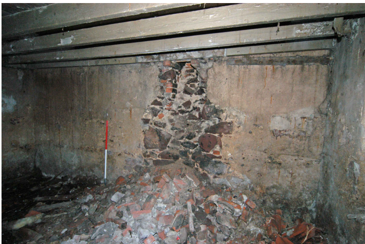
Plate 16: Building 3, Room 2 ground floor interior, east-facing wall, collapsed chimney
