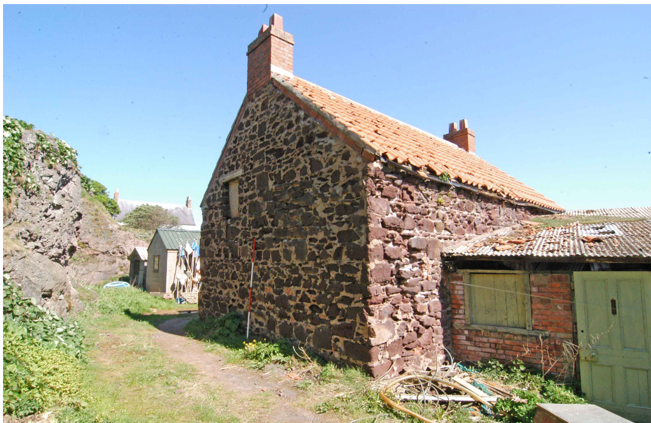
Plate 11: Building 3, Rosecroft Cottage, West-facing gable and part of the south-facing elevation with adjoining Building 4
