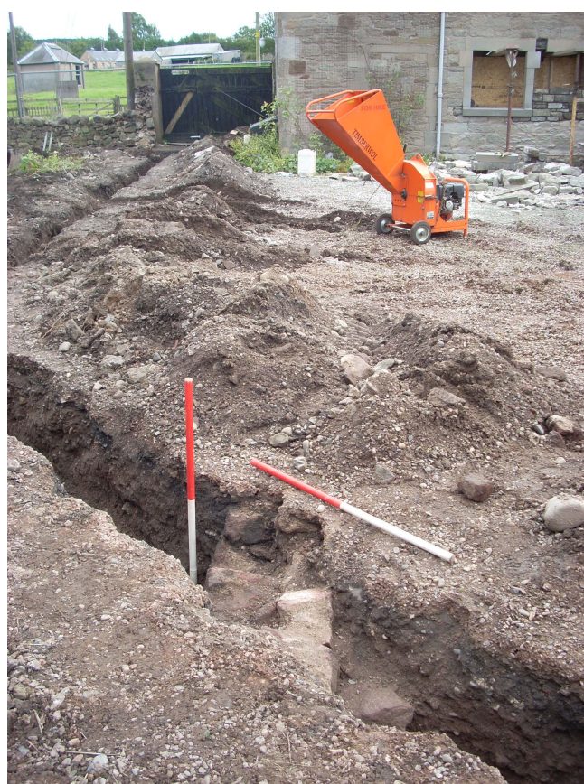
Fig.8 - Wall 017 exposed in the cable trench. This aligns with the eastern gable of Stonehouse Cottage in the background
