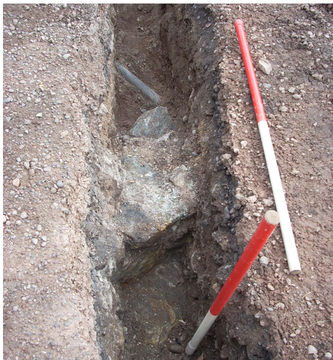
Fig.6 - Wall 008 exposed in the cable trench. The only wall made of a grey-blue schist
