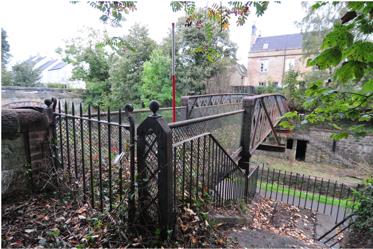
Plate 8 - Wrought iron gate and structural detail of the west end of the footbridge
