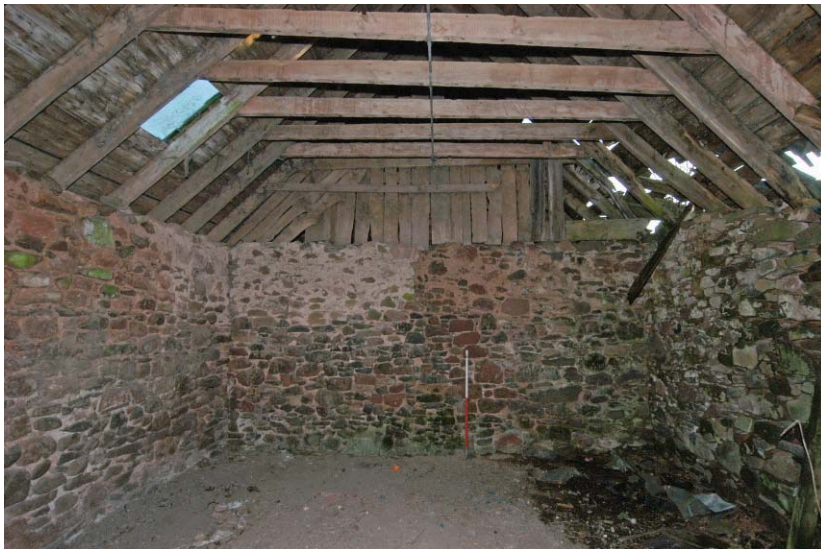
Plate 9 - A-frame roof joists resting on the wall heads and the partition wall
