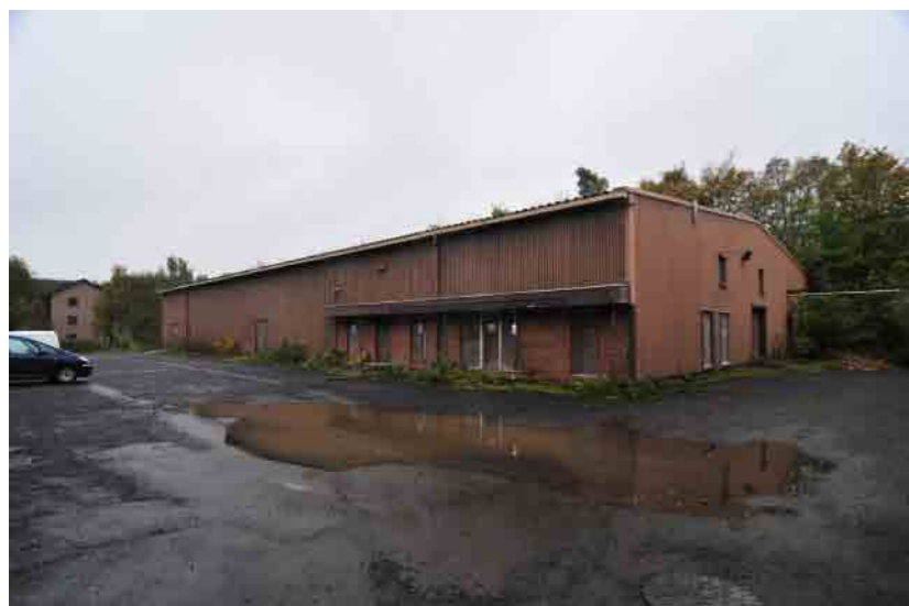
Plate 25 - Building 6, north and west-facing elevations of the South of Scotland Weavers factory building
