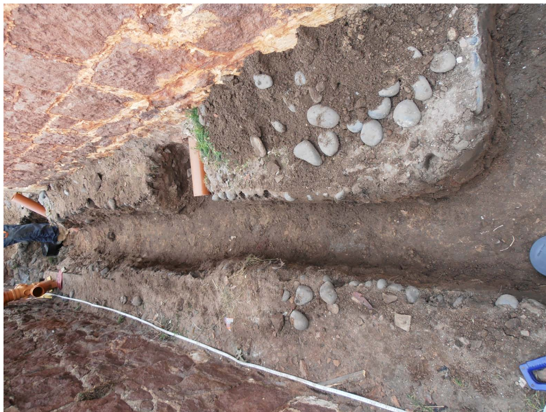
Figure 3 - General view of the service trench along the west side of the Coastguard Station
