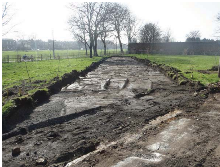
Fig. 4 - View over the demolished boundary wall with the topsoil removed from the cycleway within Leith Links
