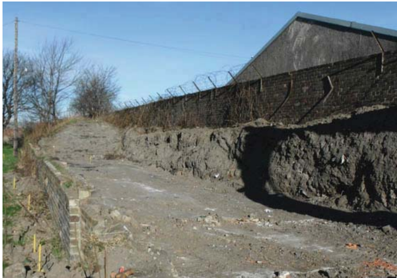
Fig. 2 - The boundary wall on the left with the section through the railway embankment on the right
