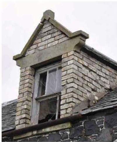
Fig. 18 - General view of one of the dormer windows prior to its removal
