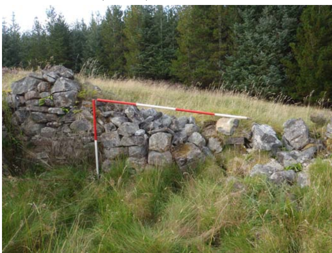
Fig.13 - Shot of blocked feature in south-facing elevation of former north gable of Room 6 (Site 1a)
