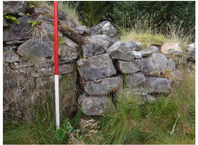
Fig.16 - Shot of running joint and blocked feature in south-facing elevation of north gable (Site 1a)
