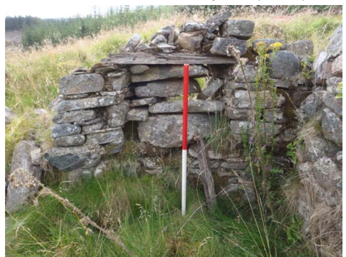
Fig.14 - Blocked feature, probably a window, with wood lintel; west wall Room 6 (Site 1a)
