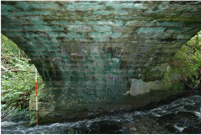
Plate 7: South abutment, north-facing ashlar stonework below the bridge and soffit stonework above
