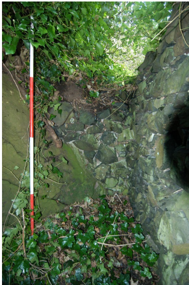
Plate 27: Infilling wall between the main interior elevation and natural rock (east side)
