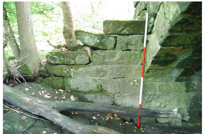
Plate 12: North abutment, west side showing tree root impact
