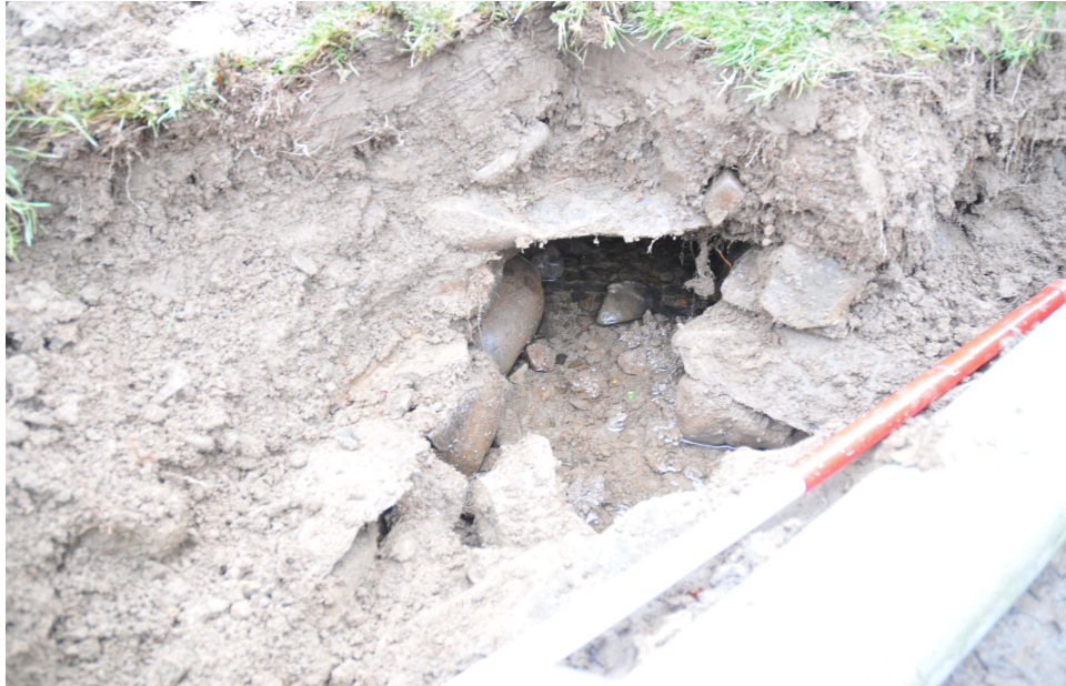
Plate 32: Gas pipe on the north side of Abbotsford House showing in-situ box-drain
