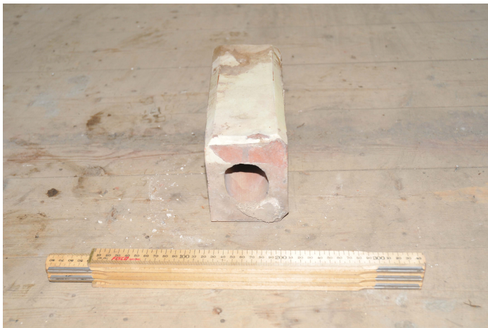
Plate 20: Room G.14 showing a cross-section of a fire-proof brick taken from the cupboard
