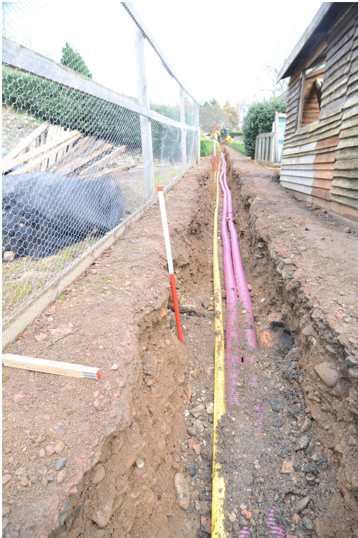
Plate 33: Gas pipe trench through the gardeners' path, general shot showing the route
