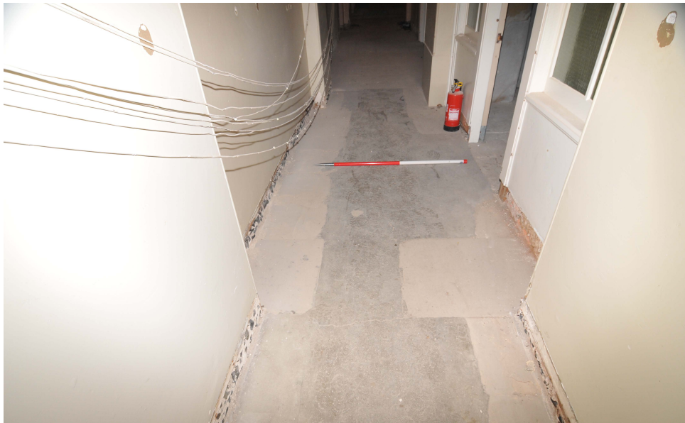
Plate 1: Basement corridor in area B.48 showing flagstones in situ prior to removal
