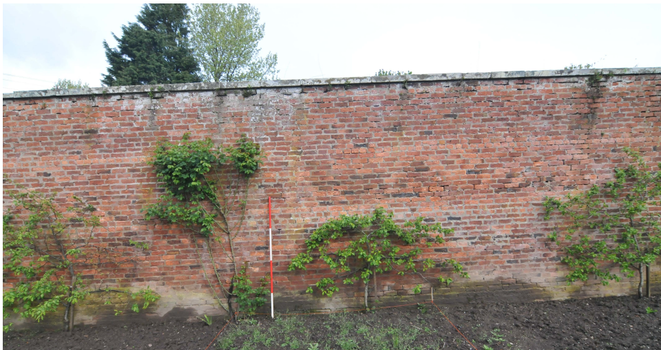
Plate 28: Kitchen garden wall showing poor condition of the brickwork
