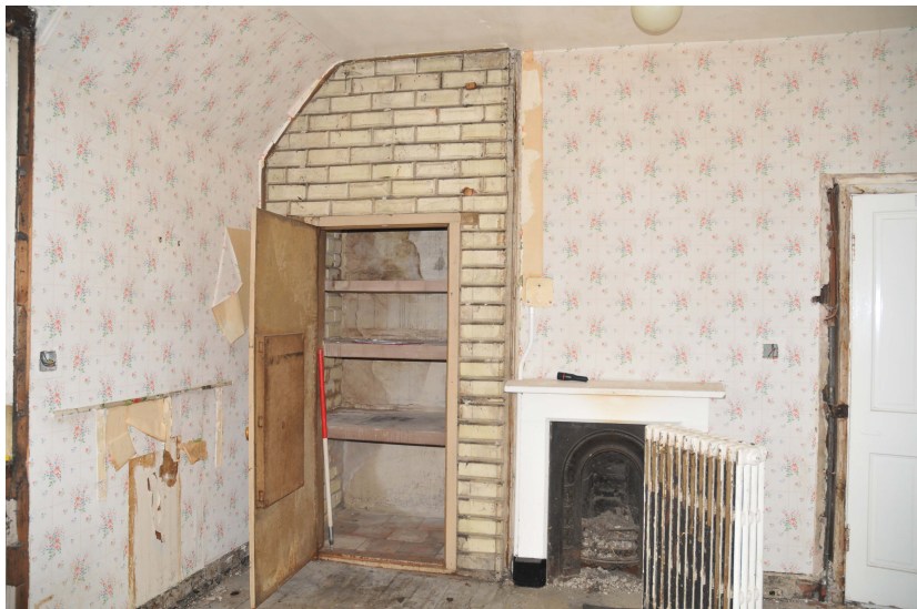
Plate 14: Room G.14 showing the fireproof cupboard in the corner of the room
