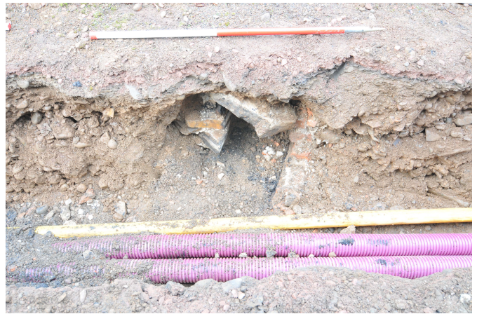
Plate 34: Gas pipe trench through the gardeners' path, general shot of the hypocaust flue
