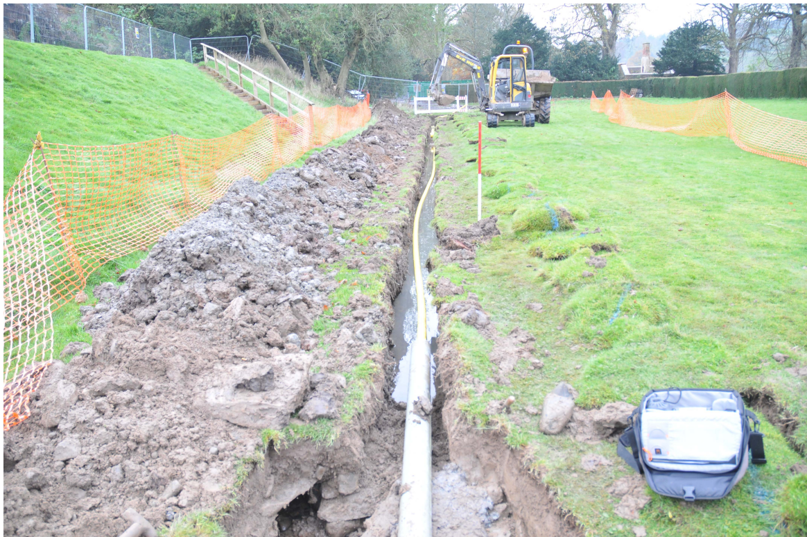
Plate 31: Gas pipe trench on the north side of Abbotsford House, general view looking east
