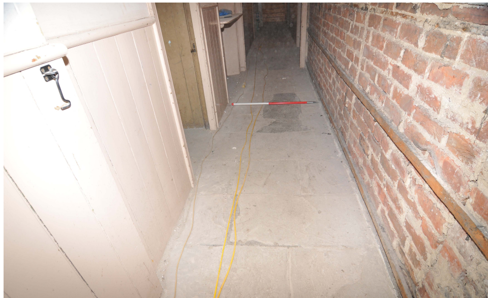
Plate 2: Basement corridor in area B.17 showing flagstones in situ prior to removal
